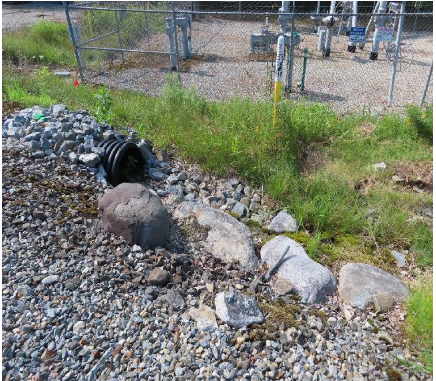
Photo 9. View (looking west) of existing stormwater culvert and swale that will be extended to facilitate stormwater discharges beyond the areas of planned ground disturbance.
