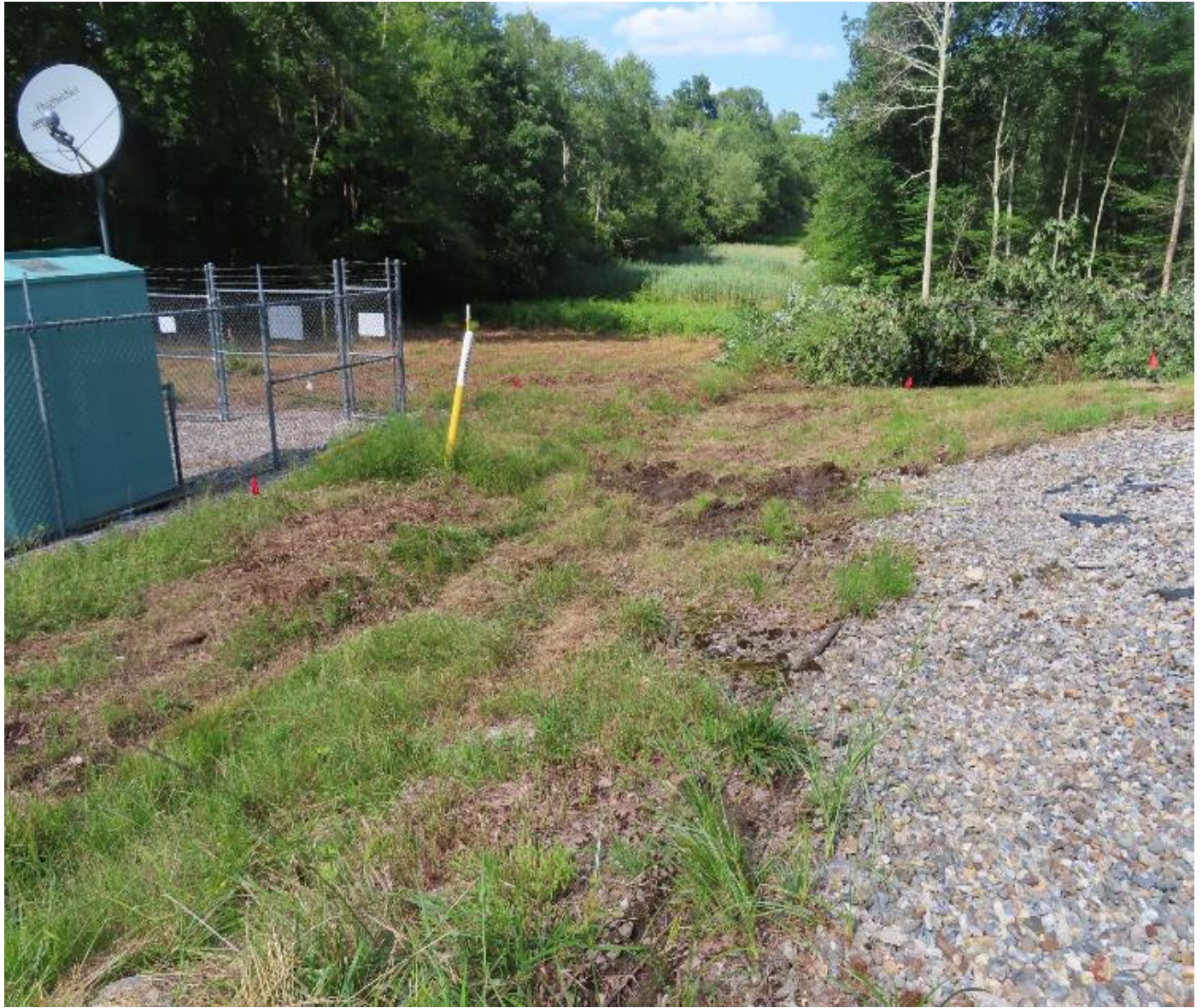
Photo 10. View (looking northeast) along area where culvert and swale will be extended.
