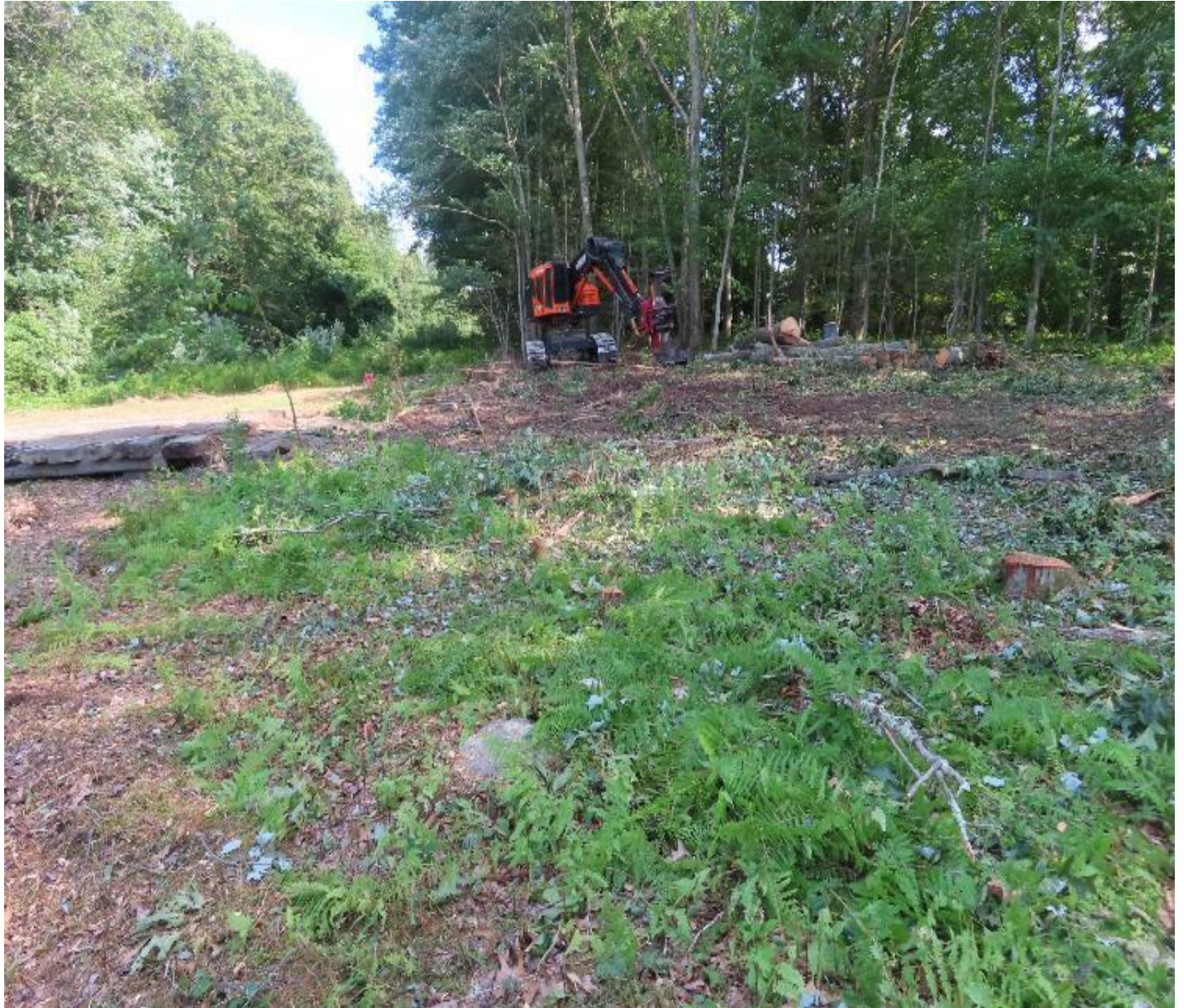
Photo 5. View (looking southeast) of trees being cleared from workspace along edge of the E-System easement. Stumps and rootlets will not be removed in areas that are being used as temporary workspace.
