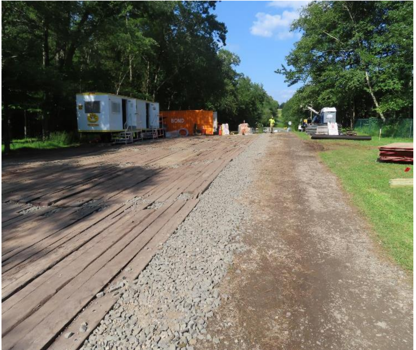
Photo 3. View (looking northeast) of matted staging area with office trailer and other staged equipment/materials.
