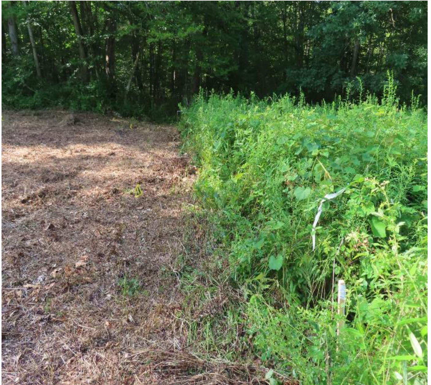
Photo 7. View (looking northwest) of workspace limits along mainline easement where vegetative buffer needs to remain intact upslope of wetland (W-CZ-01)
