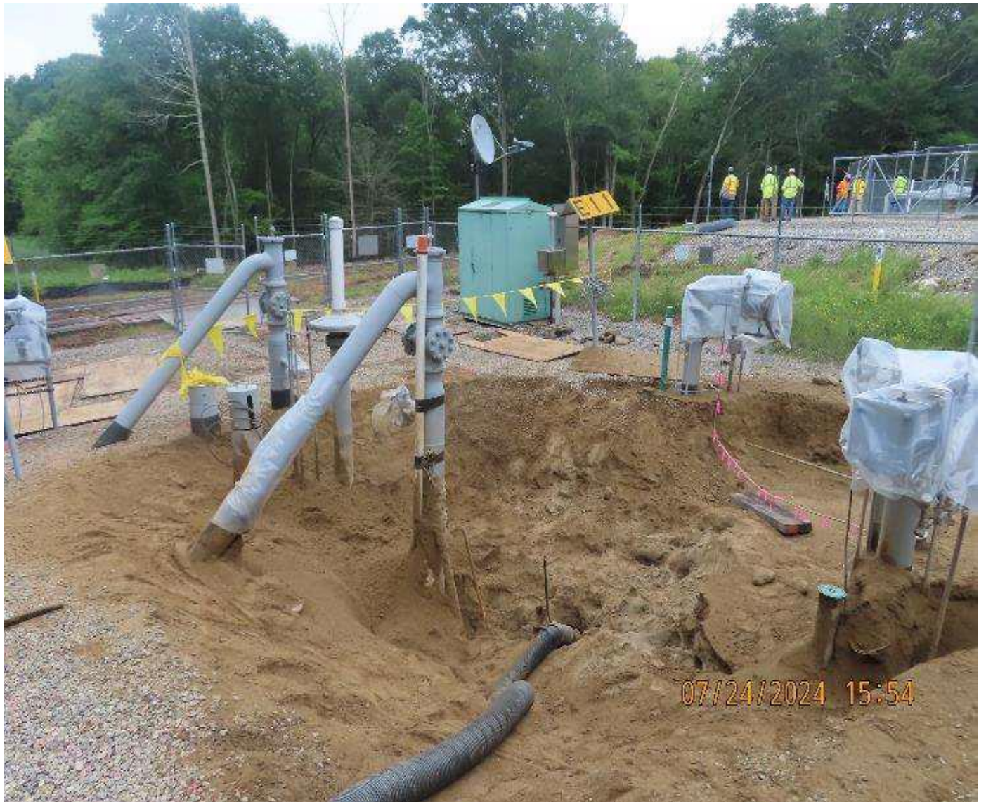
Photo 8. View (looking east) of buried pipe exposure work in the 30-inch valve pen area.
