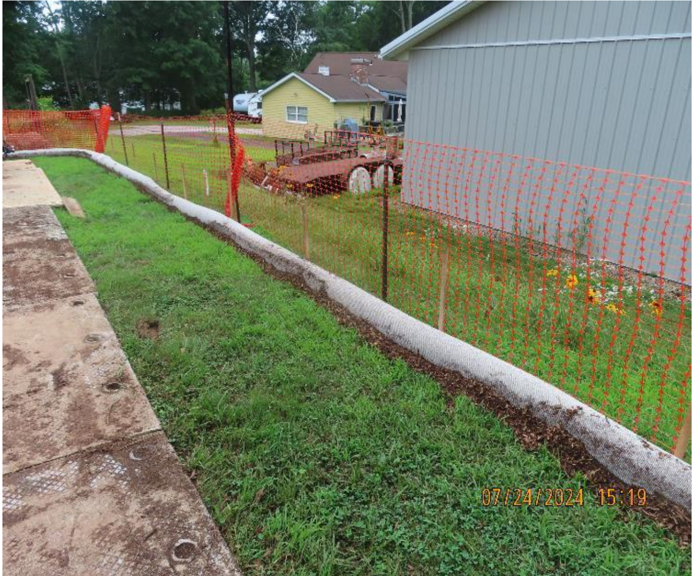
Photo 3. View (looking southwest) of filter sock and security fencing installed along both sides of the access road.
