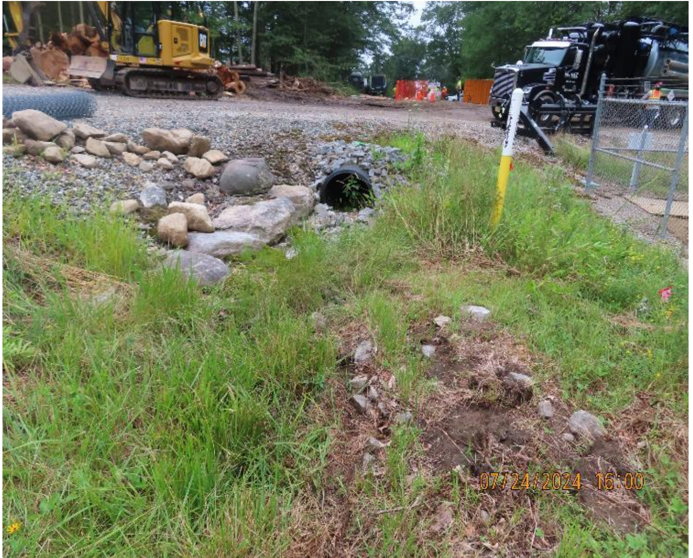
Photo 8. View (looking southeast) of drainage culvert and swale by valve pen. The culvert will be extended as ground disturbance approaches this area, which is upslope of current excavation work.
