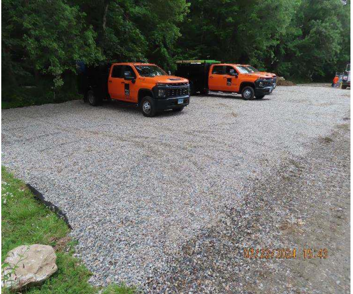
Photo 2. View (looking northeast) of stone placed over geotextile fabric to establish area for welding and fabrication.
