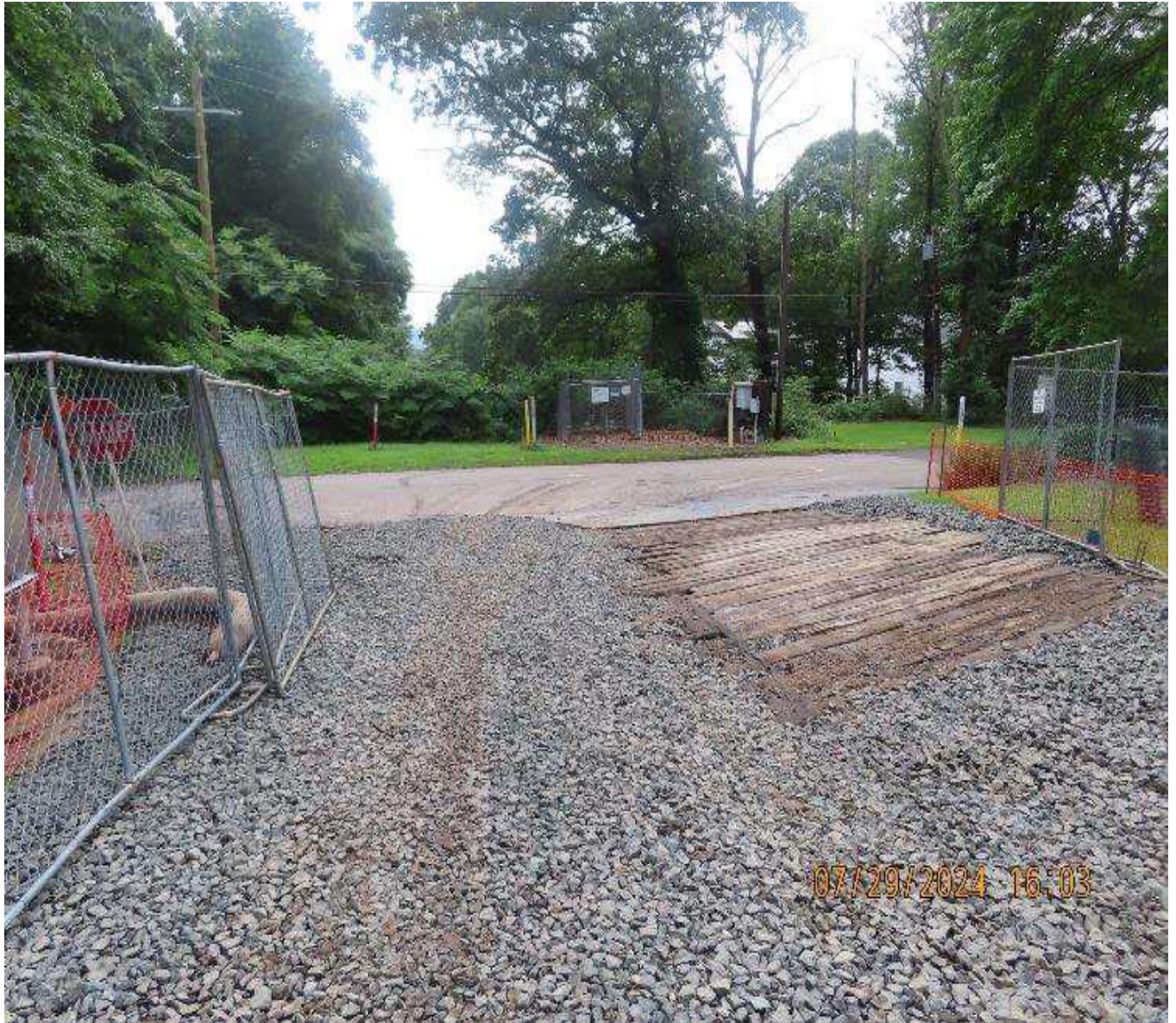
Photo 9. View (looking southwest) of site entrance shortly after a rain event. Road is swept at a minimum of once per day.
