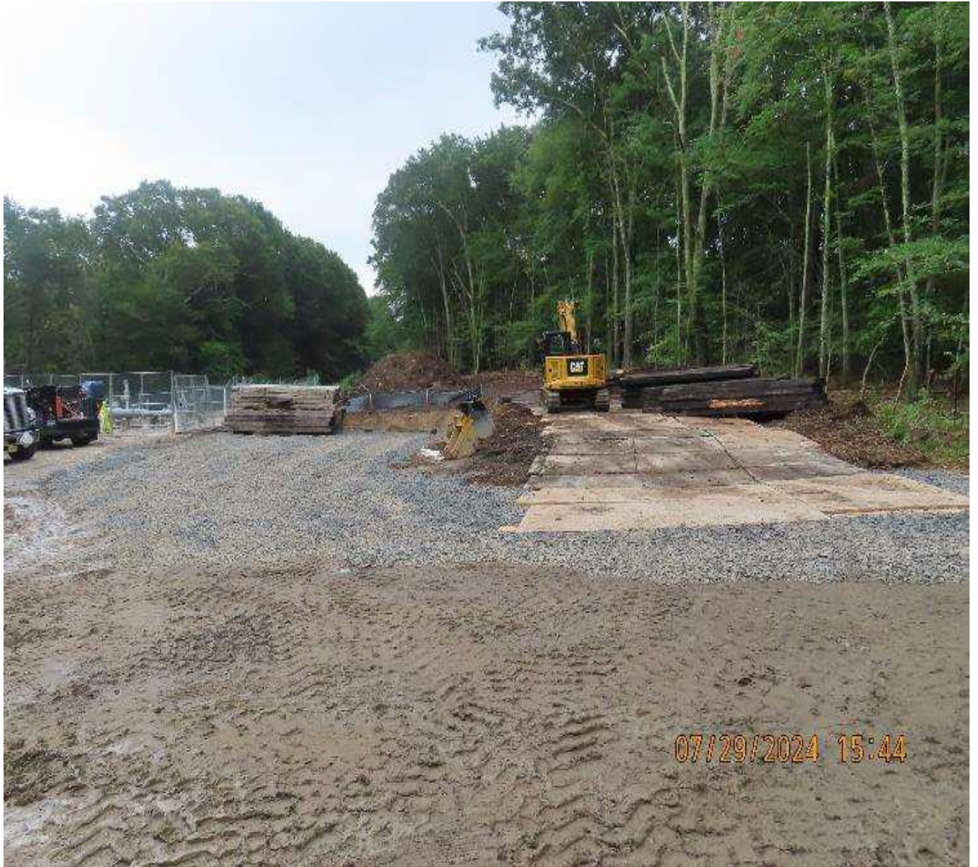
Photo 2. View (looking southeast) of mat travel lane around southwest side of launcher yard for access to E-1 system tie-in area.
