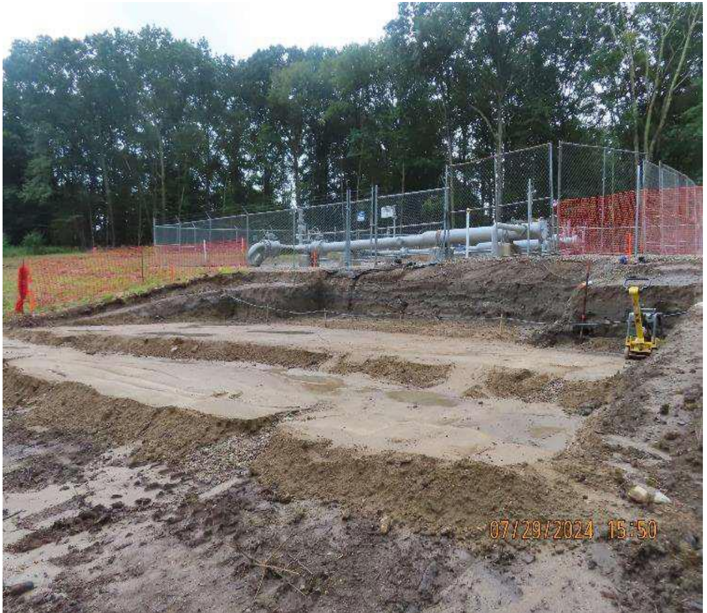
Photo 5. View (looking south) of excavation, fill, and grading area completed for the new regulator skid. Addition of stone fill and compaction is pending to set the prefabricated concrete foundation.
