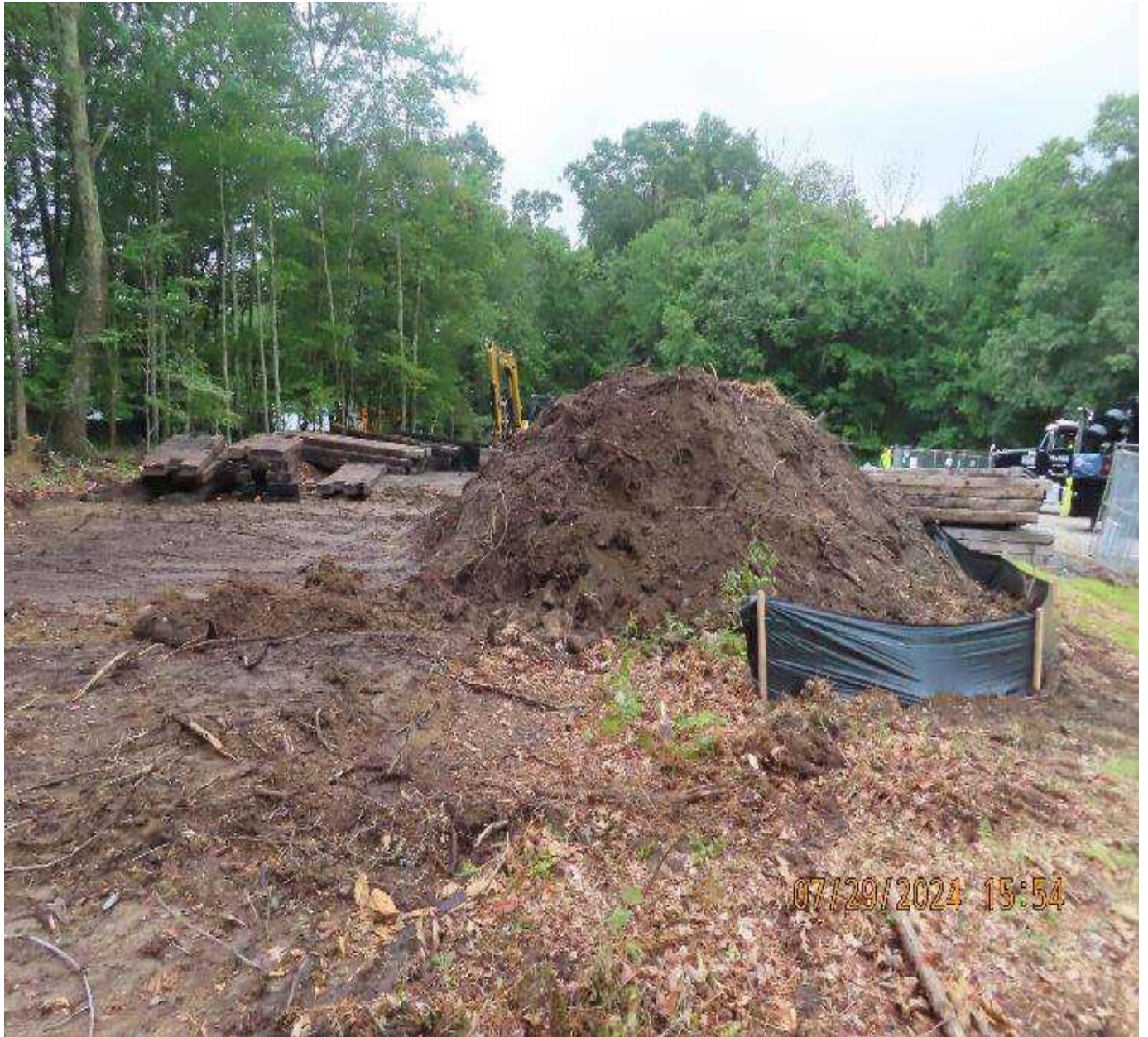
Photo 3. View (looking northwest) of topsoil stockpile with site fence bounding the downslope side.
