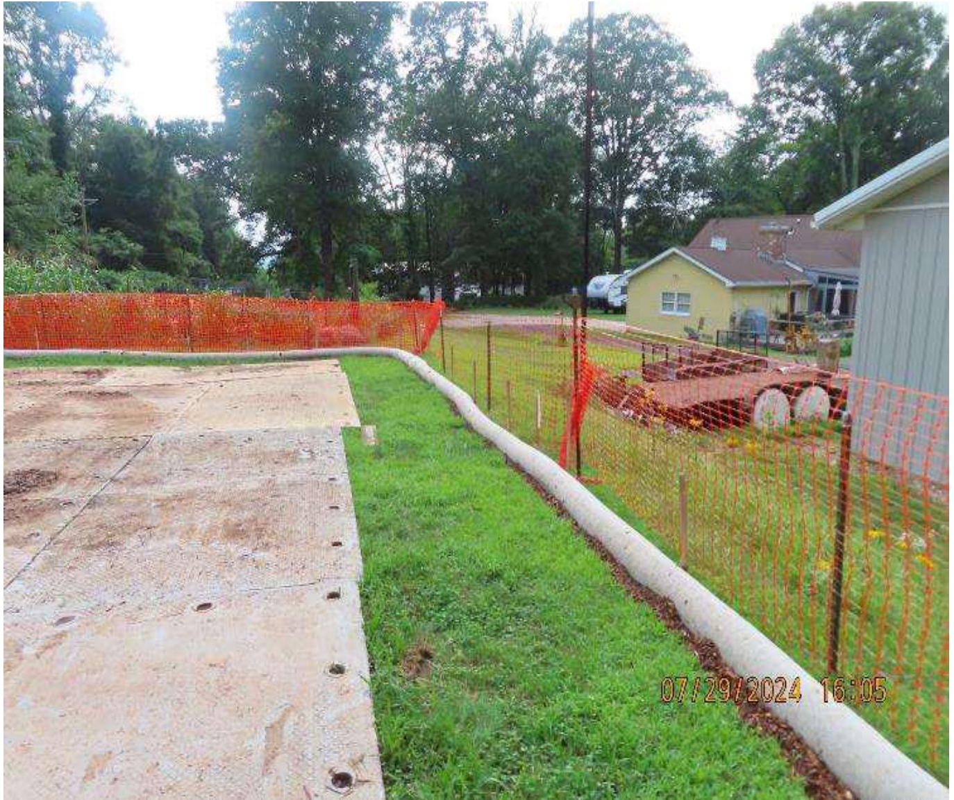
Photo 8. View (looking southwest) of compost filter sock and security fencing along north side of site access.
