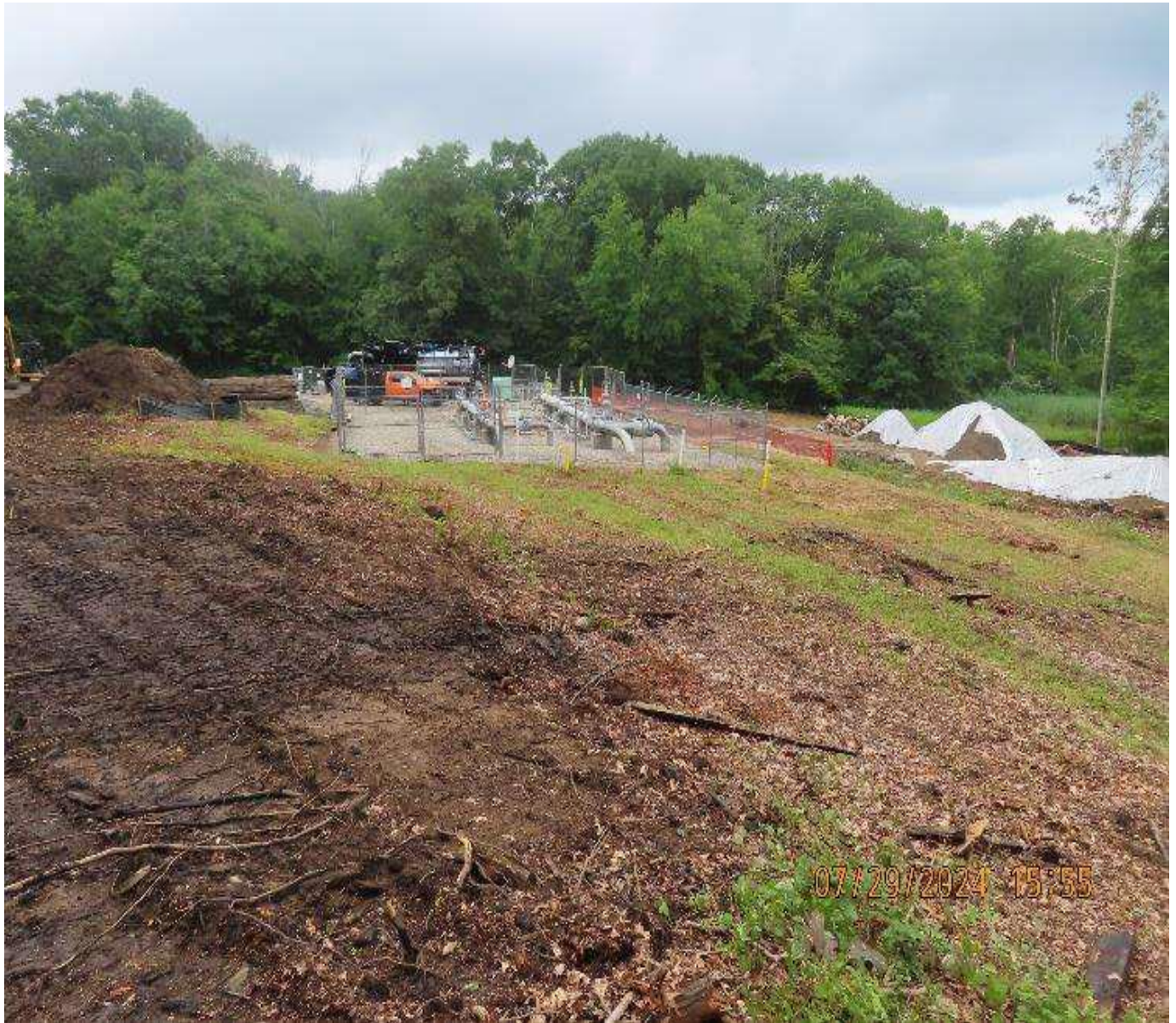
Photo 4. View (looking northwest) of workspace around the 30-inch valve pen area with excavation occurring within the fenced pen area.
