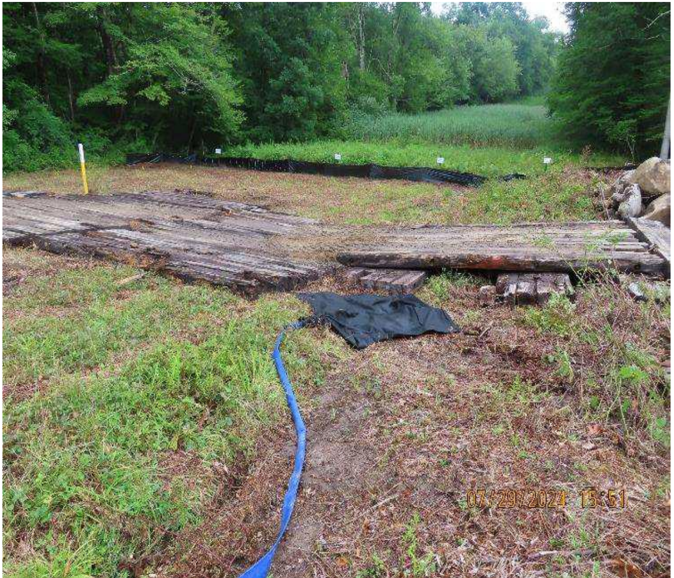
Photo 6. View (looking north) of filter bag used to manage excavation dewatering discharges
