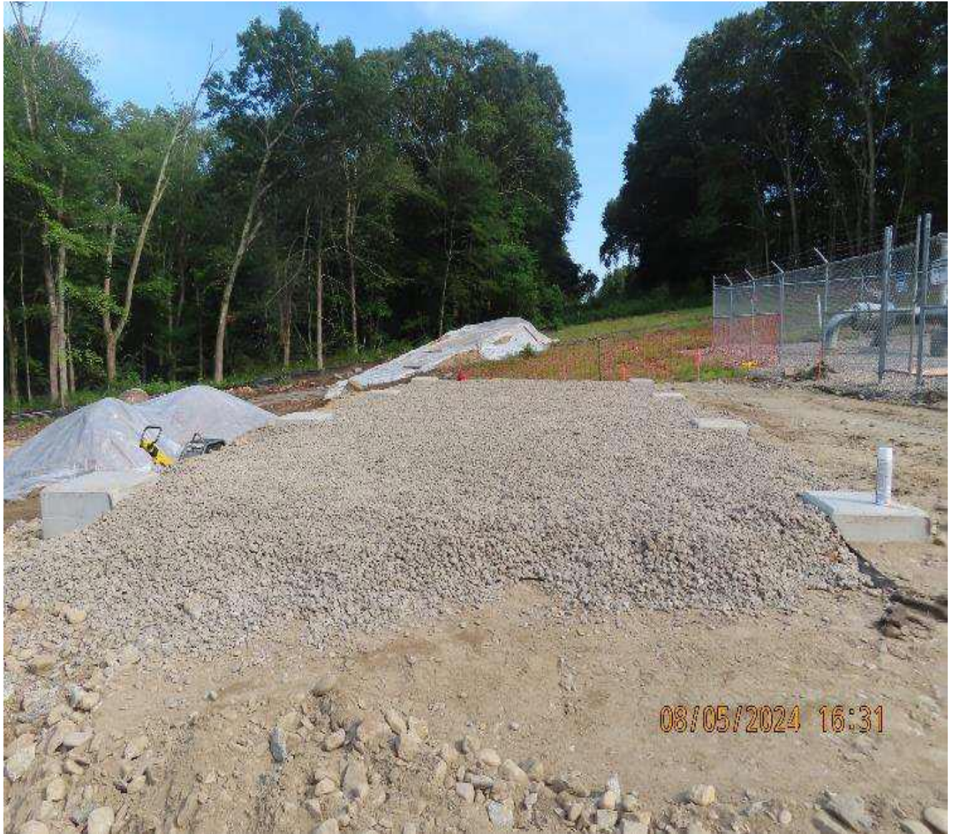
Photo 9: View (looking southeast) of precast foundations and gravel fill placed for new regulation skid.
