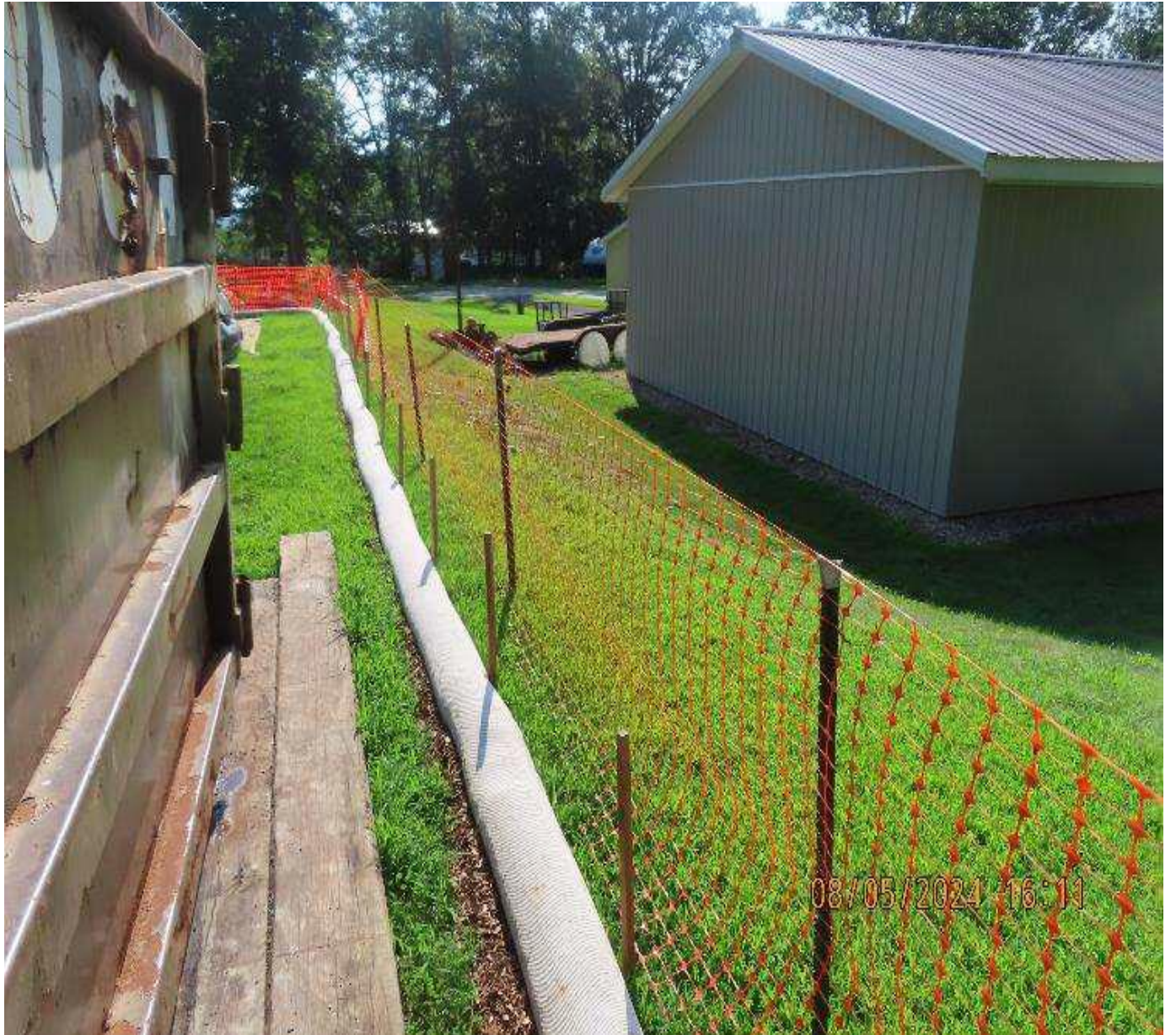
Photo 3: View (looking southwest) of temporary security fence and perimeter erosion controls near residence.
