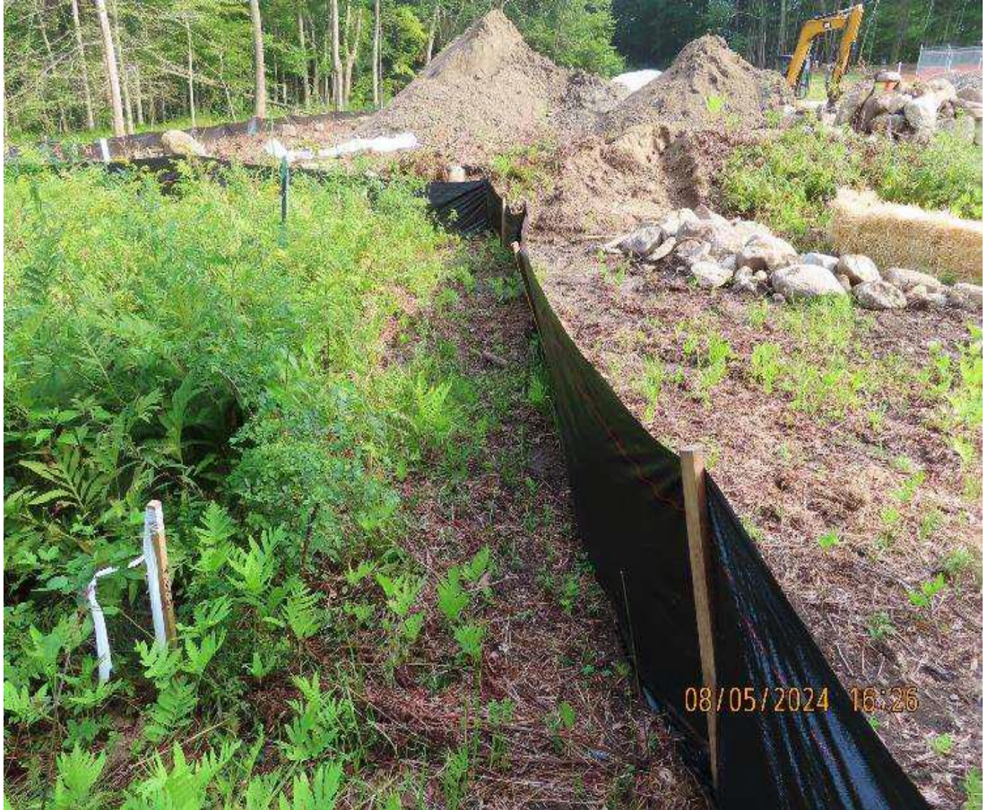
Photo 7: View (looking southeast) of perimeter silt fence in soil stockpile area.
