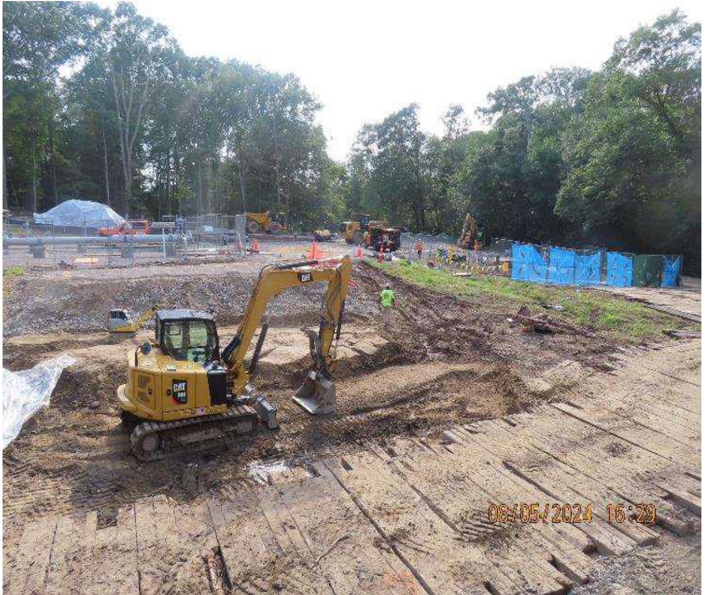
Photo 8: View (looking southwest) of earthwork occurring with launcher yard (upper left) and 30-inch valve yard (upper right) in the background.
