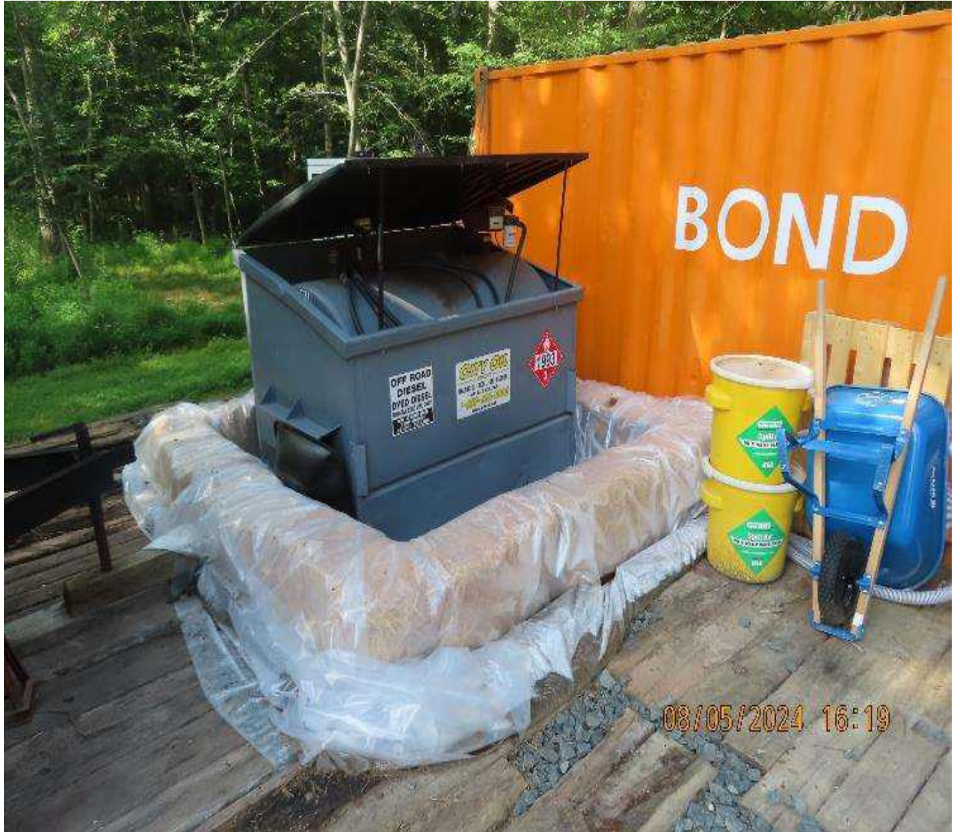
Photo 4: View (looking north) of designated refueling tanks with secondary containment.
