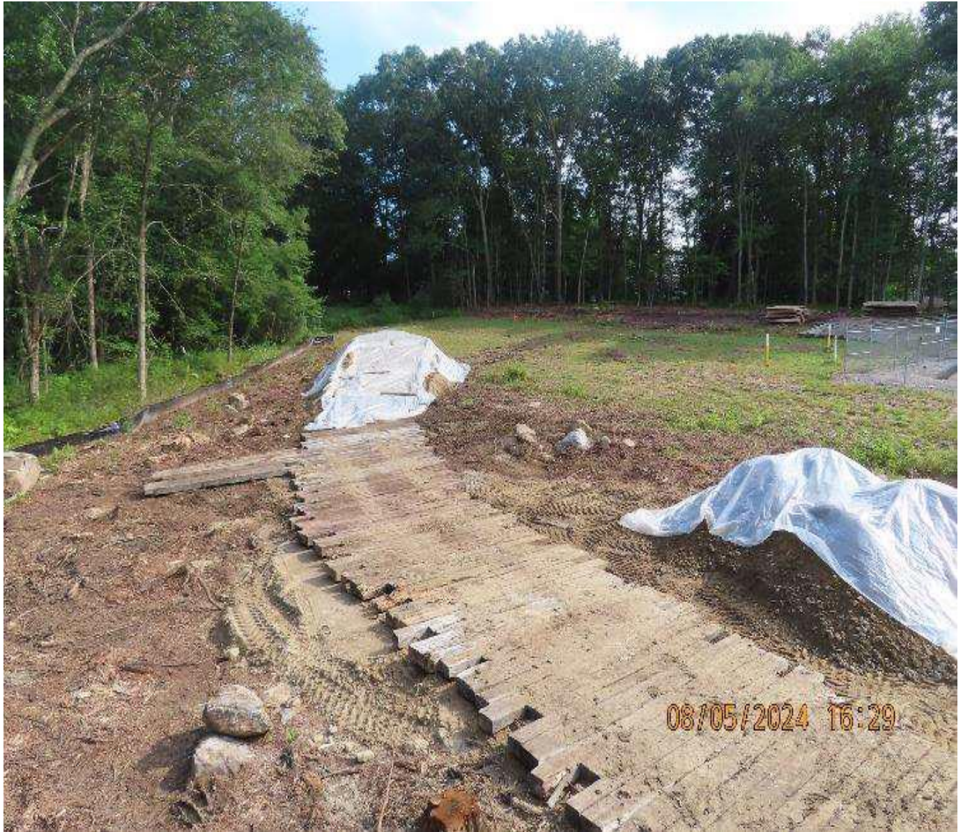
Photo 10: View (looking southeast along E-1 System right-of-way) of temporary mat road around launcher yard.
