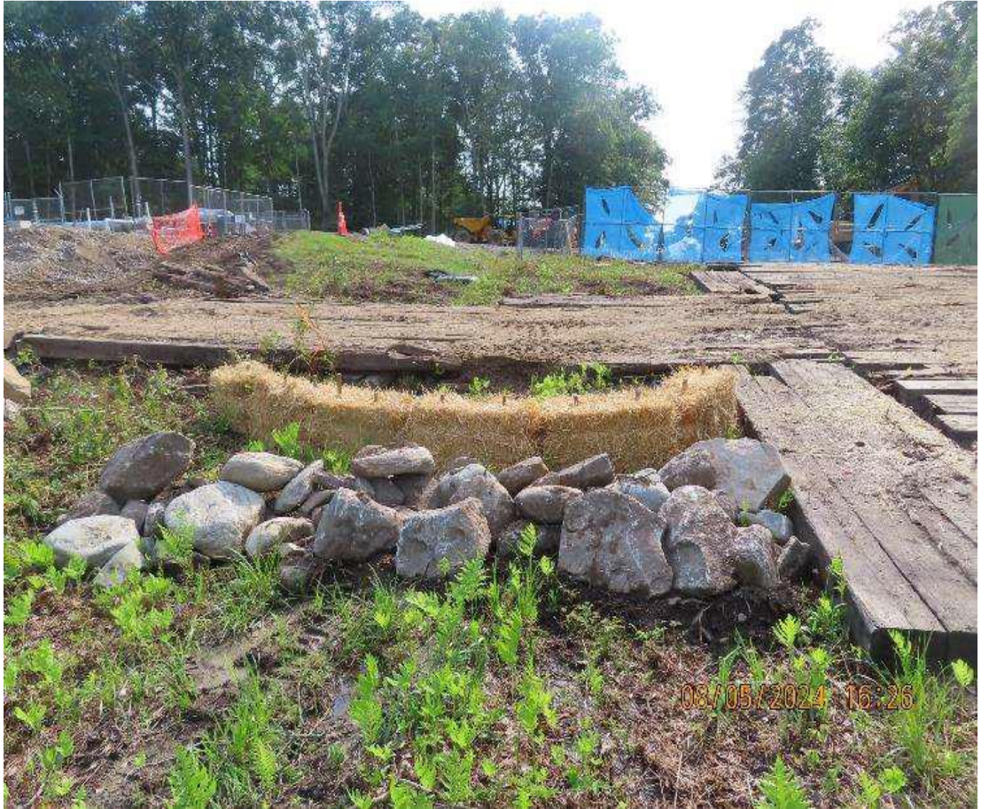
Photo 6: View (looking southwest) of straw bale and rock check dam placed downslope of dewatering discharge.
