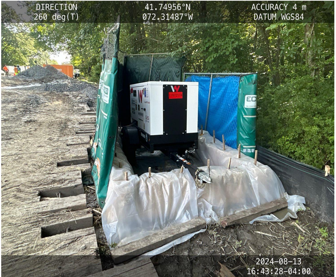
Photo 3: View (looking west) of recently mobilized generator with secondary containment and sound barriers.
