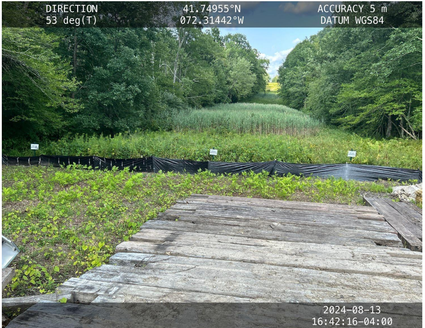
Photo 8: View (looking northeast) of silt fence and vegetation buffer separating workspace from wetland area.
