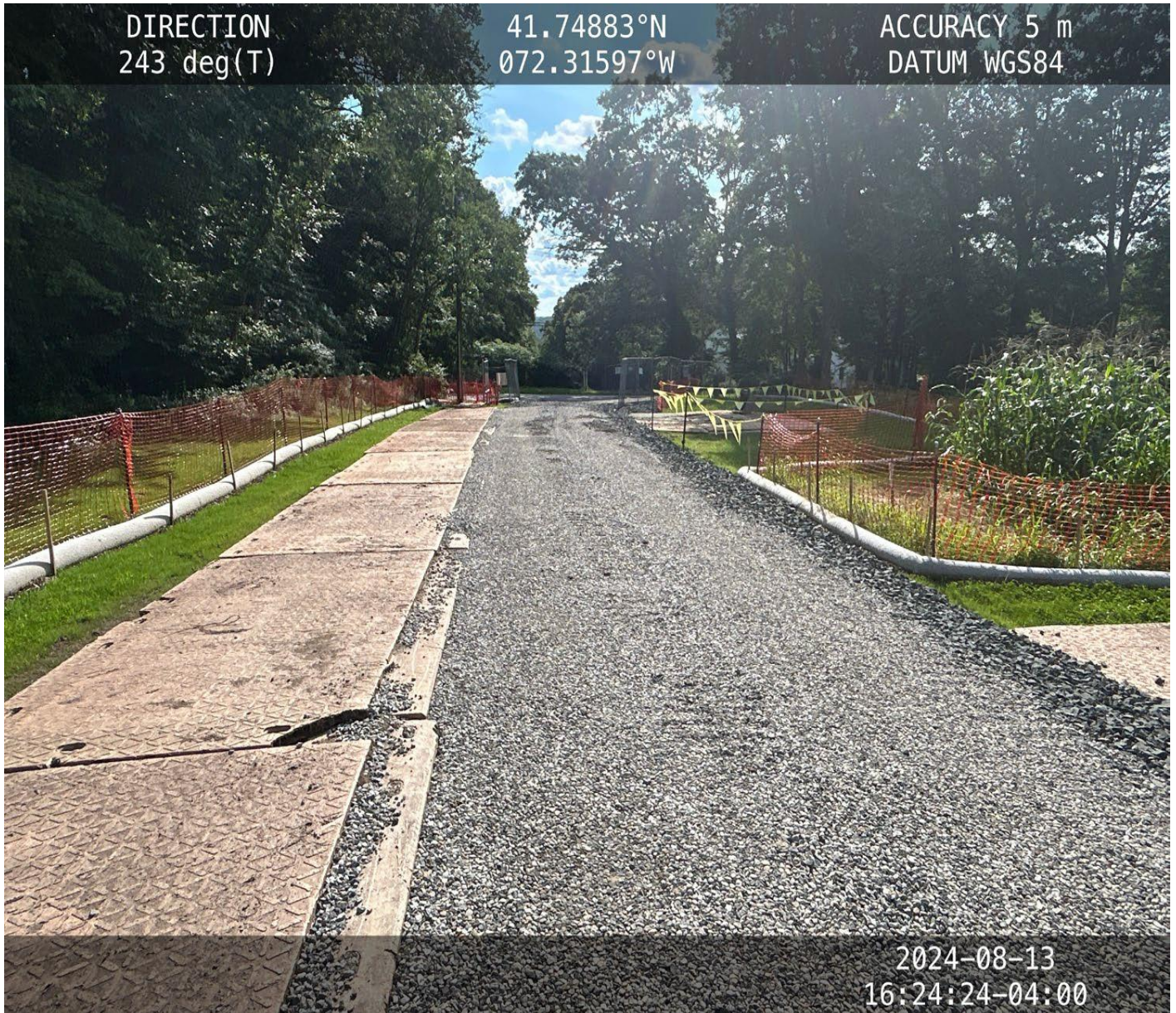
Photo 1: View (looking southwest) of access road, ECDs, and temporary fencing with mats placed to protect residential lawn.
