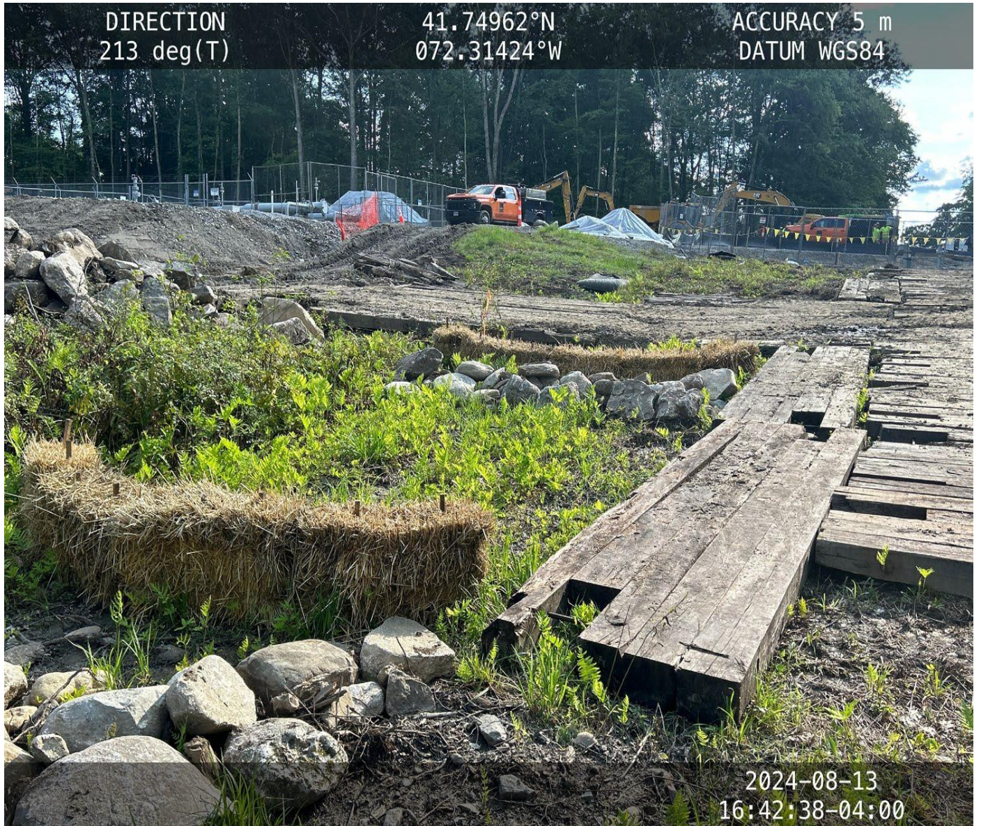
Photo 7: View (looking northeast) of filter bag for excavation dewatering discharges with check dams within drainage swale.
