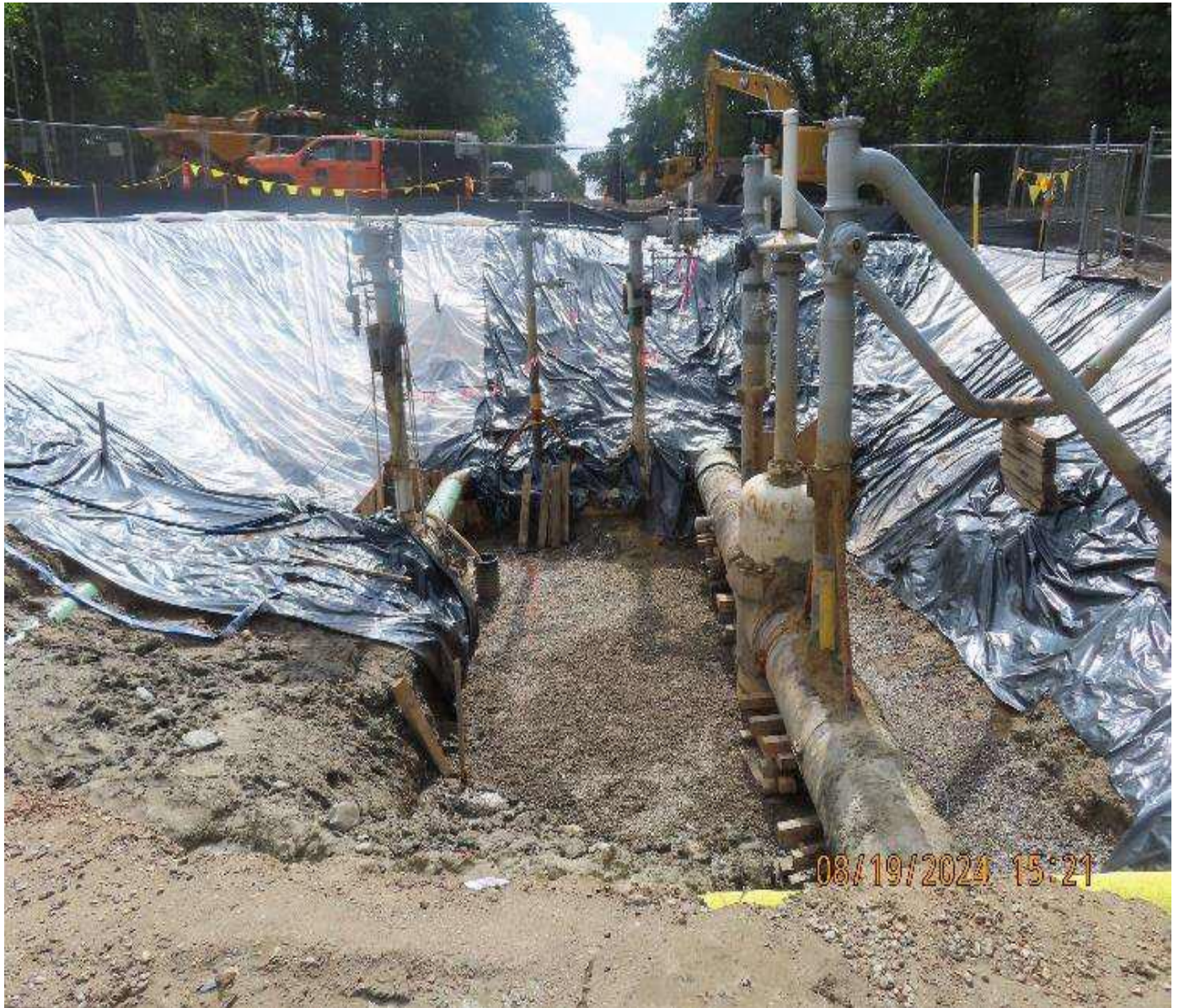
Photo 3: View (looking southwest) of valve yard excavation with side slopes lined with plastic sheeting for stability. Based is lined with clean stone.
