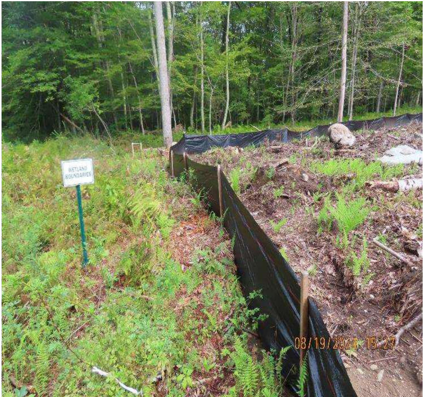
Photo 5: View (looking east) of silt fence protecting wetland W-CZ-01.
