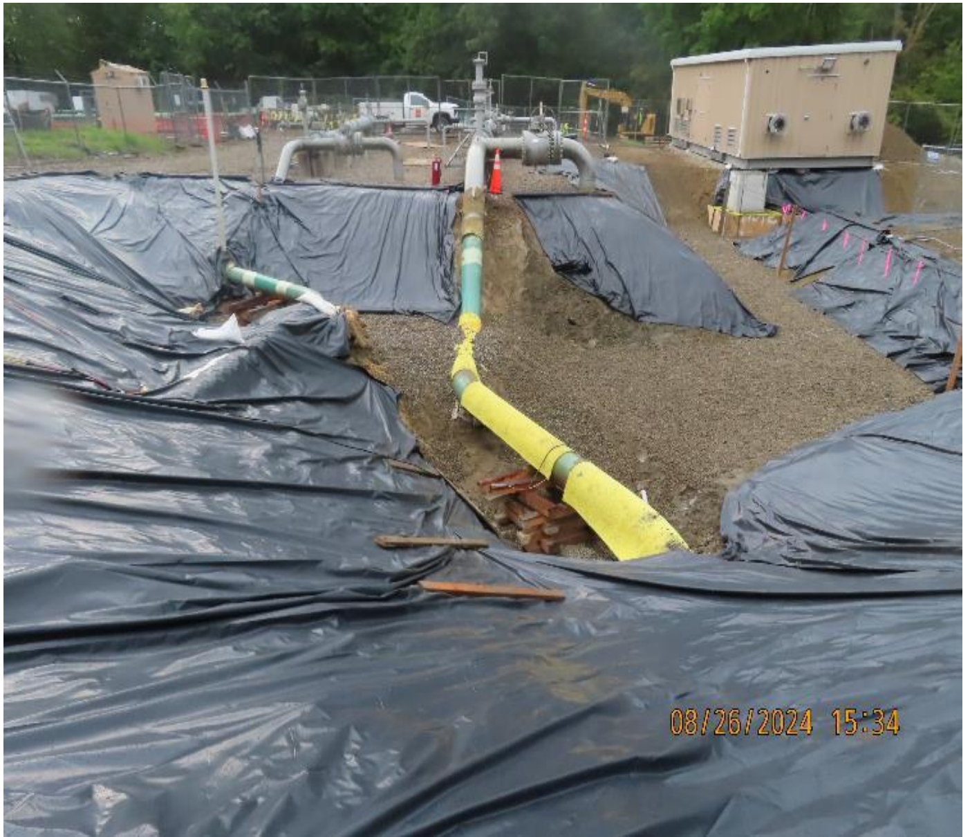
Photo 6: View (looking northwest) of stabilized excavation sidewalls for E-1 and E-1L work.
