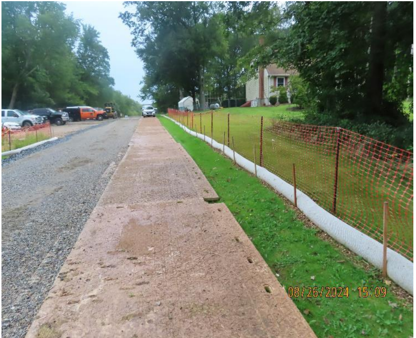
Photo 1: View (looking northeast) along access road with perimeter SESC and security fencing.
