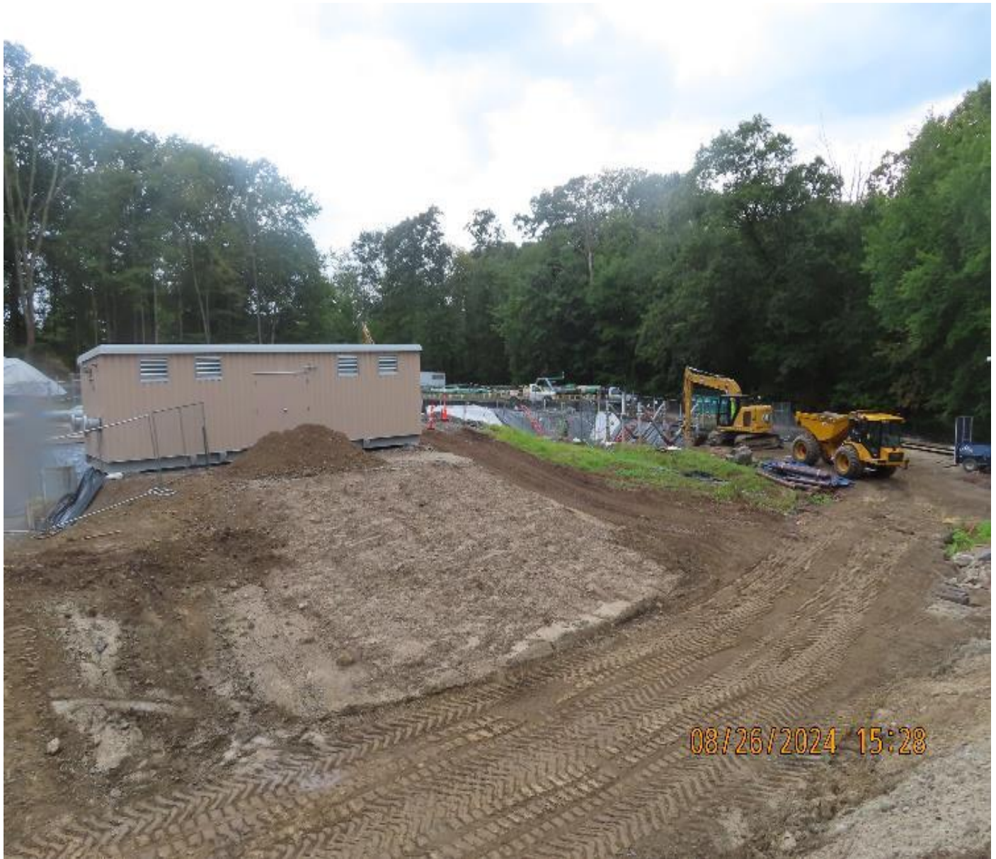
Photo 5: View (looking southwest) of new regular building after being set on foundations.
