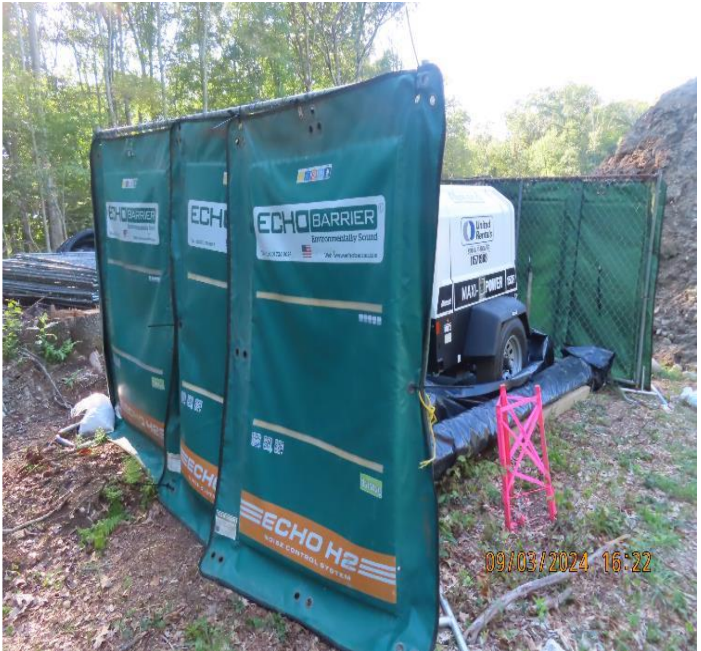
Photo 5: View (looking west) of portable generator with secondary containment and noise mitigation acoustic padding.
