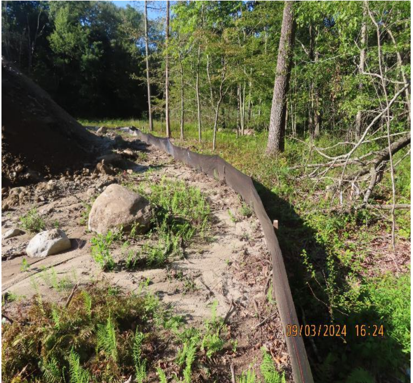
Photo 6: View (looking northwest) at silt fence in good condition after heavy rain event. Minor sediment accumulations with no migration beyond the silt fence was observed.
