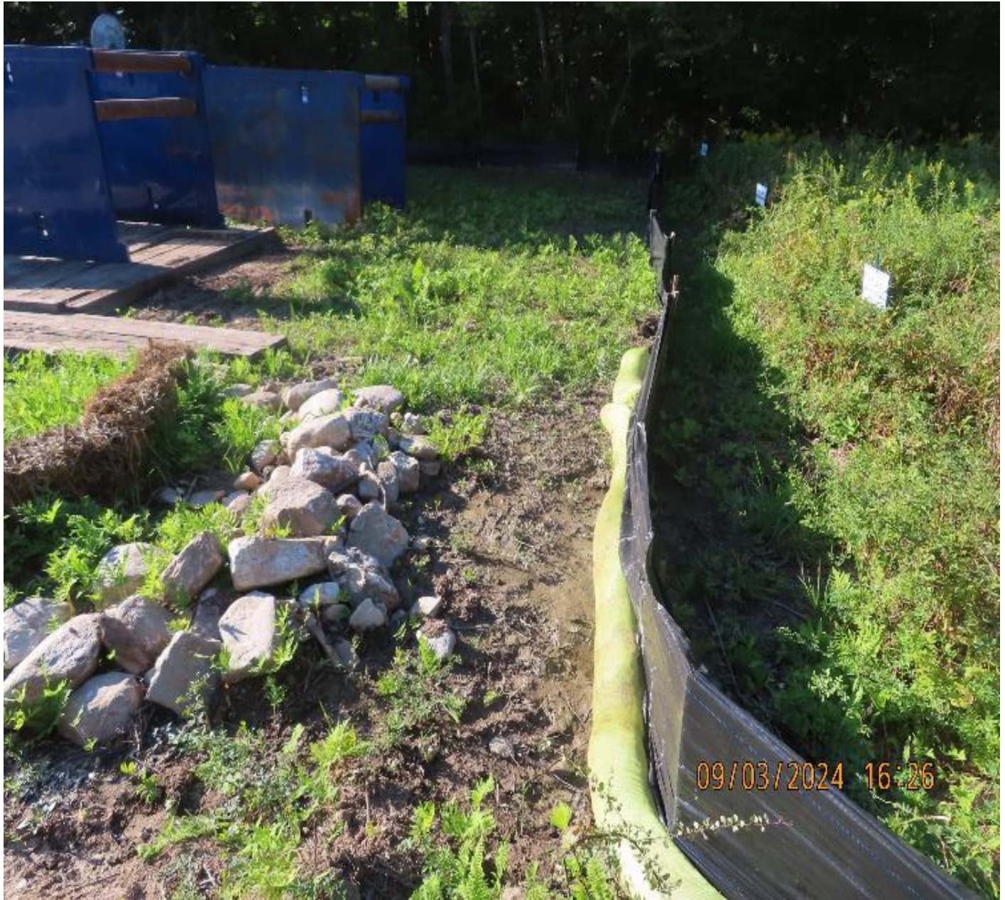
Photo 8: View (looking northwest) of silt fence protecting wetland W-CZ-01 in good condition after heavy rain event.
