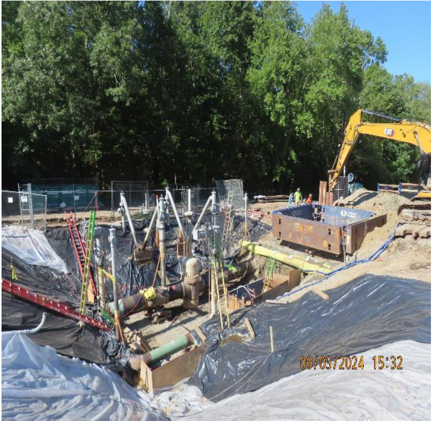
Photo 2: View (looking northwest) of excavation and sheet pile installation work taking place in the Valve Yard.
