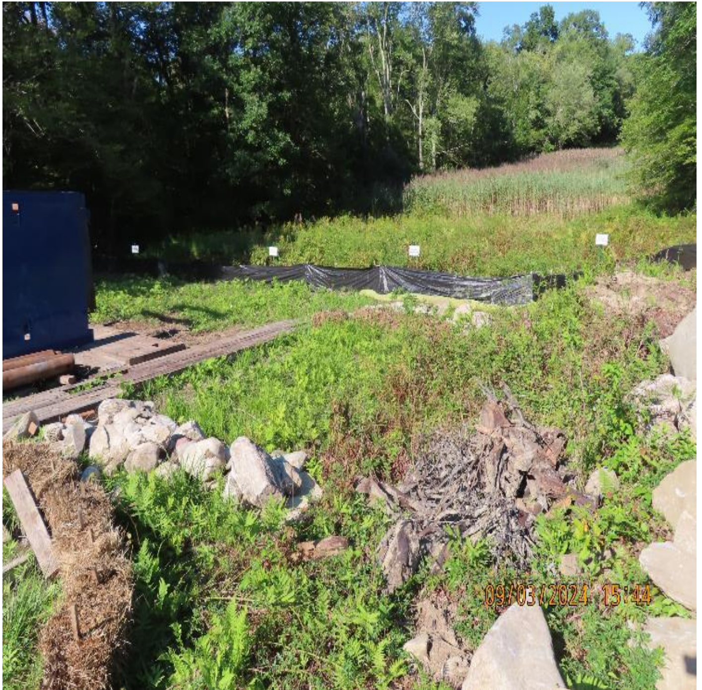
Photo 4: View (looking northeast) of excavation dewatering discharge flow path with rock check-dams.
