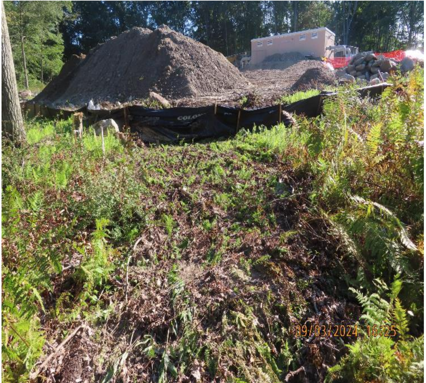
Photo 7: View (looking south) of flattened vegetation from stormwater flow that occurred during recent heavy rain event. Minor damage to silt fencing was repaired.
