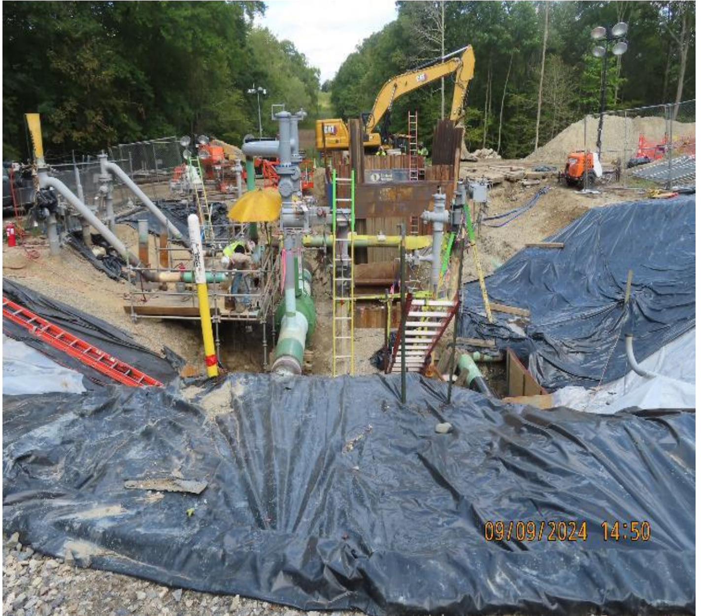
Photo 3: View (looking northeast) of ongoing excavation and mechanical work in valve yard.
