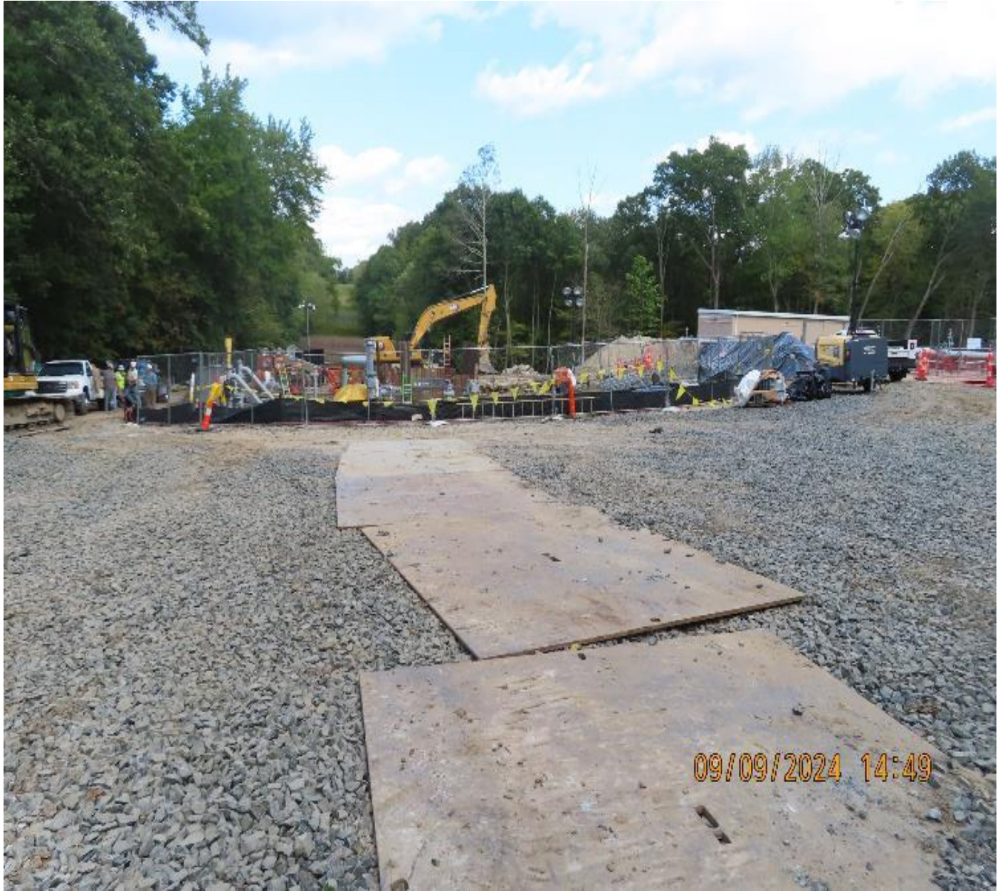
Photo 4: View (looking northeast) of area stabilized with rock and metal sheeting for lift crane setup.
