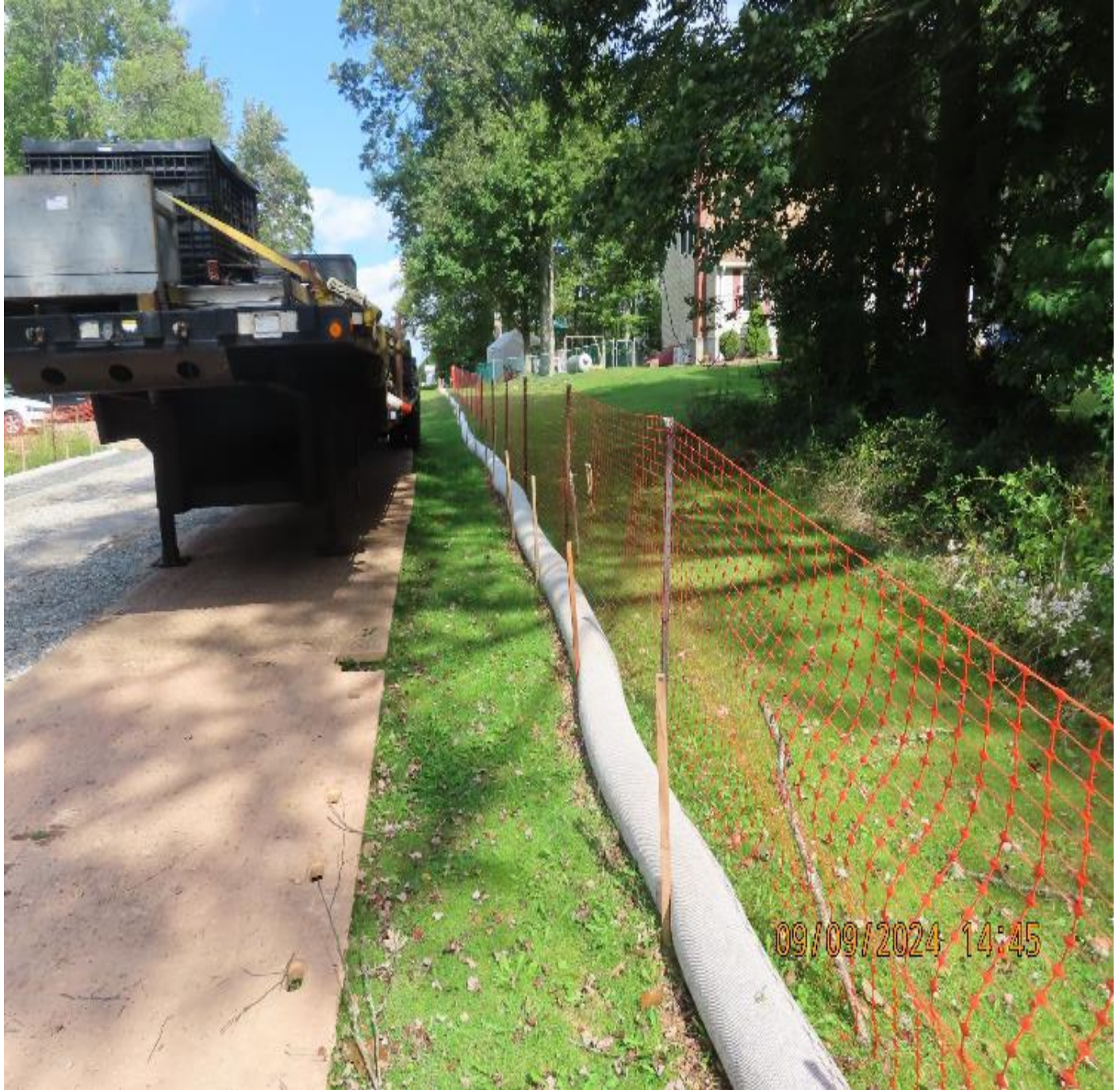
Photo 2: View (looking northeast) of compost filter sock and security fencing along workspace boundary in residential area.
