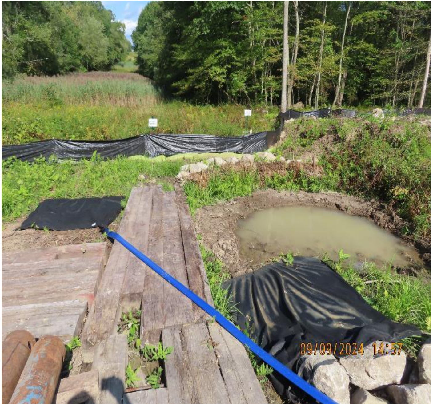
Photo 6: View (looking northeast) of filter bag for excavation dewatering discharges with shallow sump pit excavated nearby to increase retention for ground infiltration.
