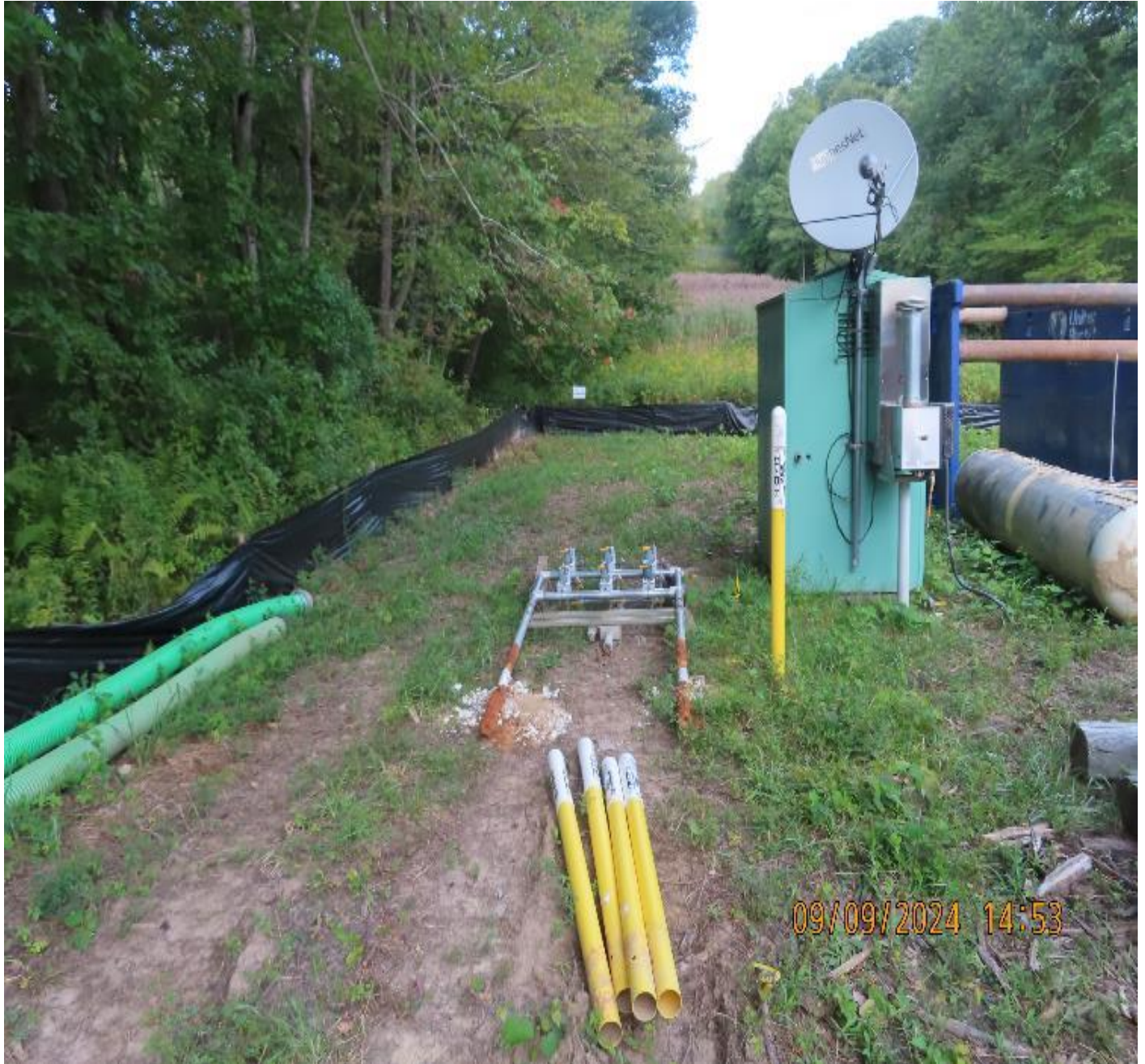
Photo 5: View (looking northeast) of new satellite dish near northwest corner of worksite.
