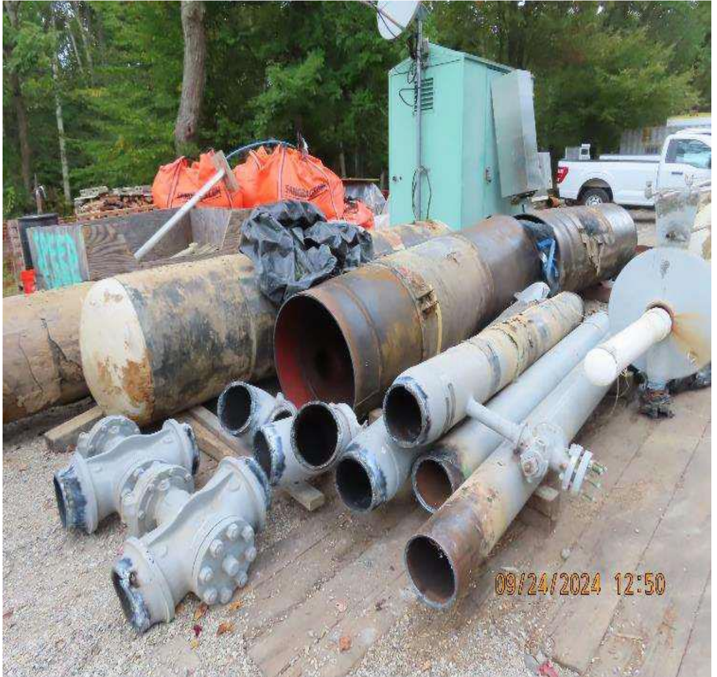
Photo 8: View (looking north) of retired valves and piping placed in staging area pending off-site transport and disposal. Open ends will be secured with plastic sheeting or
