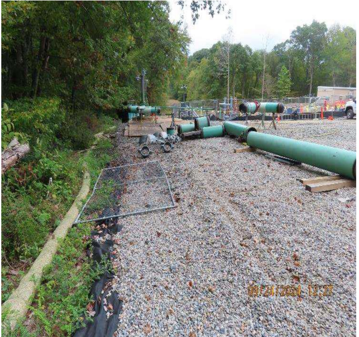
Photo 2: View (looking northeast) of ECDs along boundary of pipe and valve fabrication area.
