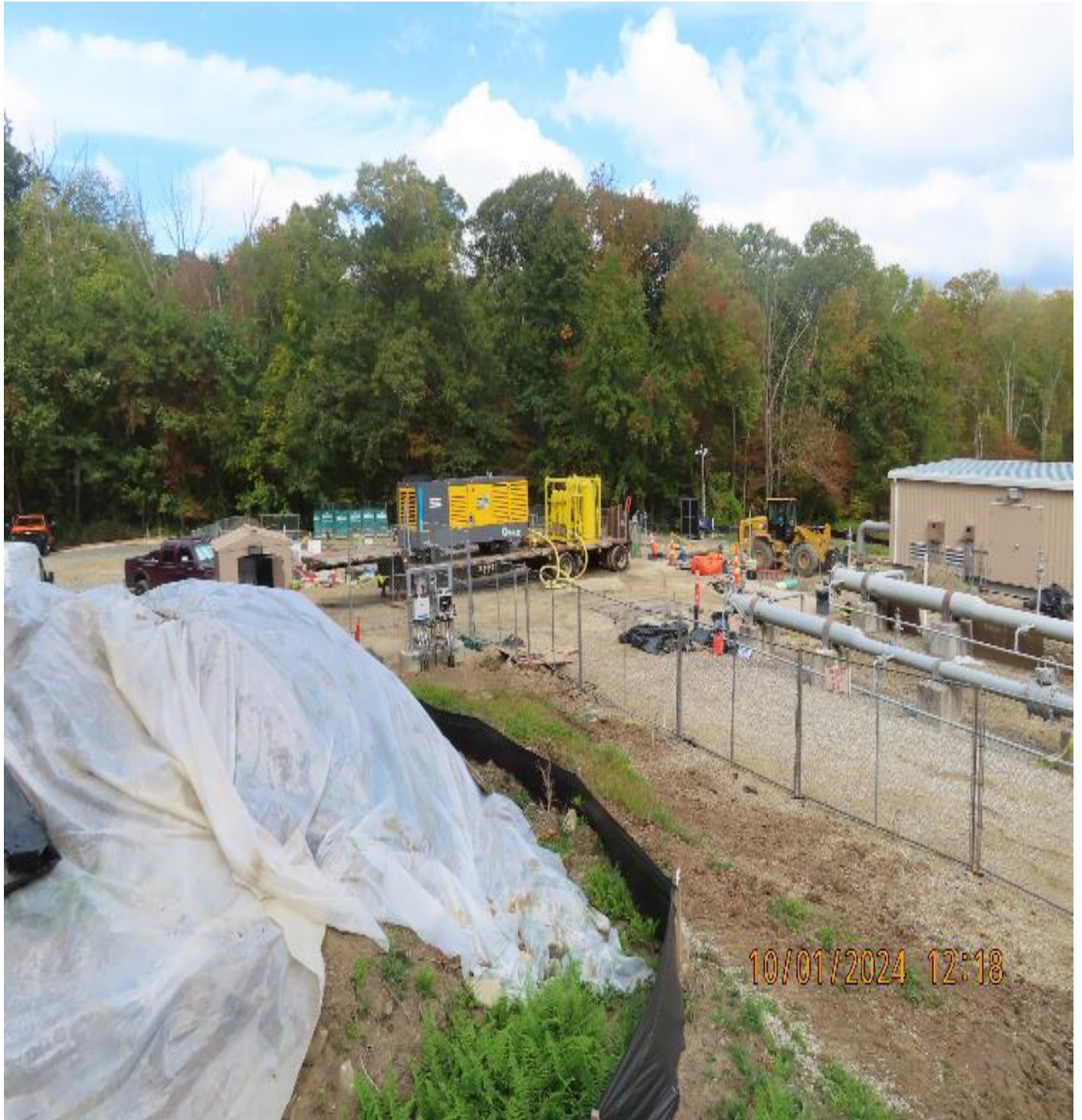
Photo 6: View (looking northwest) at segregated stockpile of topsoil with covering and perimeter erosion controls.
