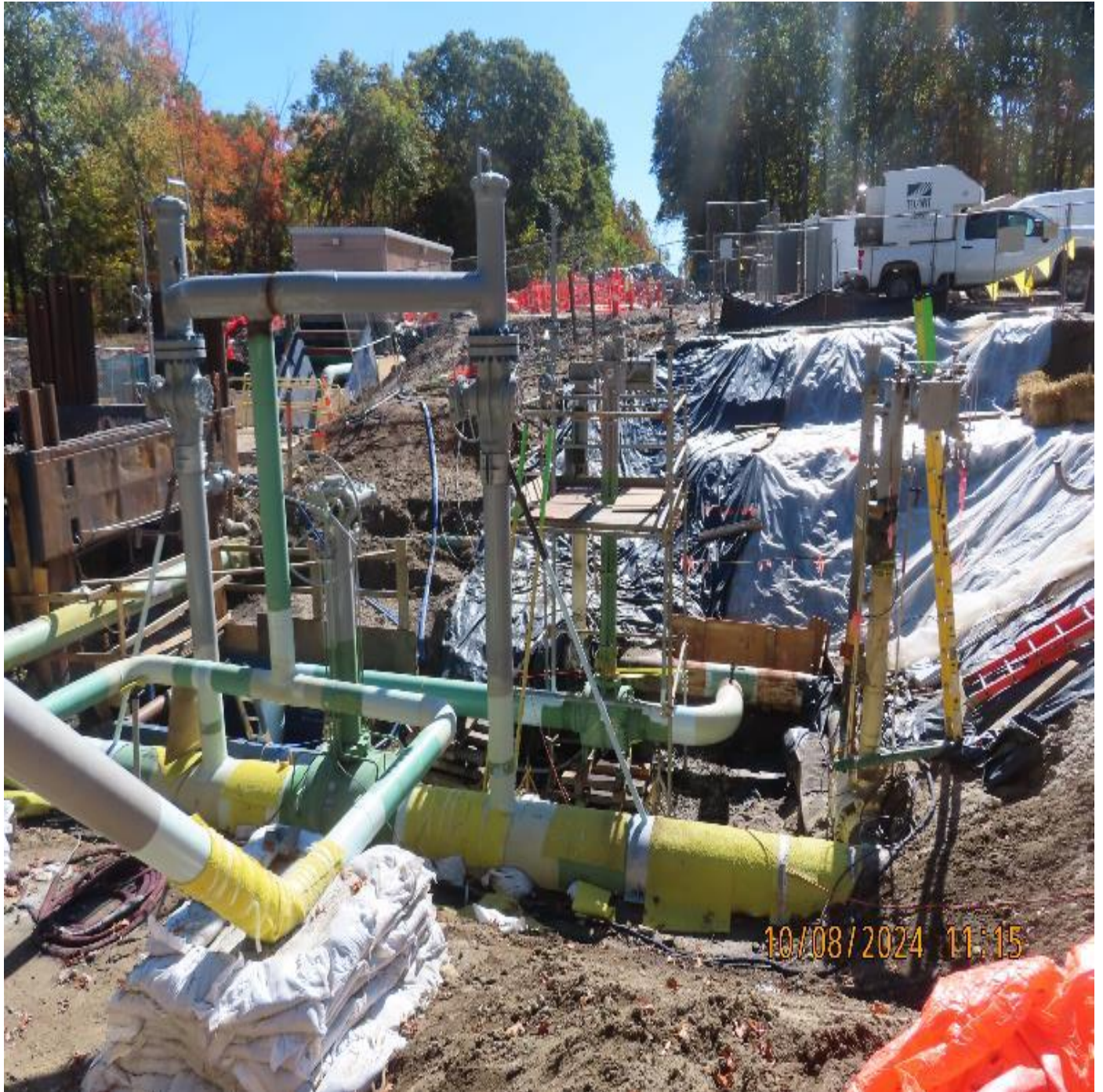
Photo 2: View (looking southeast) of conditions in the valve yard, where tie-in to the 16-inch line is scheduled for next week.
