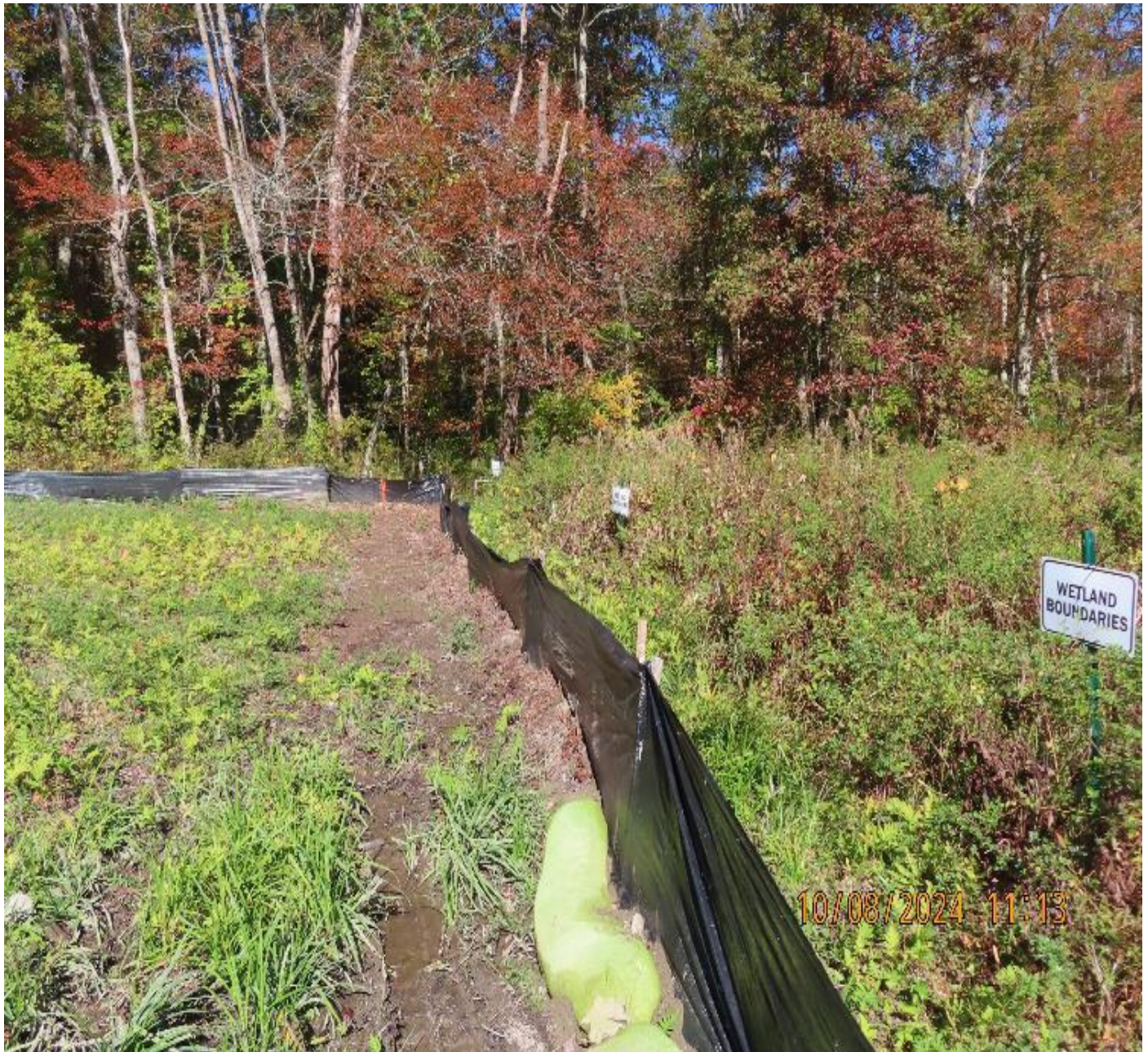
Photo 6: View (looking northwest) of silt fence around low area in northwest corner of site.
