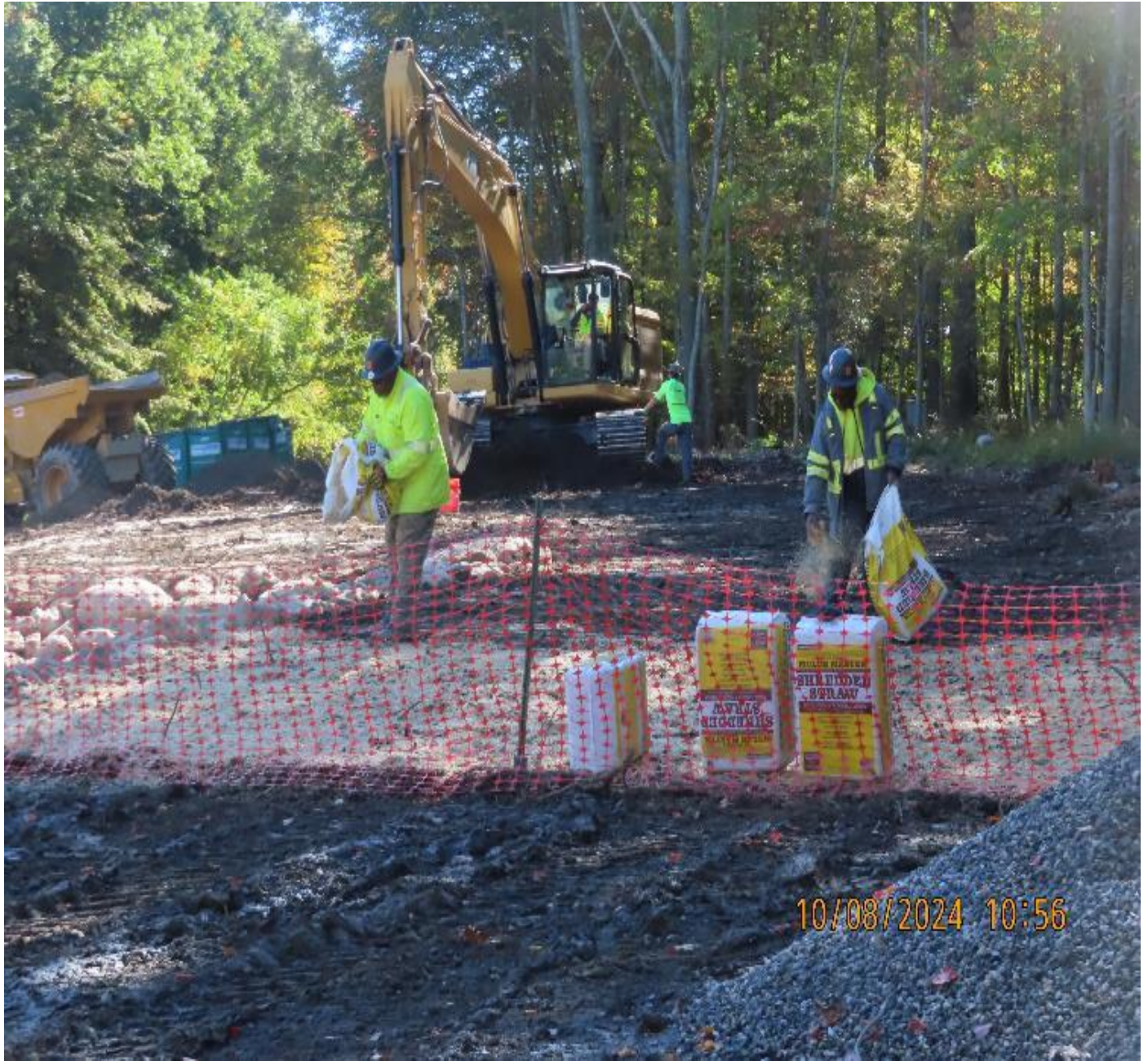
Photo 8: View (looking southeast) along southern portion of site where final grading, topsoil replacement, and seed application work was conducted.
