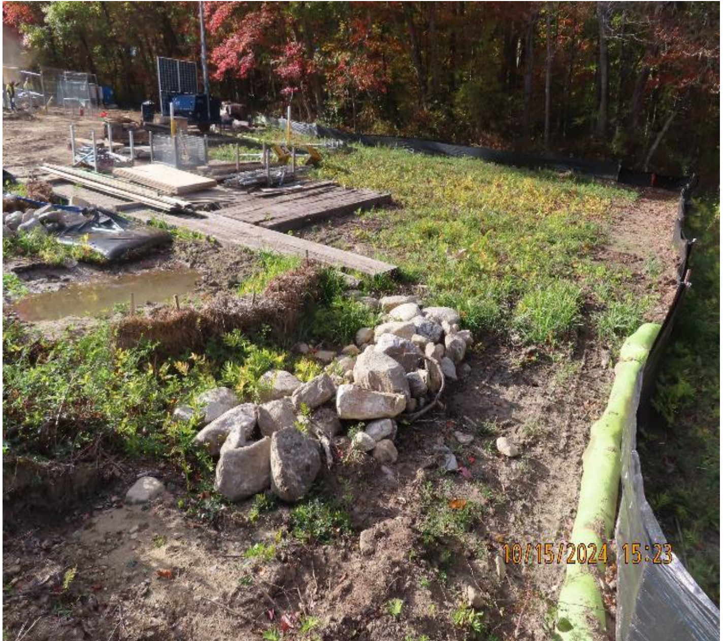
Photo 4: View (looking northwest) of excavation dewatering controls and down-gradient perimeter controls at northwest corner of site, near wetland W-CZ-01.
