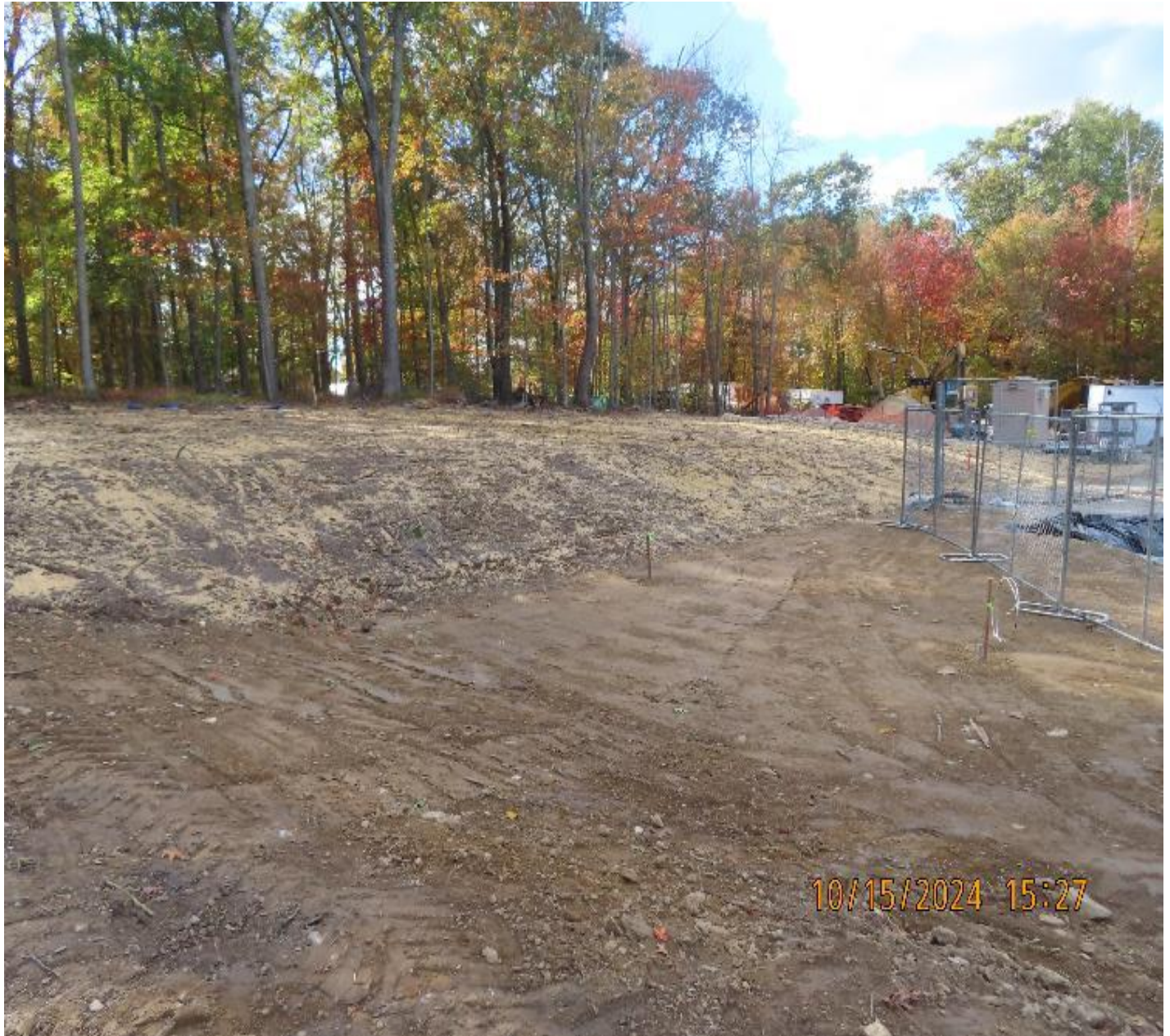
Photo 6: View (looking west) of southern portion of site where final grading and partial stabilization work has been completed.
