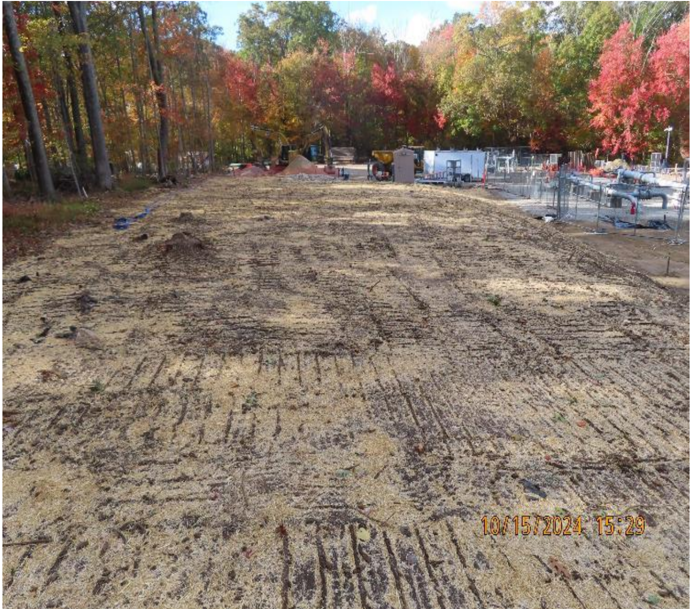
Photo 7: View (looking northwest) of area recently graded, seeded, and mulched. Additional mulch and application and crimping is planned for this area for further stabilization.
