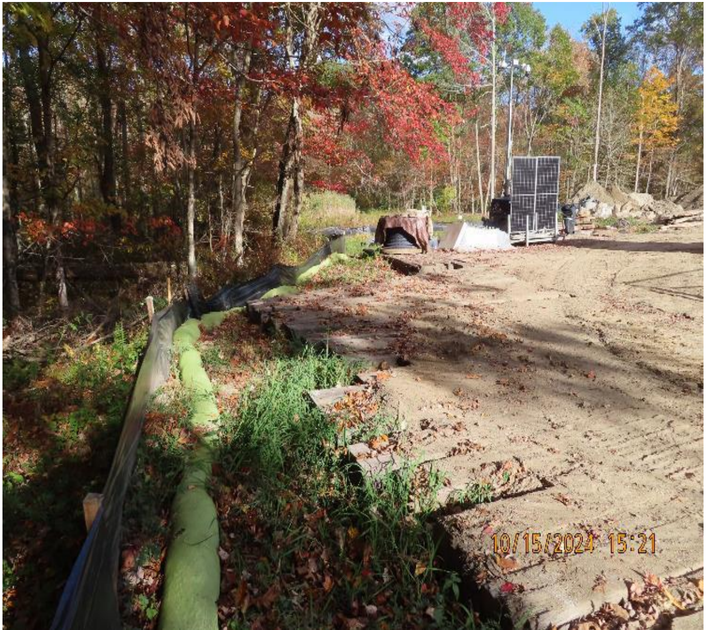
Photo 2: View (looking northeast) of silt fence and filter sock along perimeter of western workspace.
