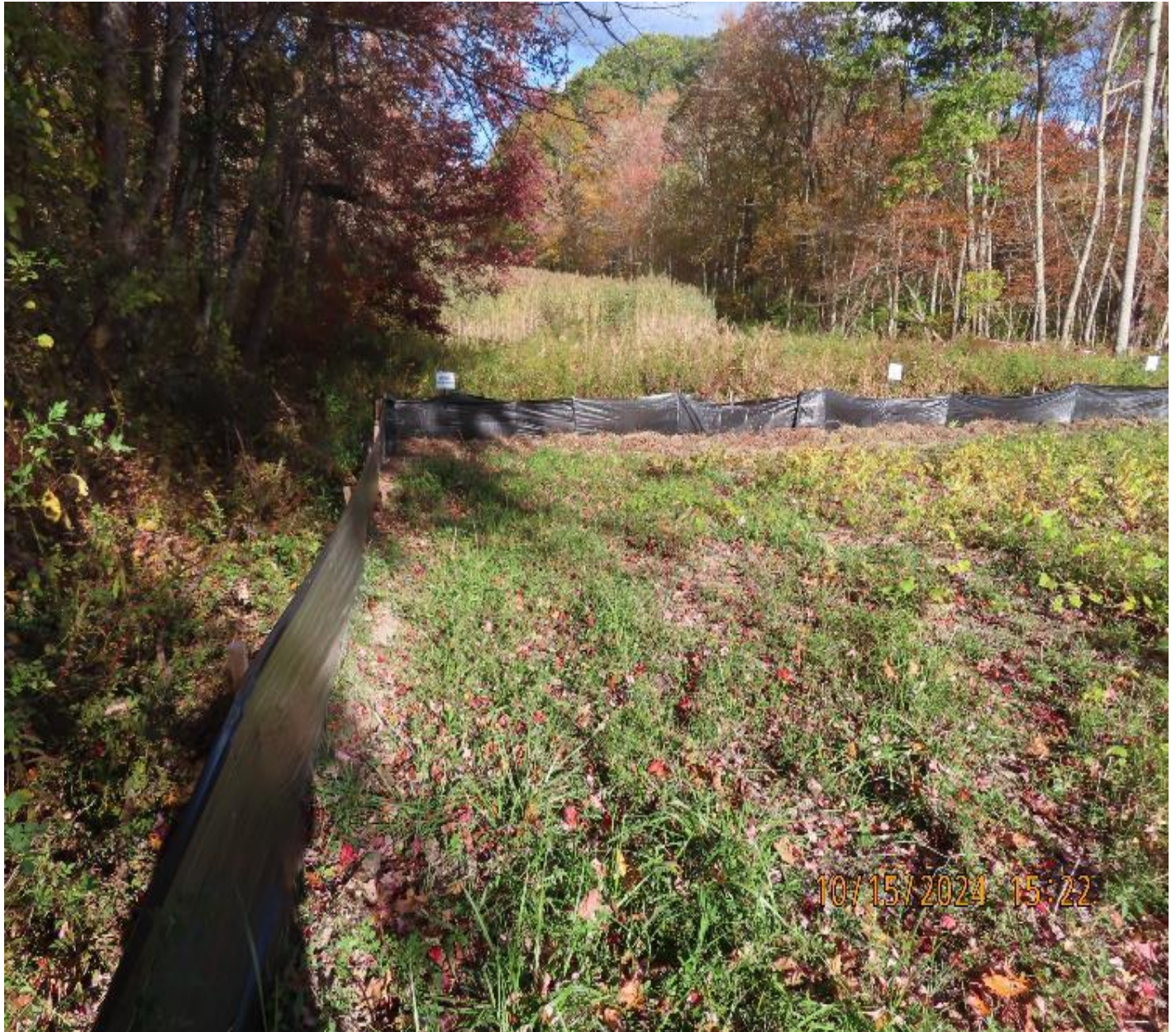
Photo 3: View (looking northwest) of silt fencing and vegetative buffer near wetland at southwest corner of site.
