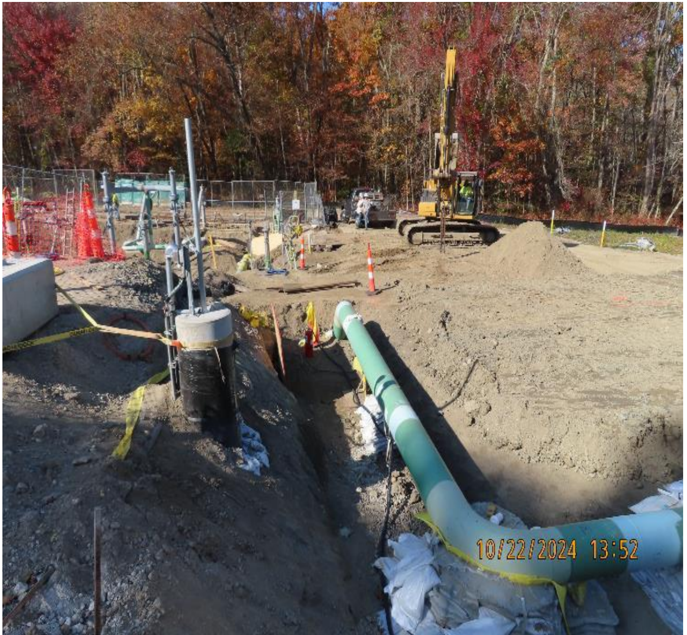
Photo 4: View (looking northwest) of backfill work along 16-inch inlet piping and tie-in point.
