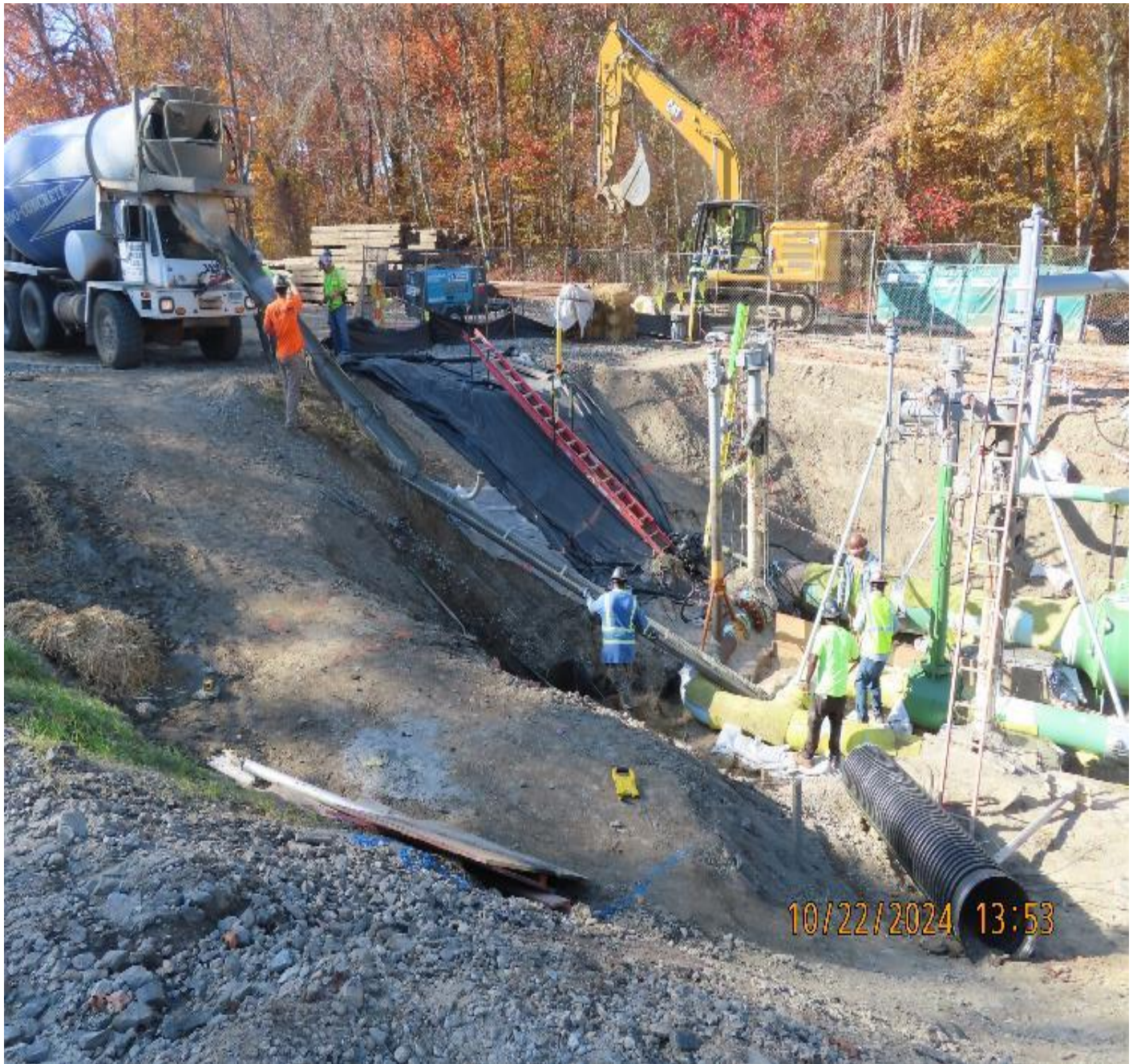
Photo 3: View (looking northwest) of concrete supports being installed in valve yard excavation.
