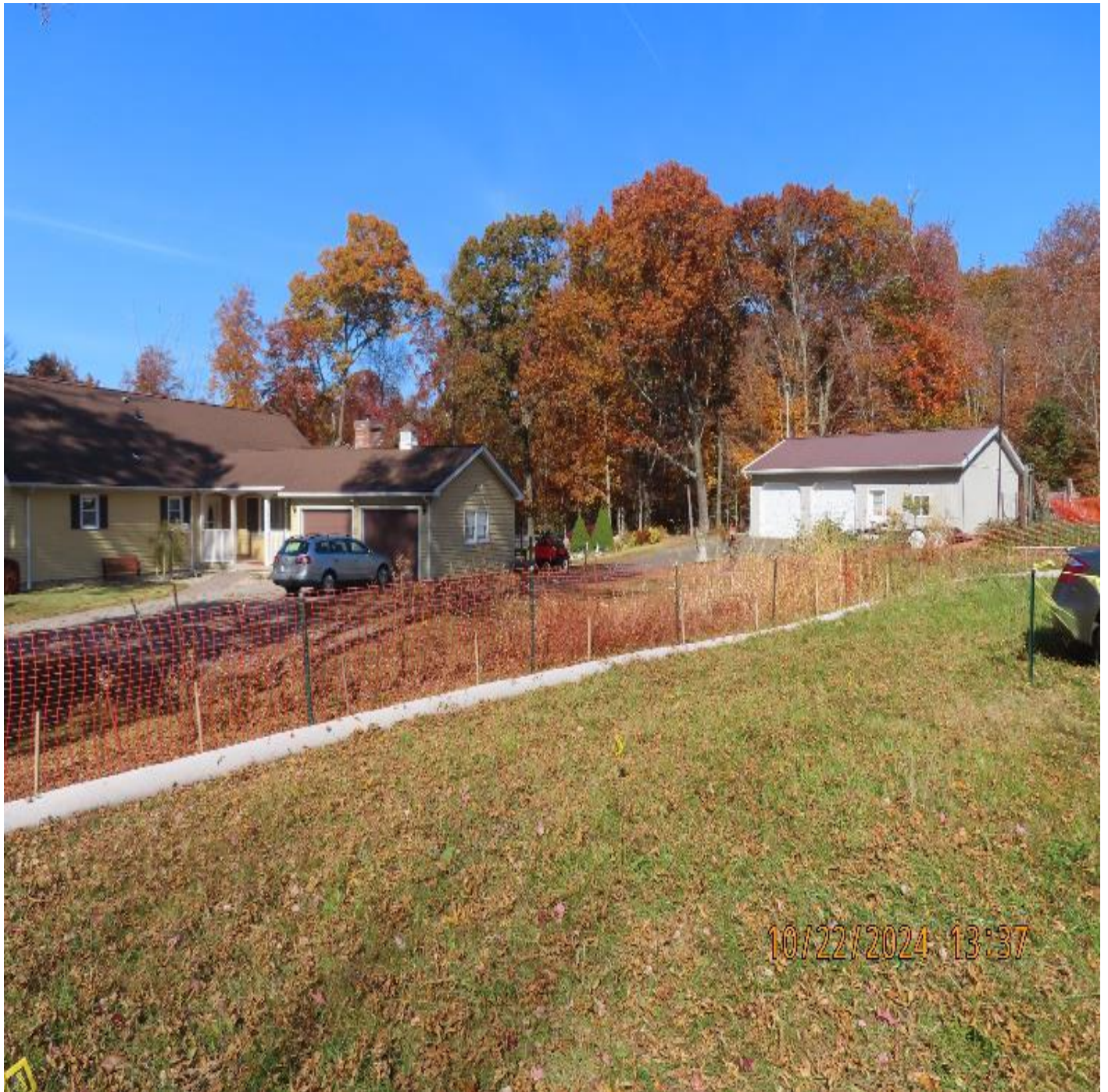
Photo 2: View (looking northwest) of perimeter ECDs and security fencing along west side of site access.
