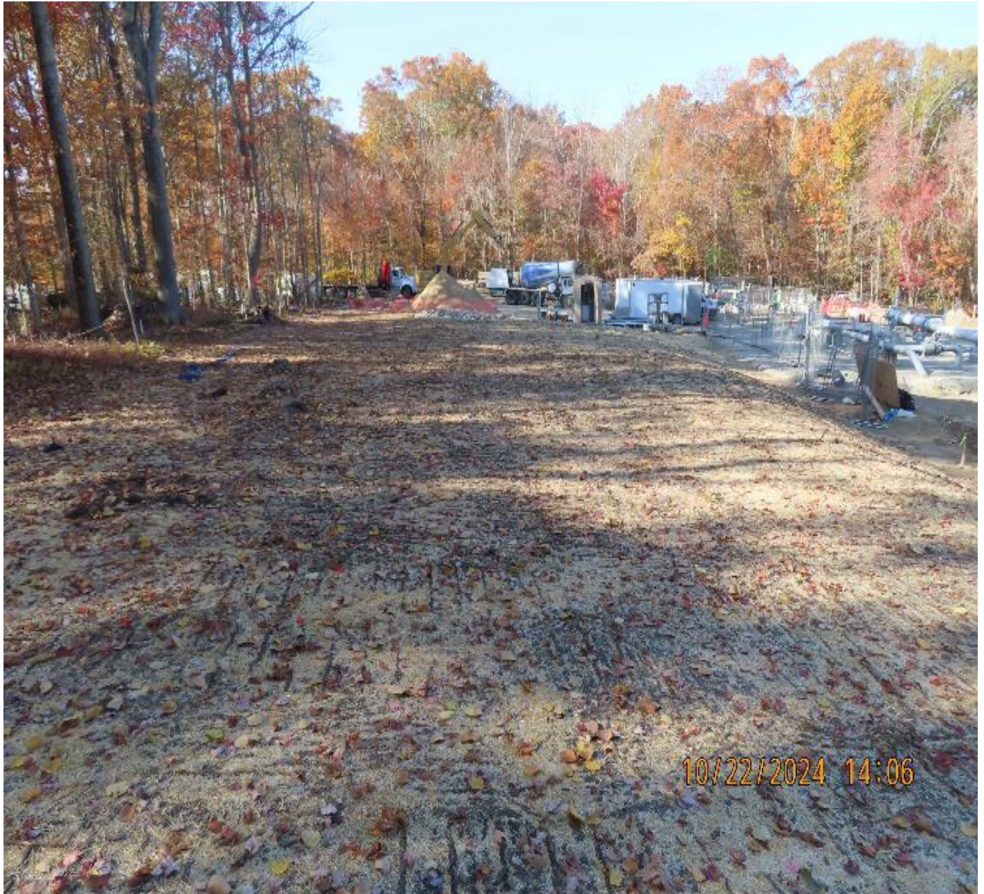
Photo 7: View (looking west) of stabilized soil conditions where construction is complete in southern portion of site.
