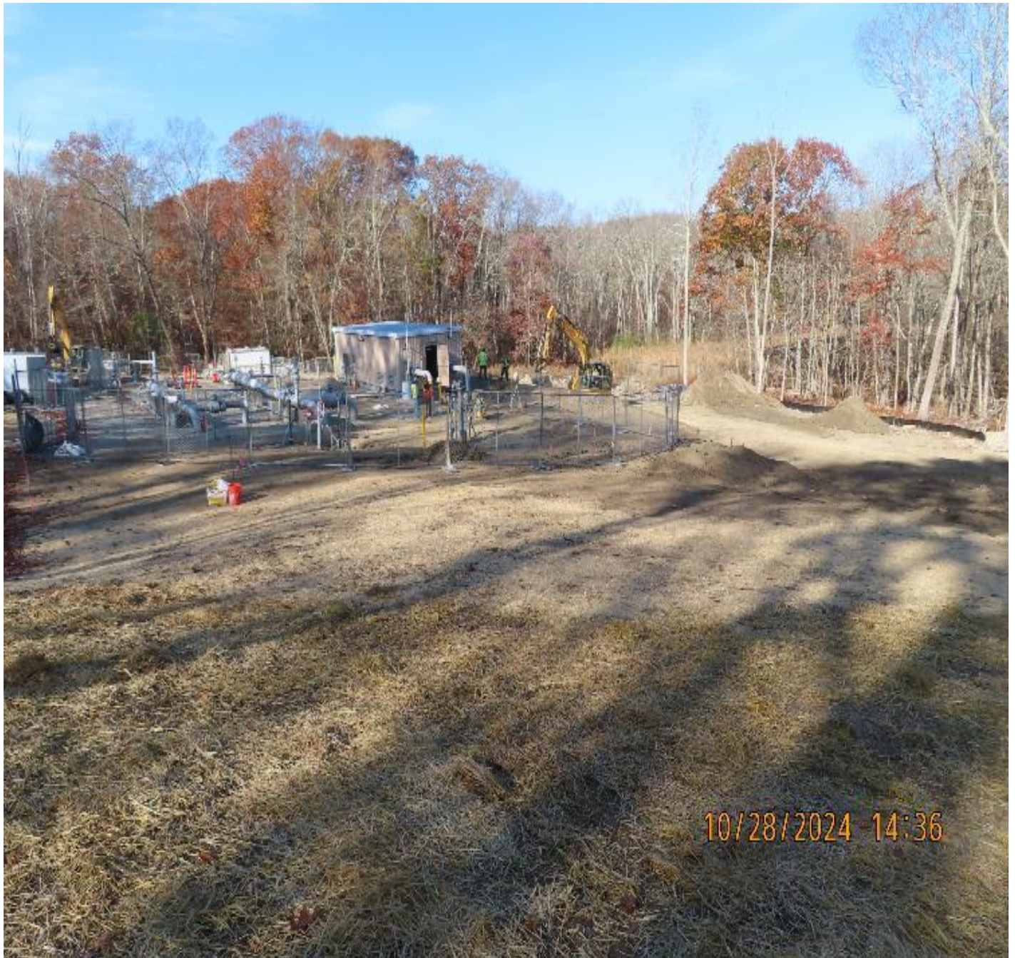
Photo 5: View (looking north) of backfill and grading work around valve yard and diminishing spoil piles.
