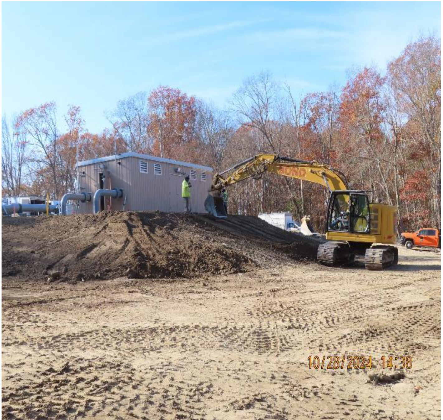
Photo 6: View (looking west) of grading work to contour slope along north side of new regulatory building.
