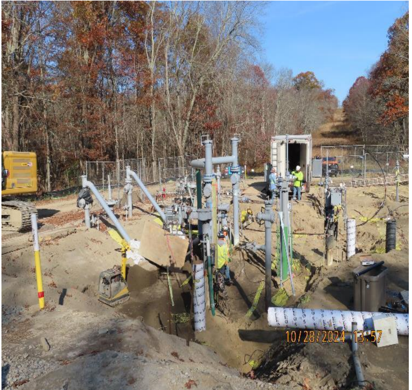
Photo 3: View (looking northeast) of valve yard after backfilling progressed to where excavation dewatering is no longer needed.
