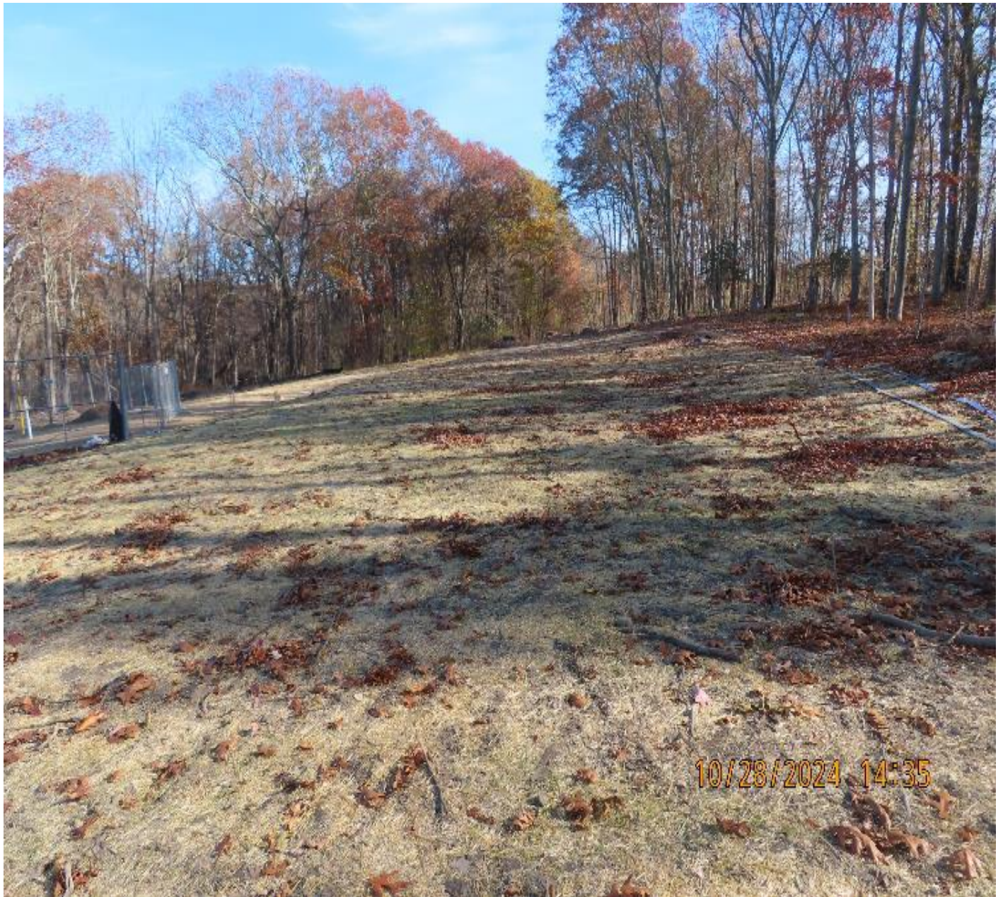
Photo 4: View (looking southeast) of south side of work site after seed and straw mulch application.
