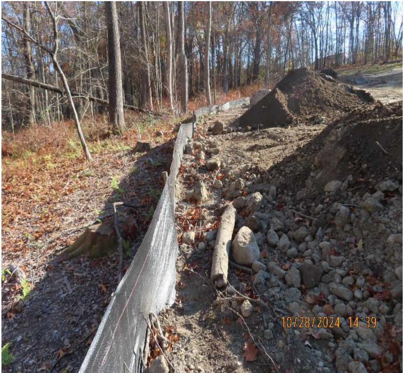
Photo 7: View (looking southeast) of perimeter silt fence along north side of work site.
