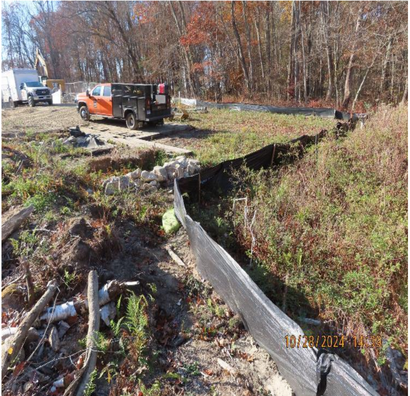
Photo 8: View (looking west) of perimeter silt fence protecting wetland W-CZ-01 (northeast corner of work site)
