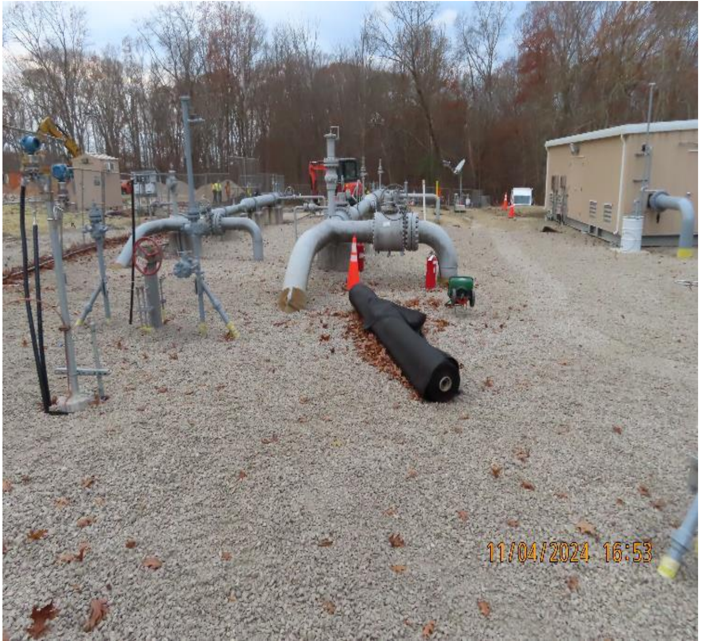
Photo 6: View (looking northwest) of former E-System tie-in excavations after backfilling, final grading, and surface gravel installation.
