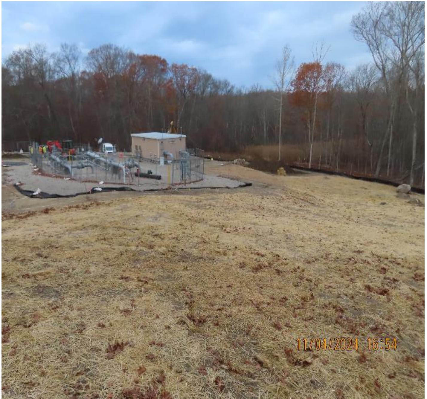
Photo 7: View (looking northwest) of stabilized areas east of the new regulator building.
