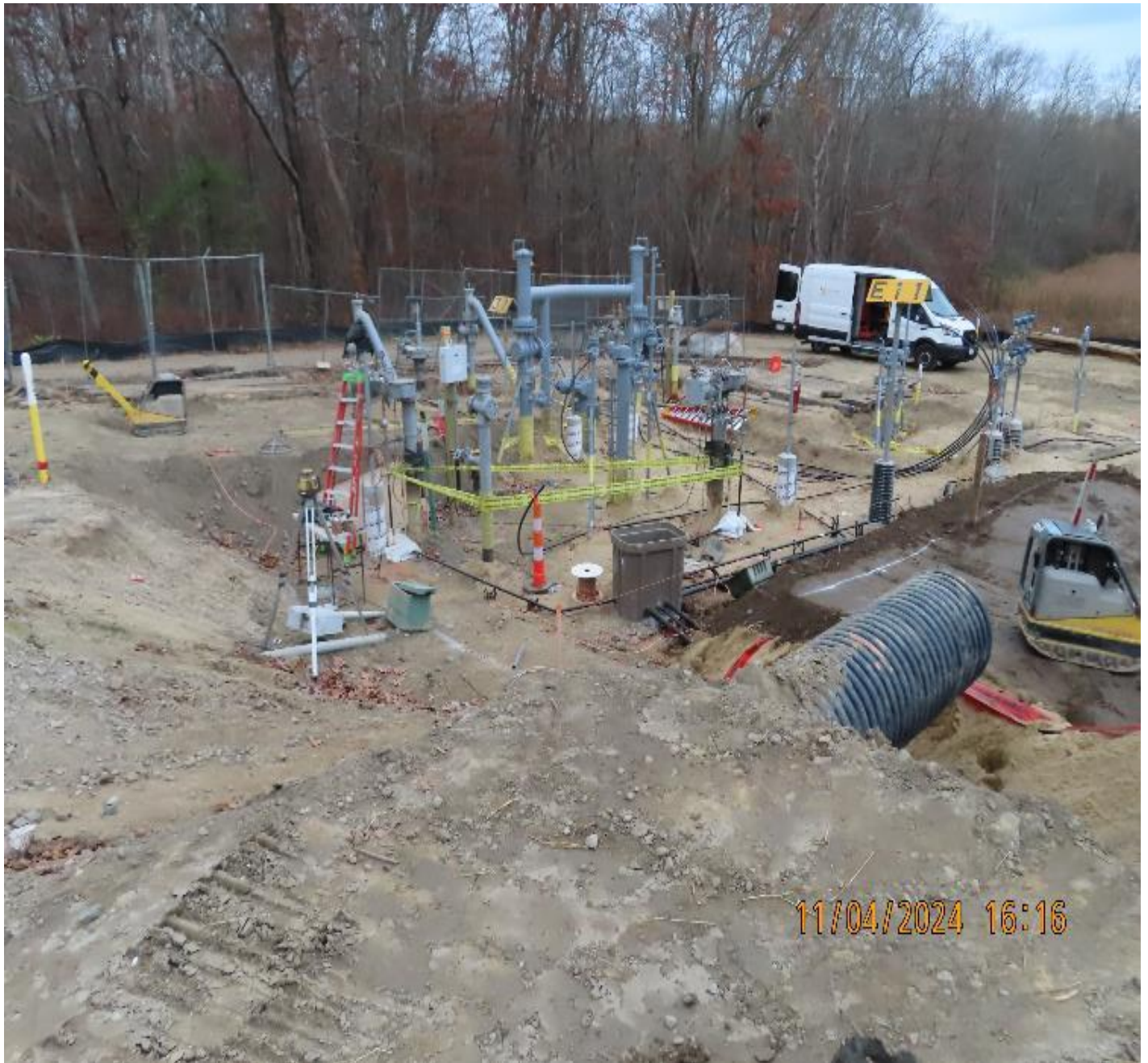
Photo 4: View (looking northwest) of backfilling and grading progress in the valve yard.
