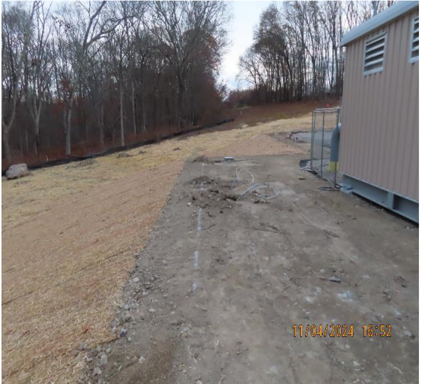
Photo 5: View (looking southeast) of sloped area restored with erosion control blanket north of the new regulator building.
