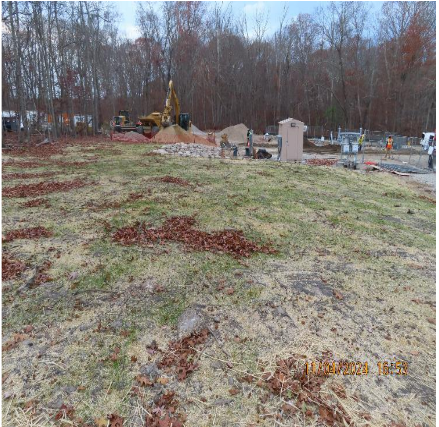
Photo 2: View (looking northwest) of grass germination progress in south portion of the work site.
