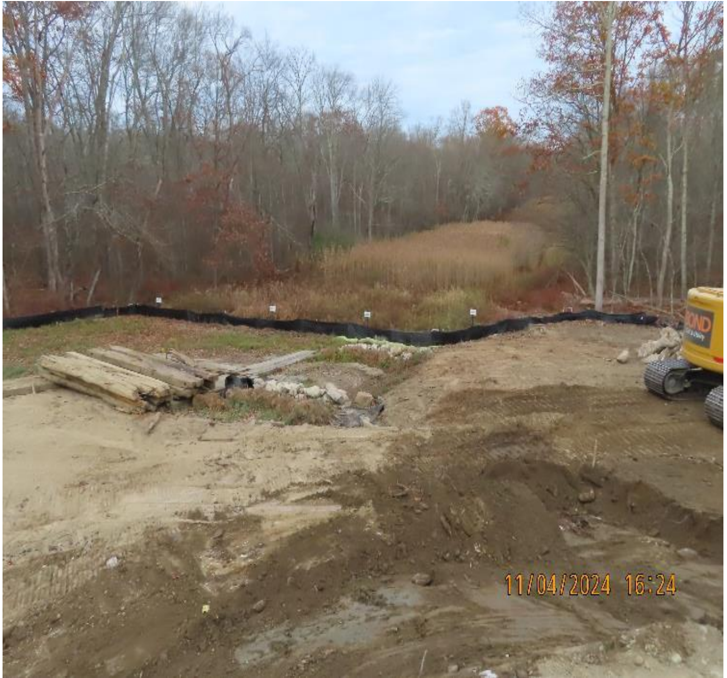
Photo 3: View (looking northeast) of clean-up work underway as mats are removed and final grading is completed near the north boundary of the work site.
