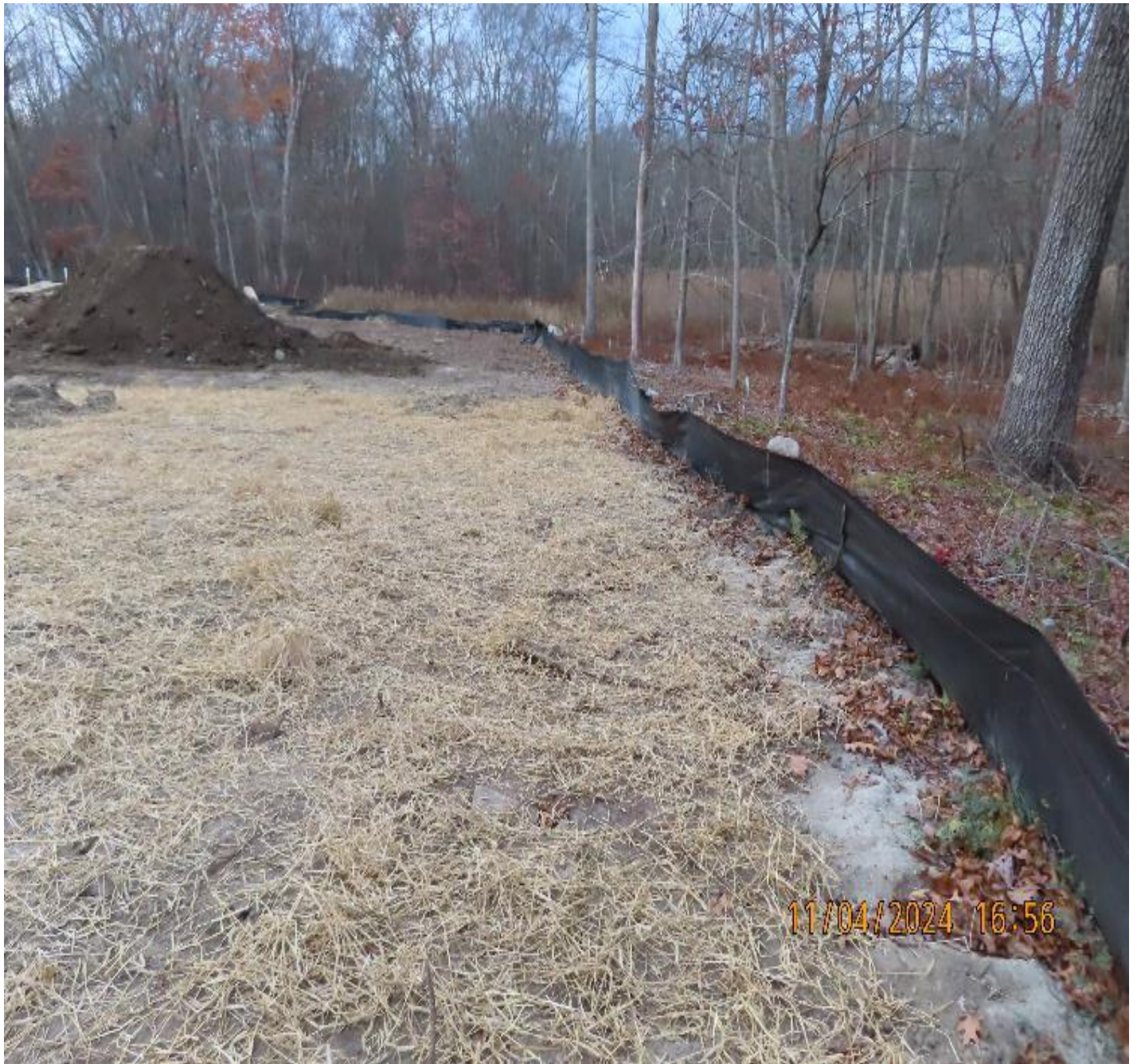
Photo 8: View (looking northwest) of perimeter silt fence downslope of northern portions of the work site.
