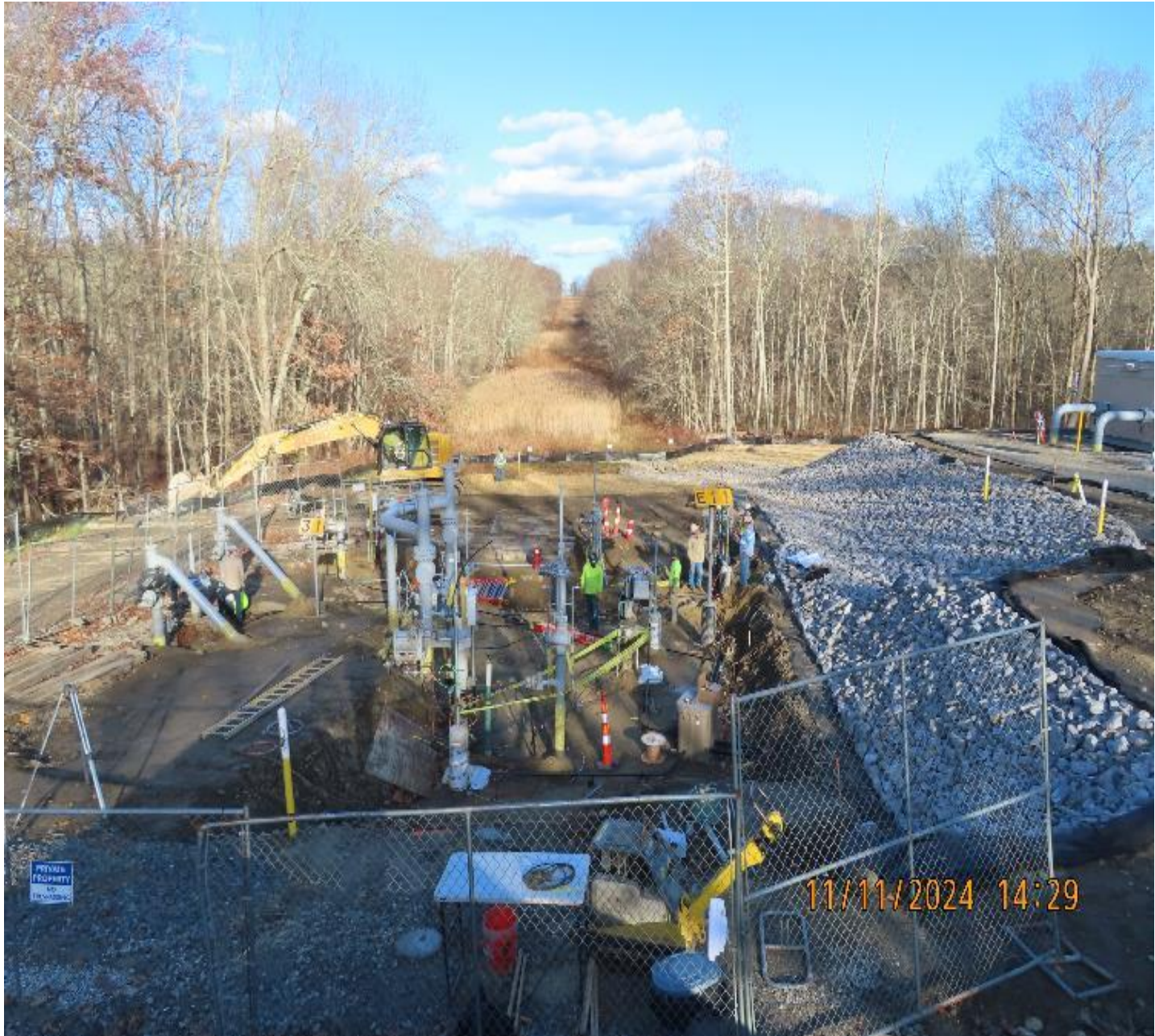
Photo 5: View (looking northeast) of valve yard area where backfilling and grading work is approximately 90 percent complete. Note culvert replacement and riprap installation in the drainage swale.
