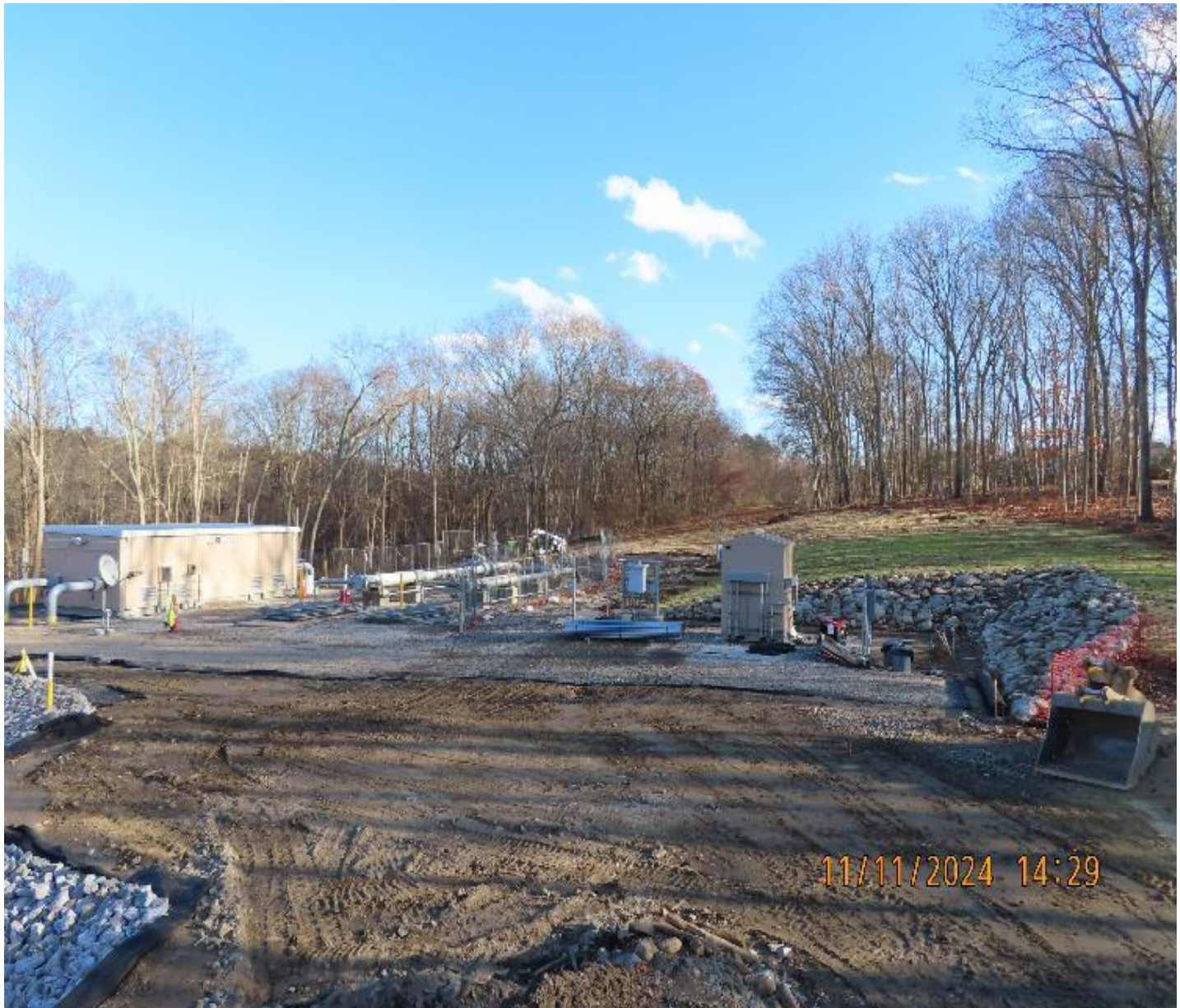
Photo 3: View (looking southeast) of valve yard and new regulator building.
