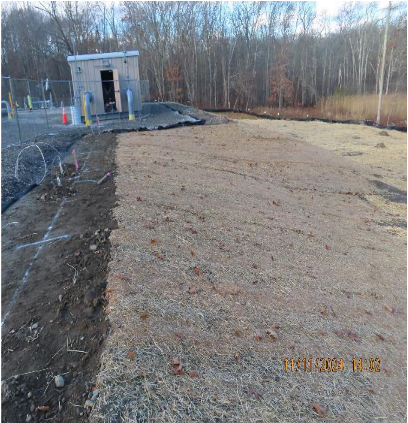
Photo 8: View (looking northwest) of stabilized area on northeast side of new regulator building.
