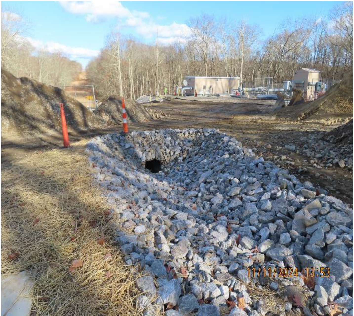
Photo 6: View (looking northeast) of replaced 24-inch culvert and new riprap placed in drainage swale.
