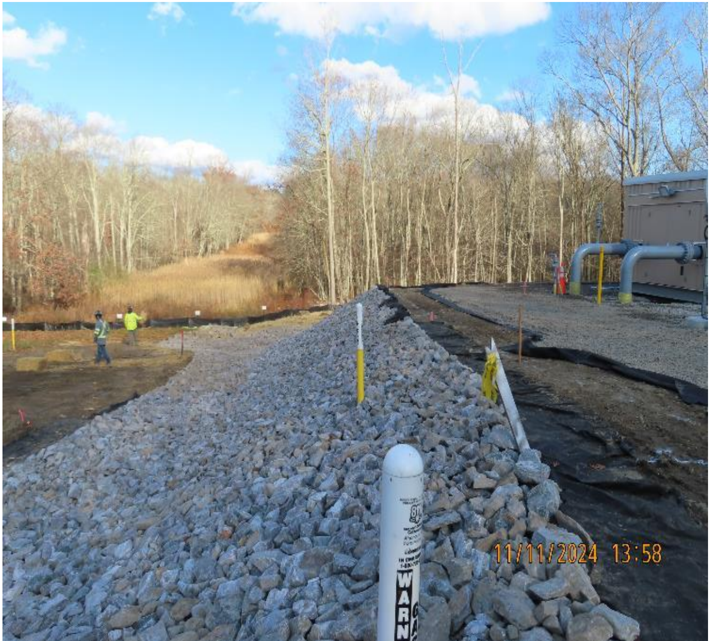
Photo 7: View (looking north) of riprap installation on slope northwest of new regulator building.
