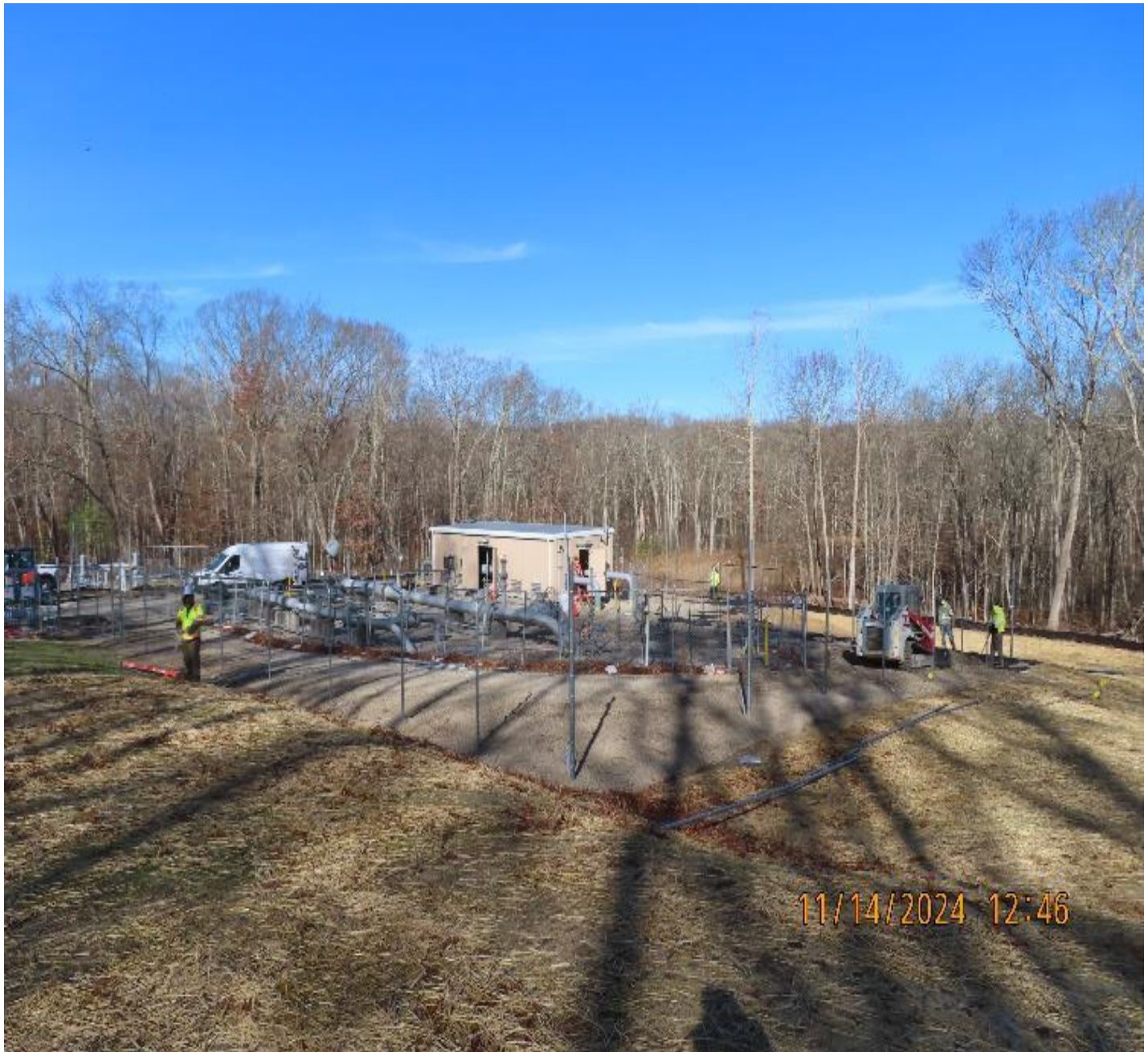
Photo 5: View (looking northwest) of new regulator site as permanent security fencing is being installed.
