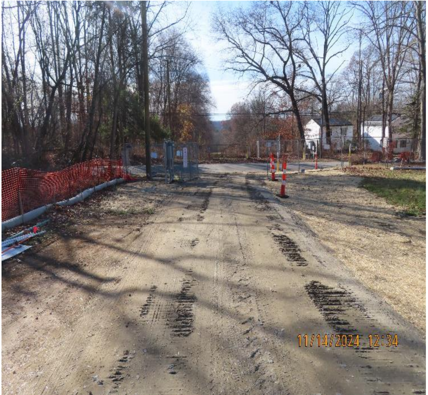
Photo 7: View (looking northeast) of worksite entrance after crushed rock applied for permanent improvement.
