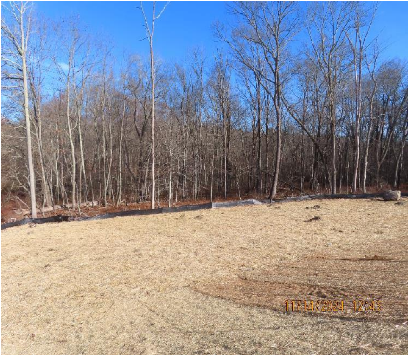
Photo 4: View (looking northeast) of restored and stabilized sloped area along northern portion of the worksite.
