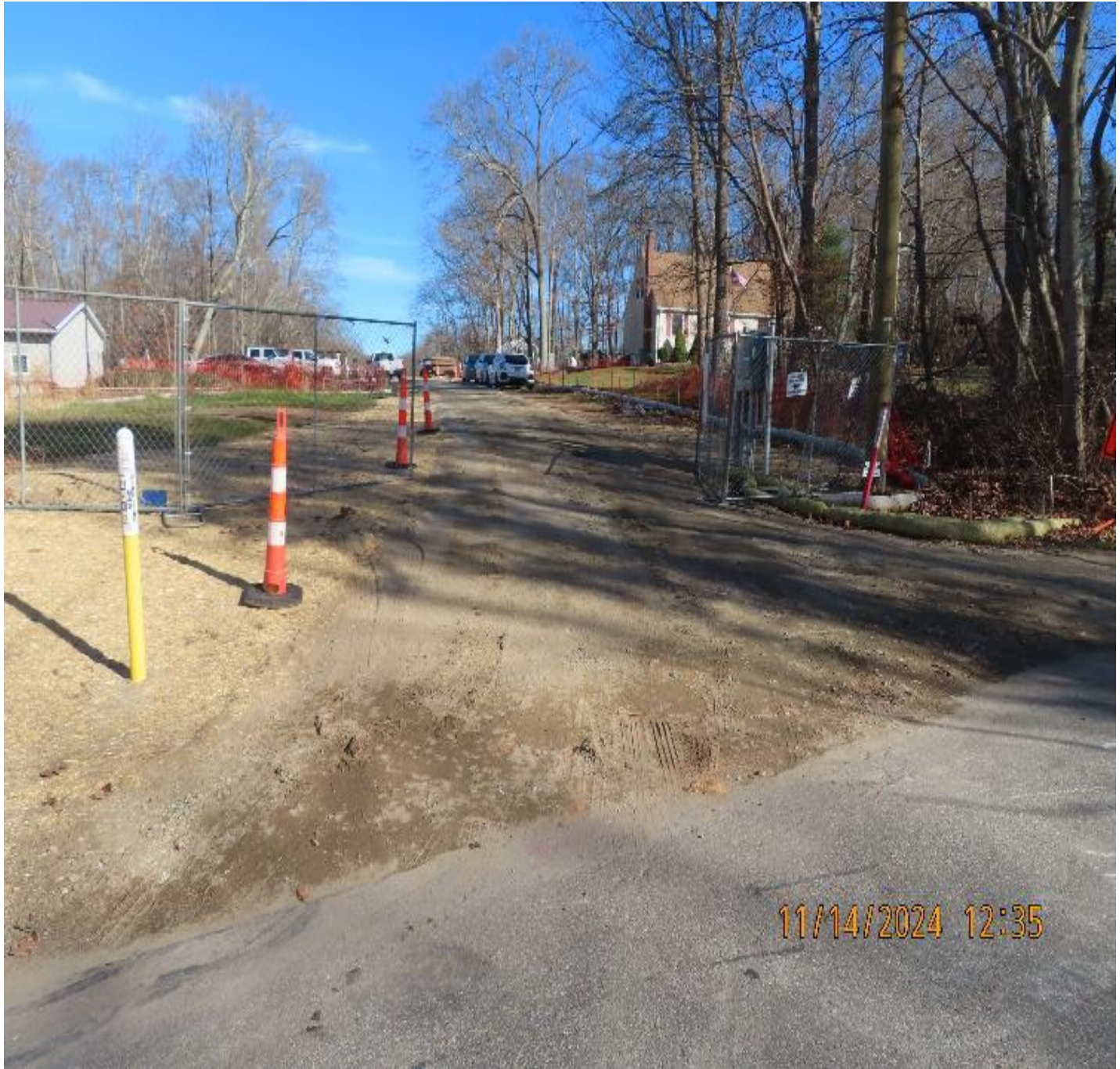
Photo 8: View (looking northeast) of worksite entrance after crushed rock applied to access road.
