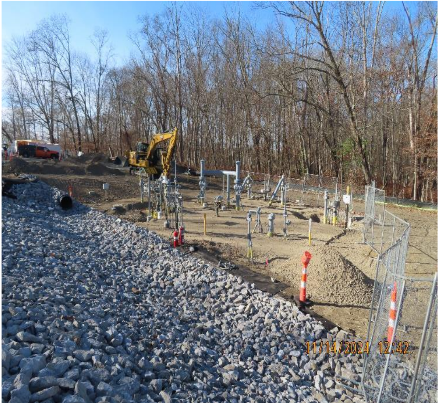
Photo 3: View (looking west) of remaining backfilling work being completed in valve yard. Placement of rock riprap is complete.
