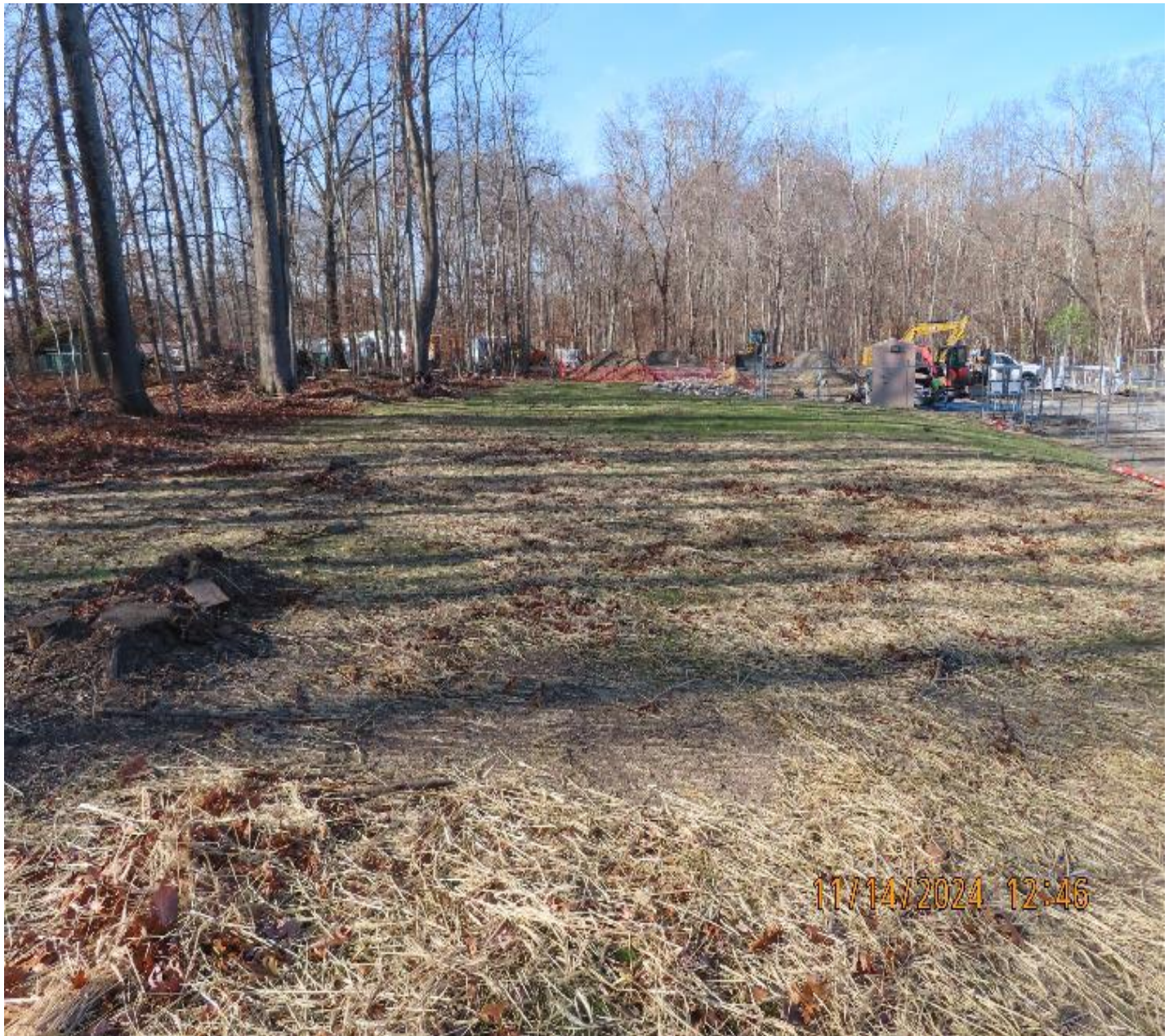
Photo 6: View (looking west) of restored and stabilized conditions in southern portion of the worksite.
