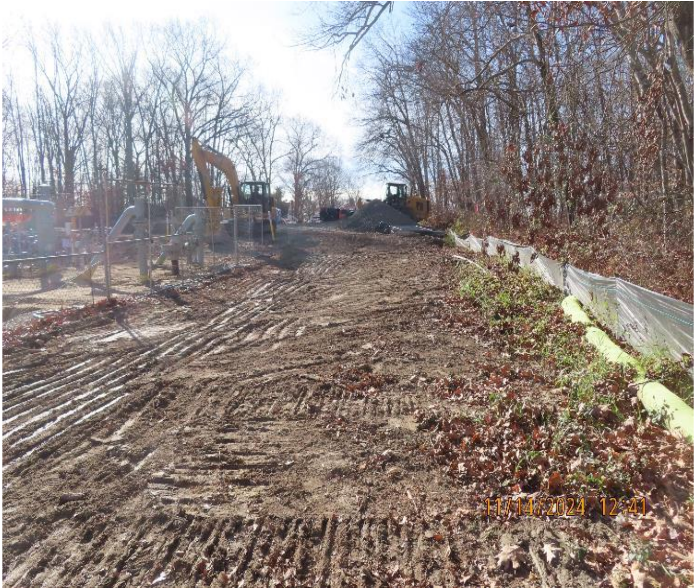
Photo 2: View (looking southwest) of west side of the valve yard where mats have been removed to prepare for placement of gravel surfacing for permanent access improvements.
