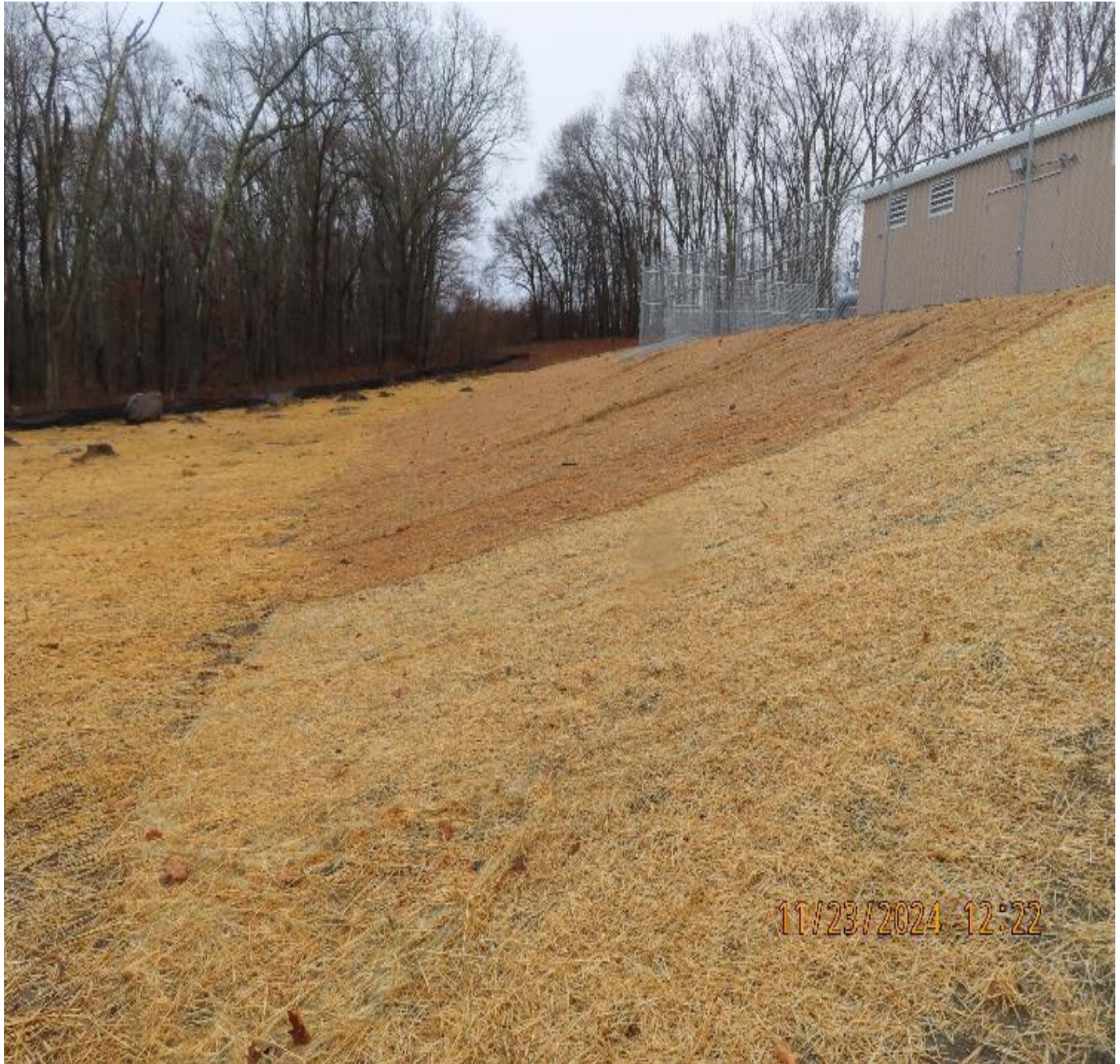
Photo 7: View (looking southeast) of stabilized slope along the northeast side of the new regulator building.
