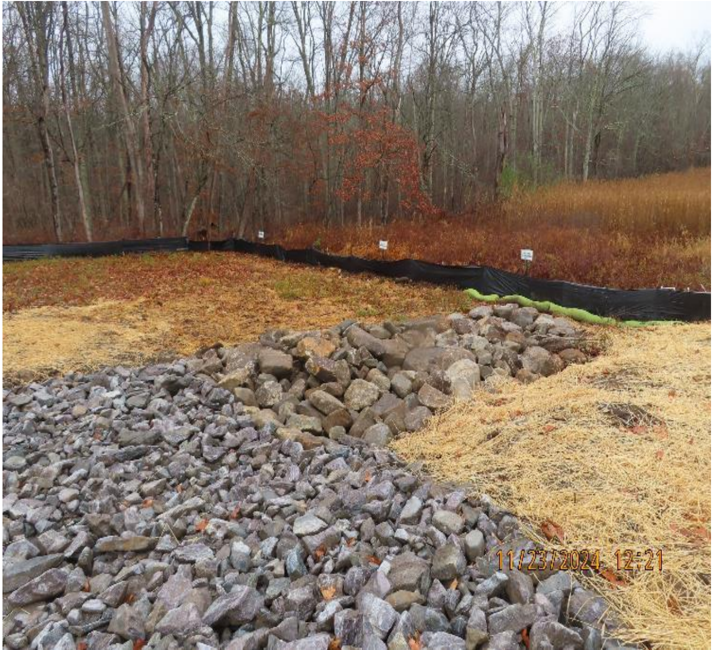
Photo 6: View (looking north) of riprap armored drainage swale that directs stormwater runoff away from the site.
