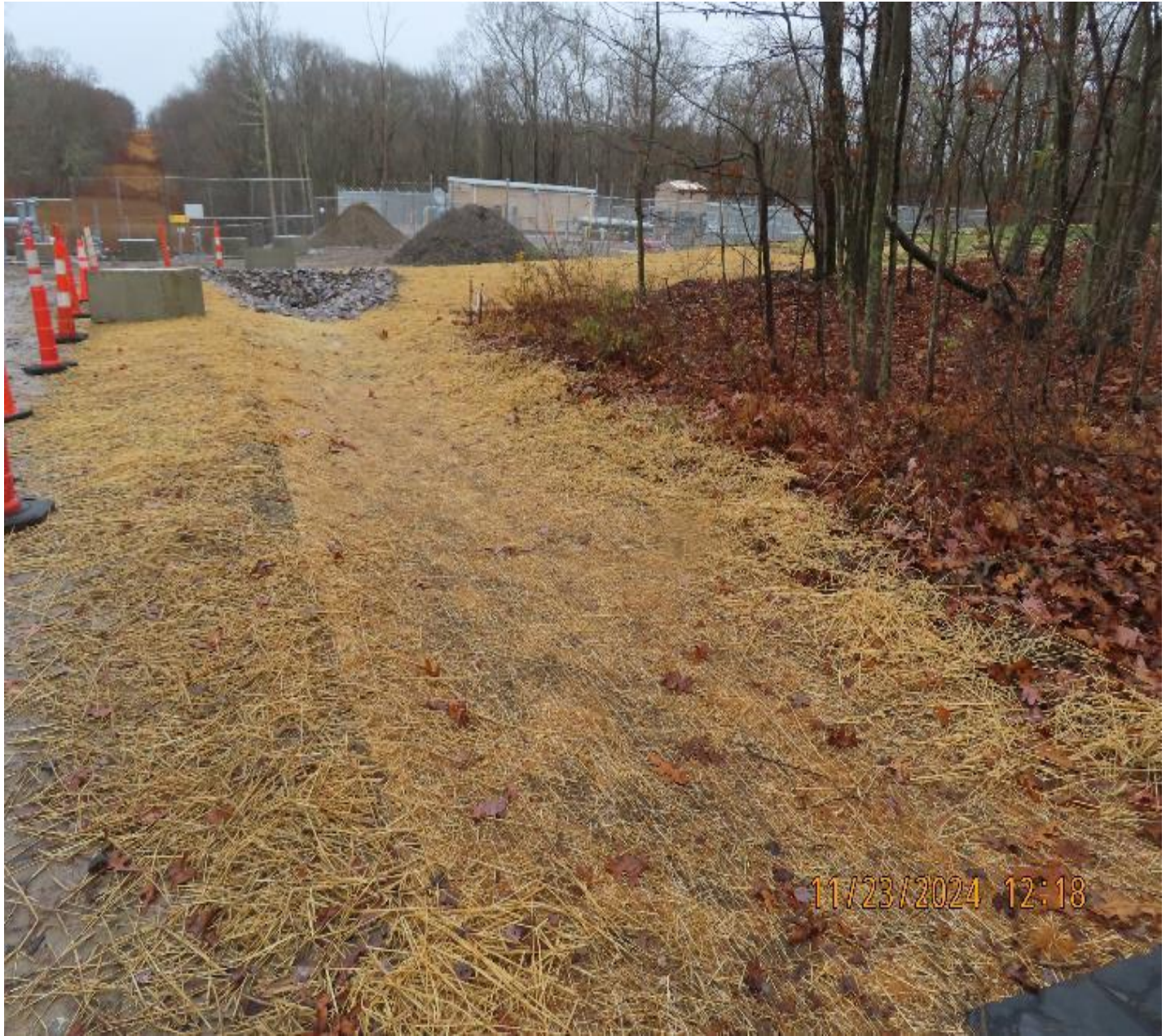
Photo 3: View (looking northeast) of stabilized drainage swale that bisects the site southwest to northeast
