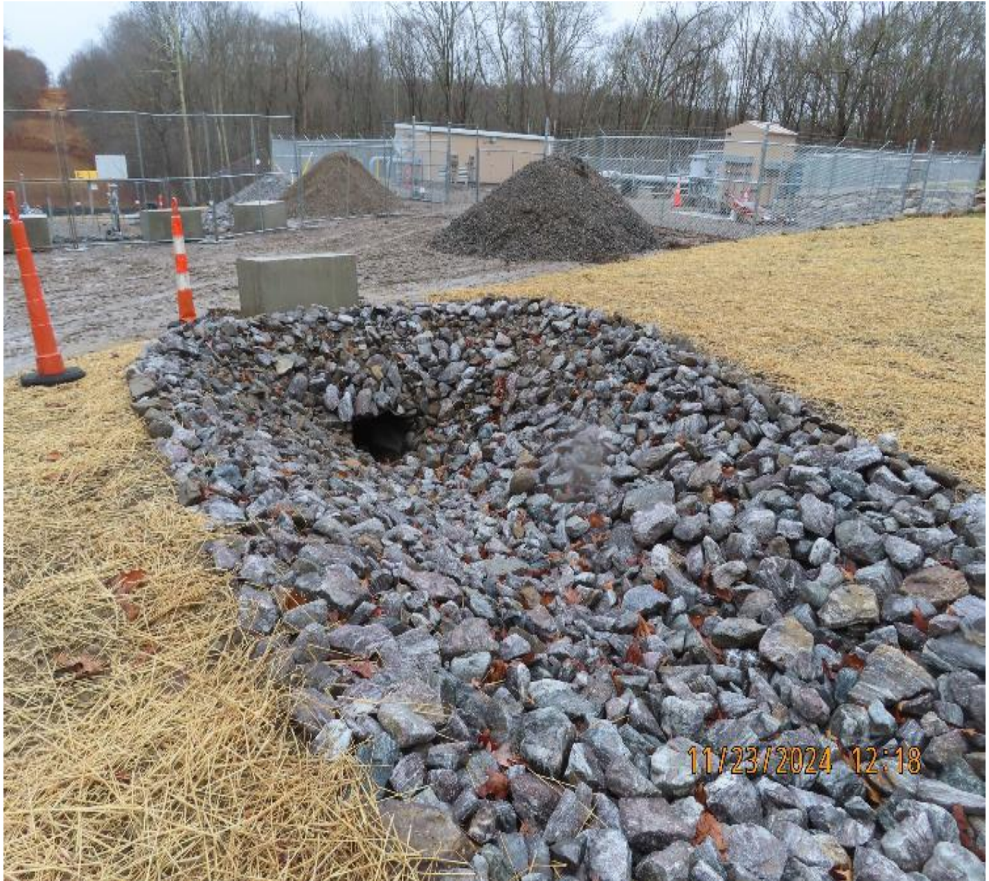
Photo 4: View (looking northeast) of riprap installed around entrance to the culvert that runs beneath the access road to the regulator and RTU buildings.
