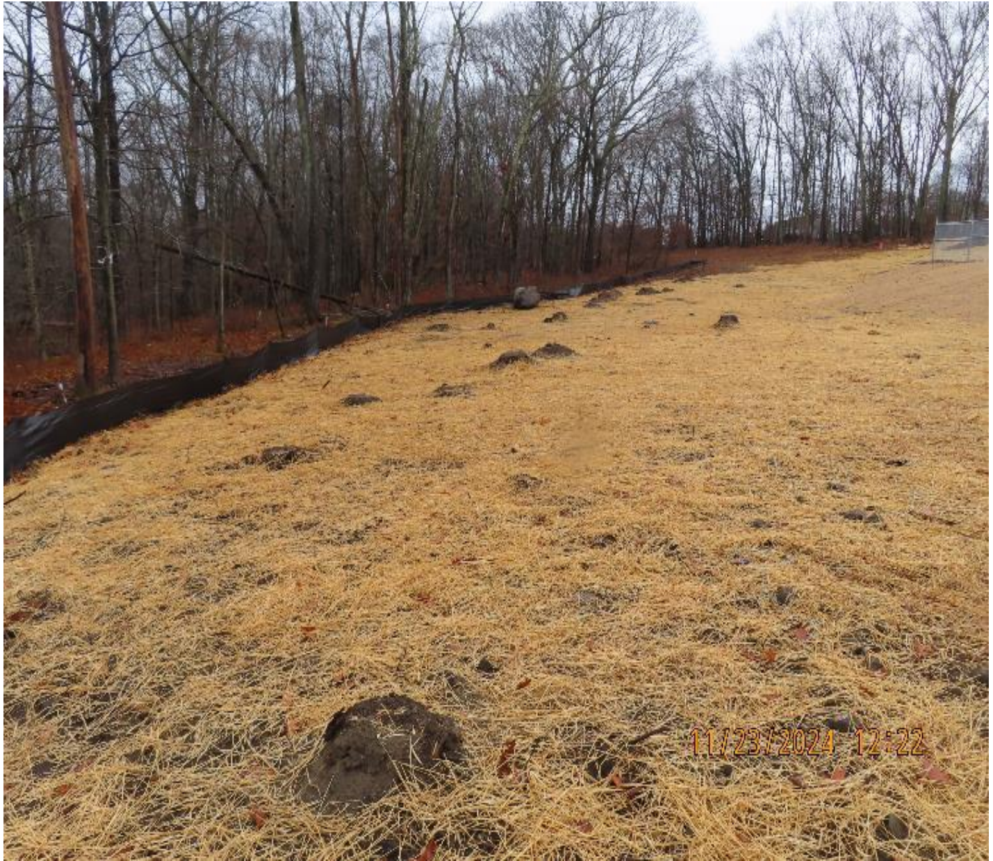
Photo 8: View (looking southeast) of winter stabilization conditions in eastern part of the worksite. The brown clumps are tree stumps that were left in place.
