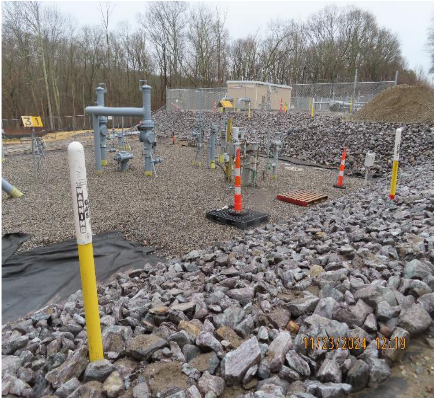
Photo 5: View (looking east) of valve yard with stone surfacing work at approximately 80 percent complete.
