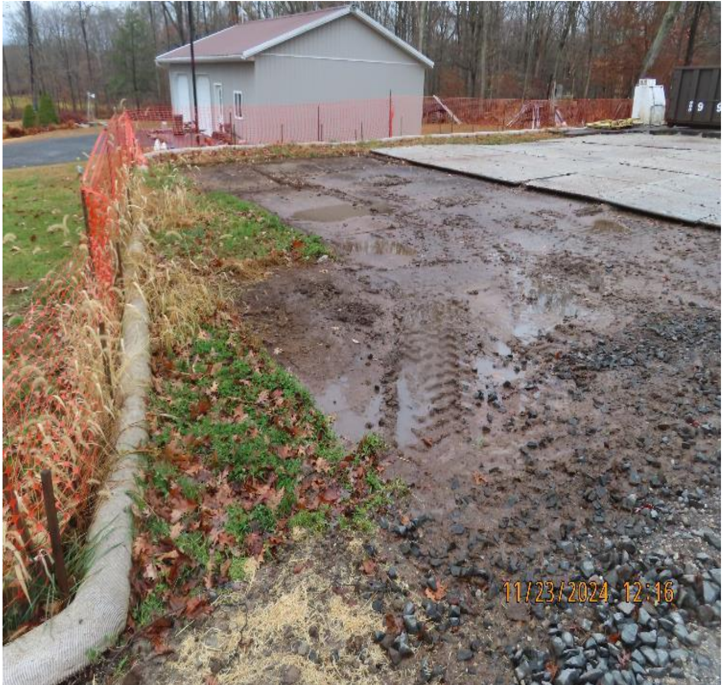
Photo 2: View (looking northwest) of ground surface of workspace immediately after removal of composite matting (before seed application and temporary stabilization).
