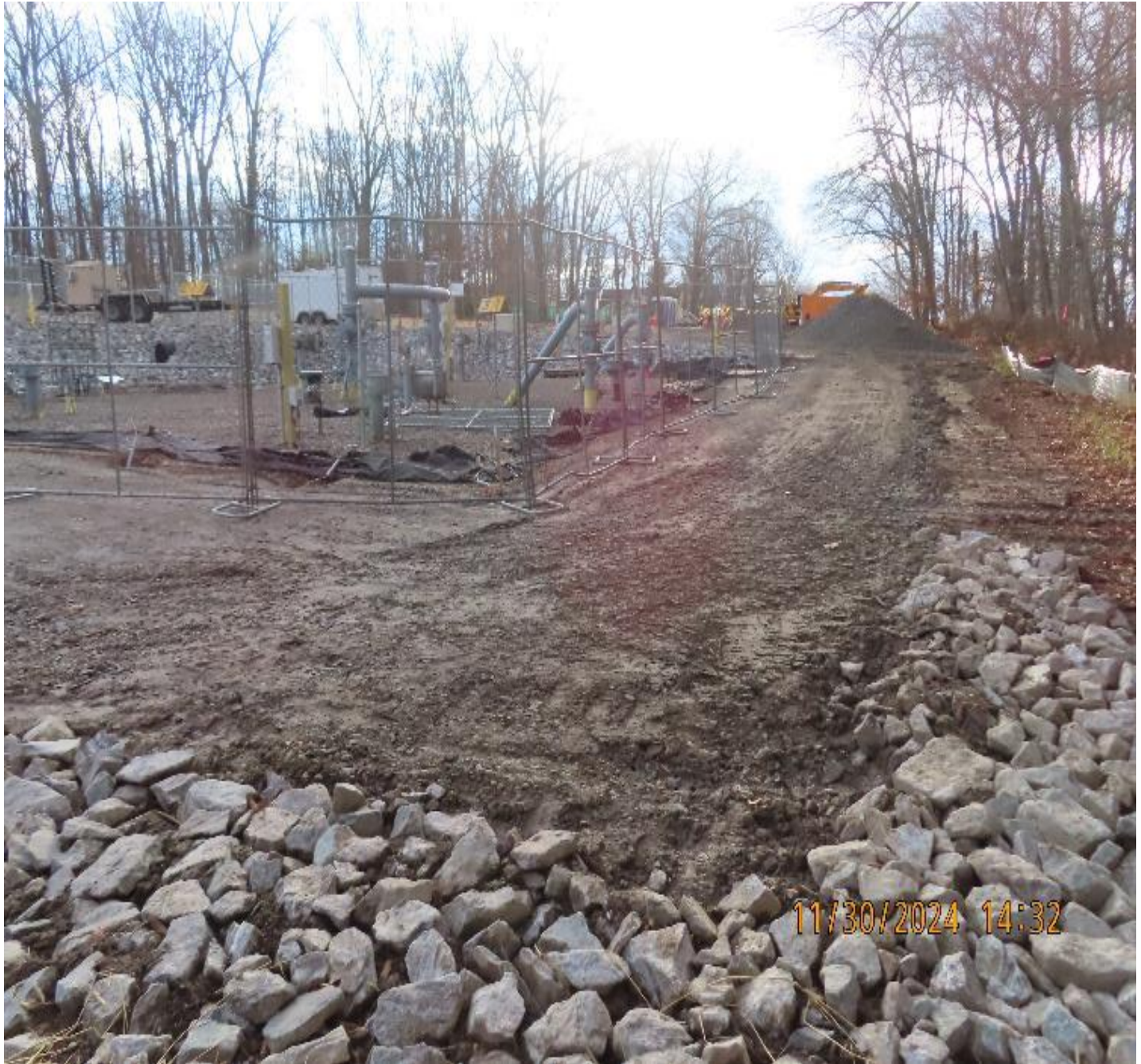
Photo 5: View (looking southwest) of new access road along west side of the valve yard after rough grading.
