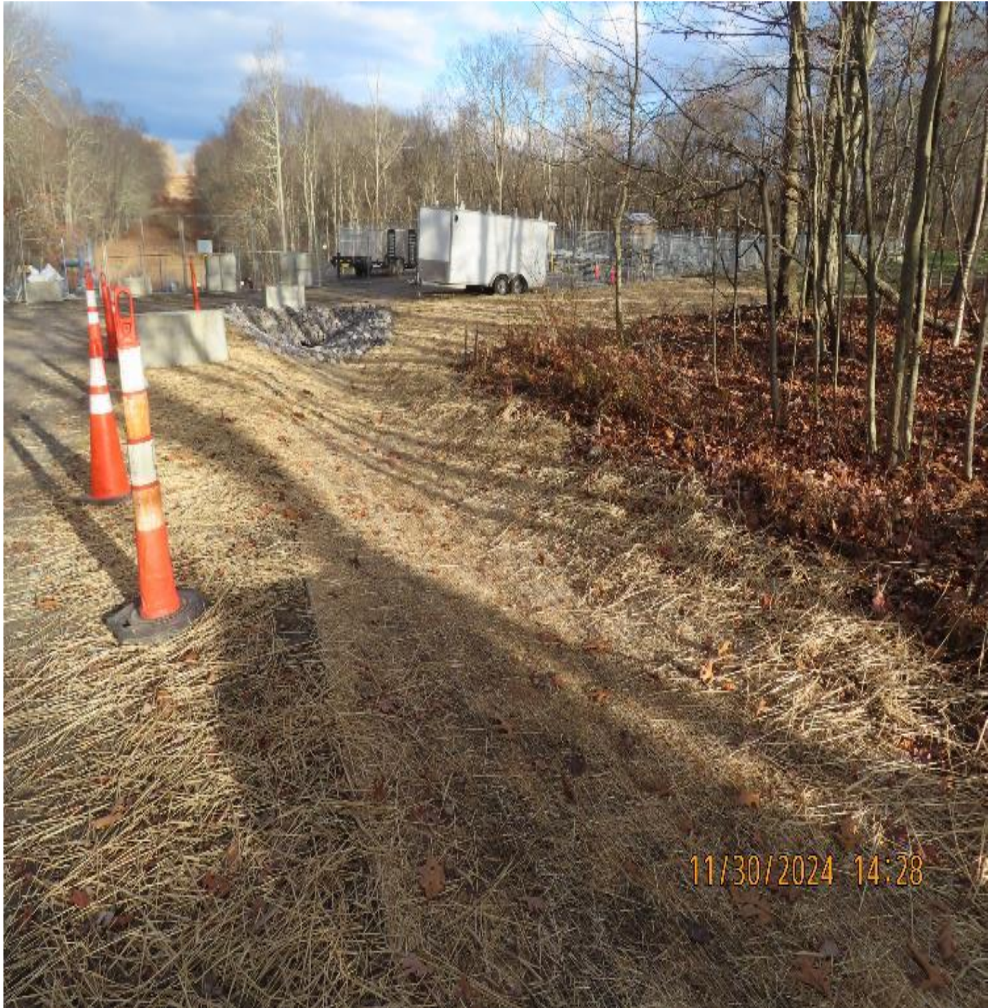
Photo 3: View (looking northeast) of stormwater swale along southwest side of valve yard after grading and temporary stabilization work.
