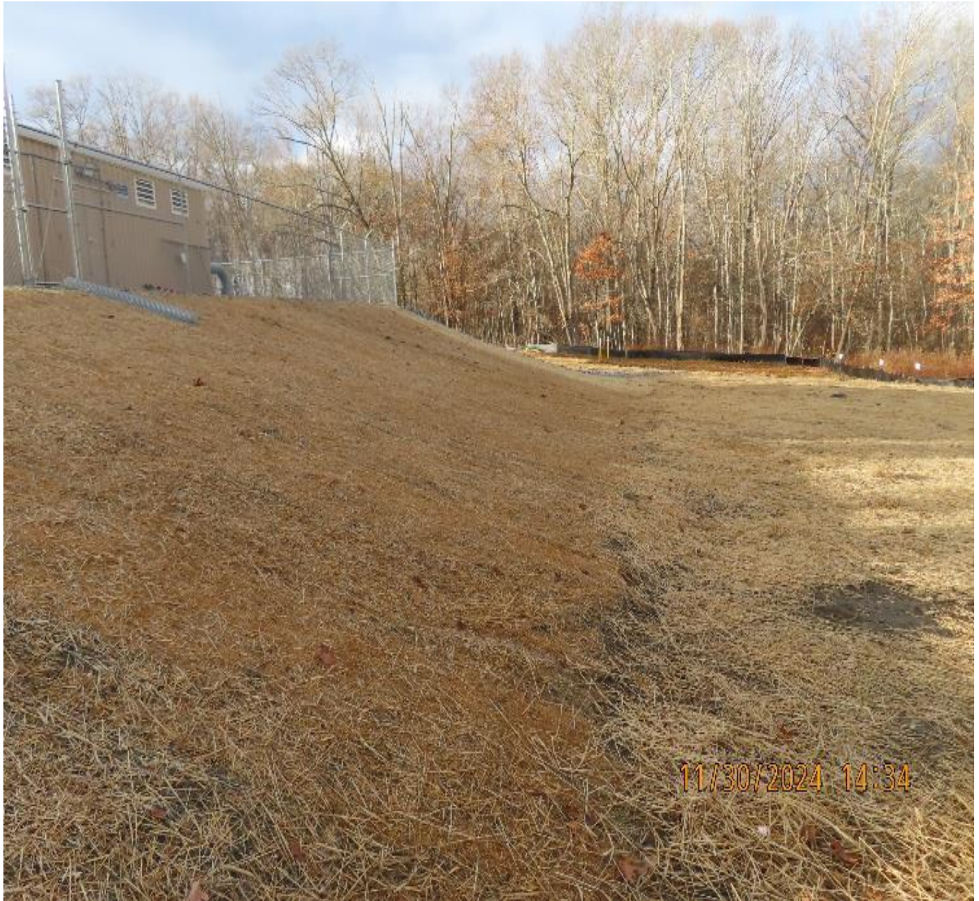
Photo 7: View (looking northwest) of stabilized slope along north side of new regulator building.
