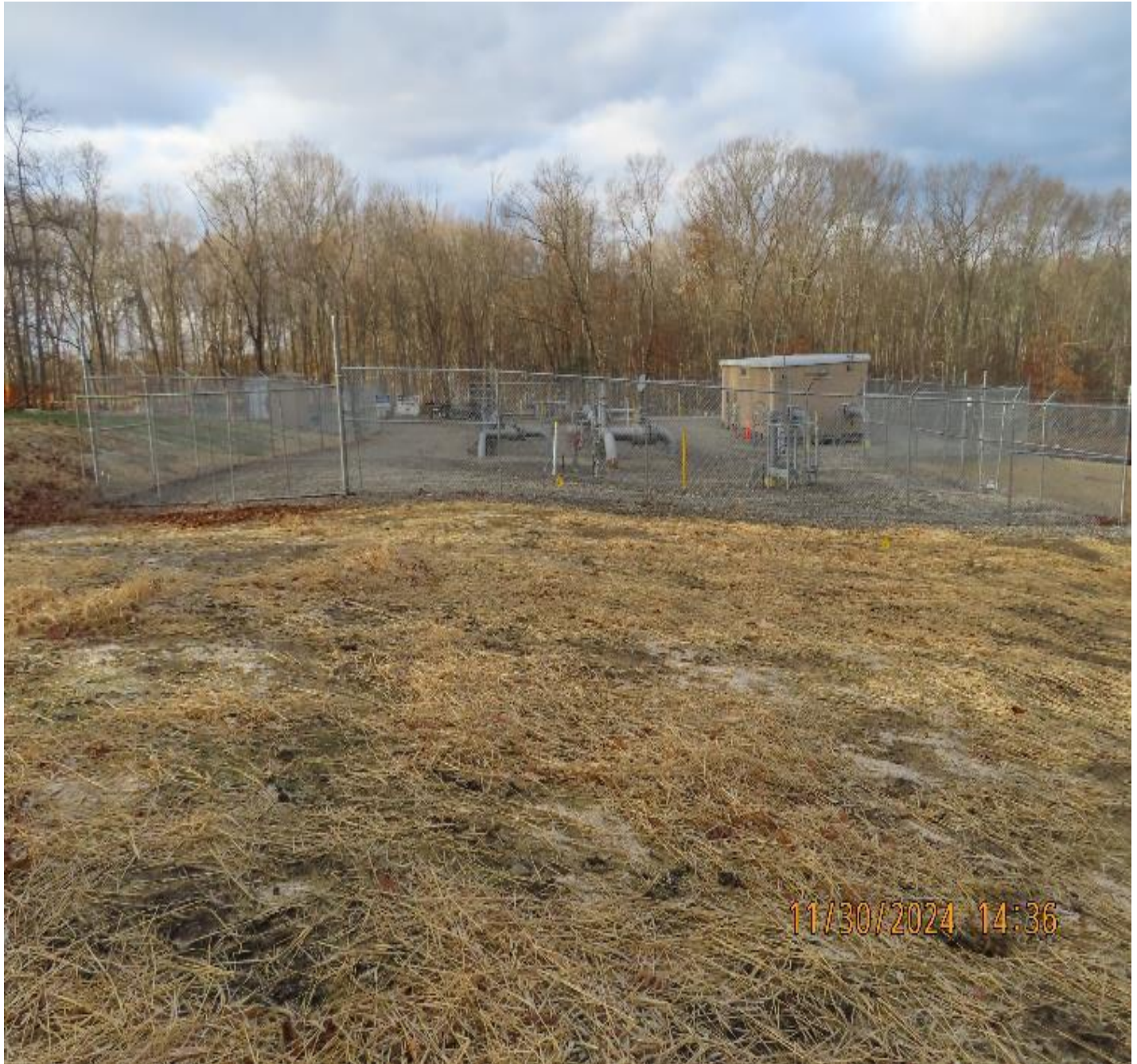
Photo 8: View (looking northwest) of valve yard after stone surfacing work was complete.
