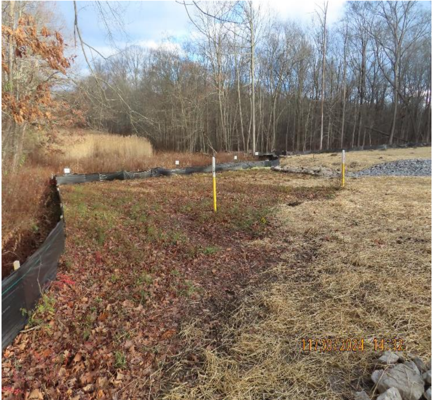
Photo 6: View (looking northeast) of silt fencing and recently stabilized ground downslope of the main work area.
