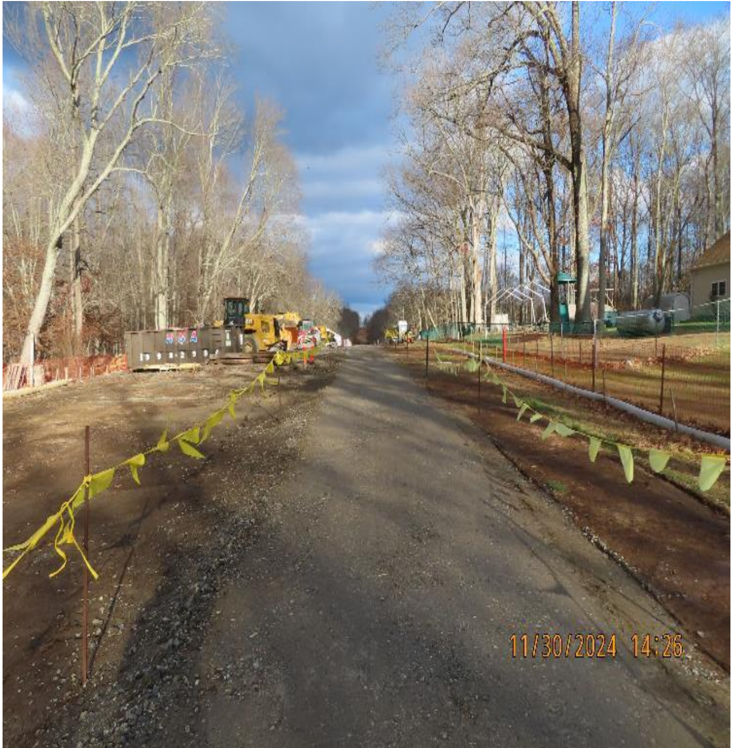
Photo 2: View (looking northeast) of access road after mats placed along the edges for parking and materials staging were removed. Soil decompaction and stabilization work in this area is pending.
