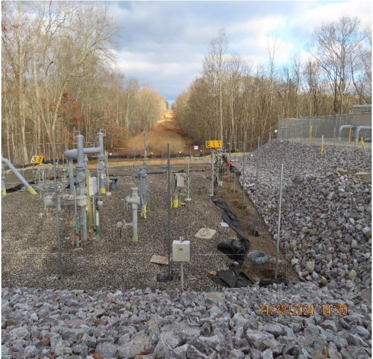
Photo 4: View (looking northeast) of valve yard with remaining security fence installation work in progress.
