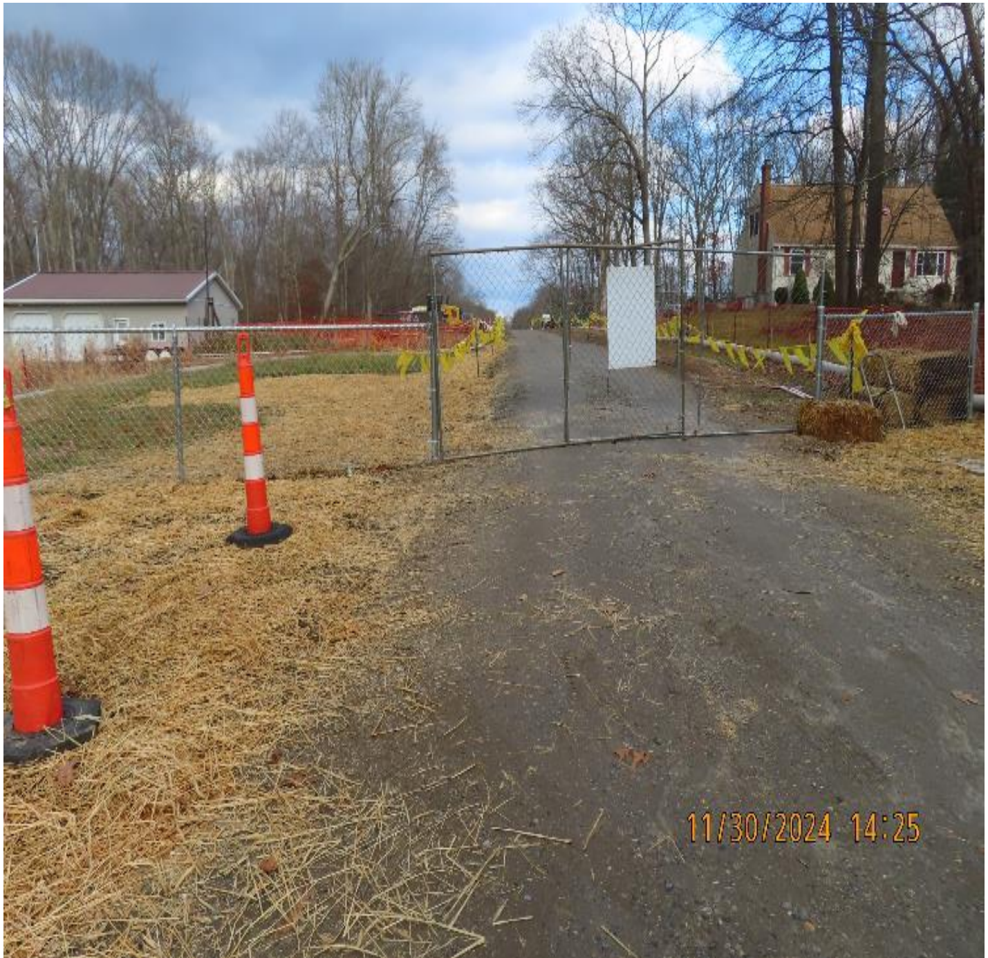
Photo 1: View (looking northeast) of site access entrance after mulch was placed along the edges.
