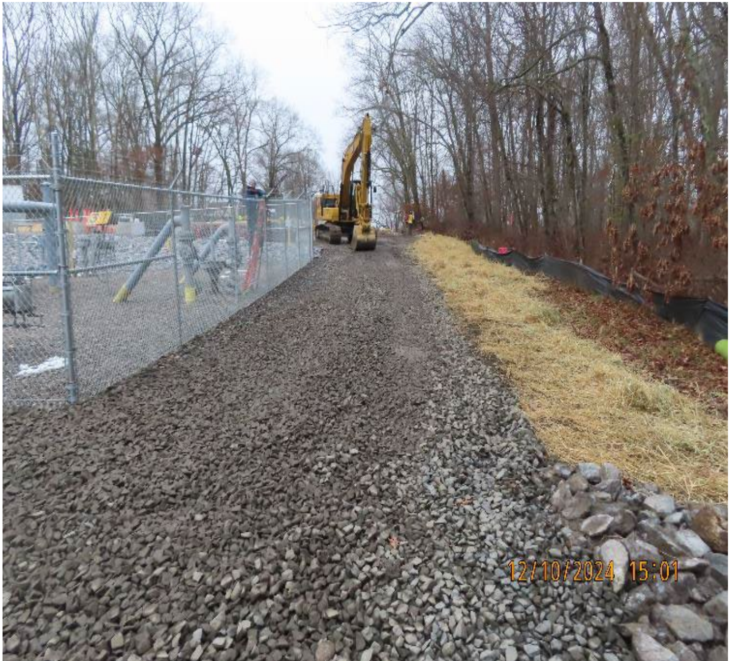
Photo 7: View (looking southwest) of new access travel lane along west side of the valve yard.
