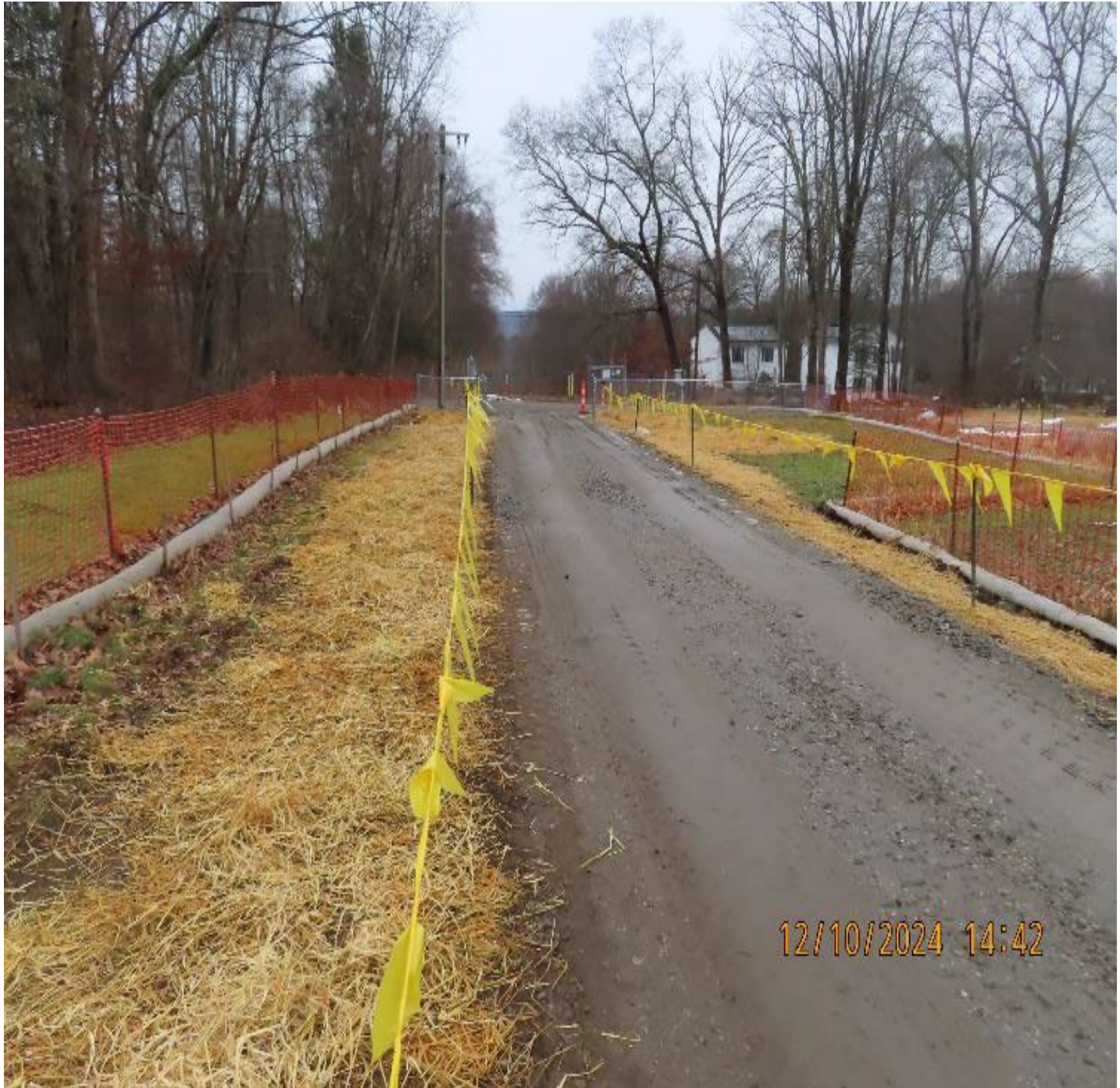
Photo 3: View (looking southwest) of access drive after winter stabilization. Compost filter sock and safety fence will remain until touch-up mechanical and final restoration work is completed in Spring of 2025.
