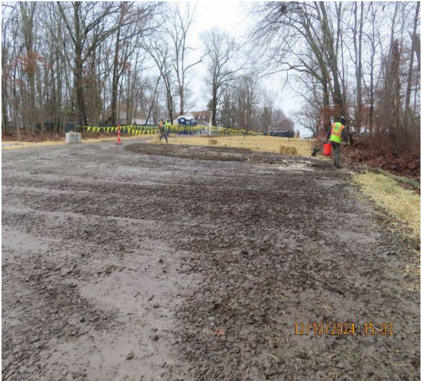
Photo 8: View (looking southwest) of seed and mulch application taking place southwest of the valve yard.
