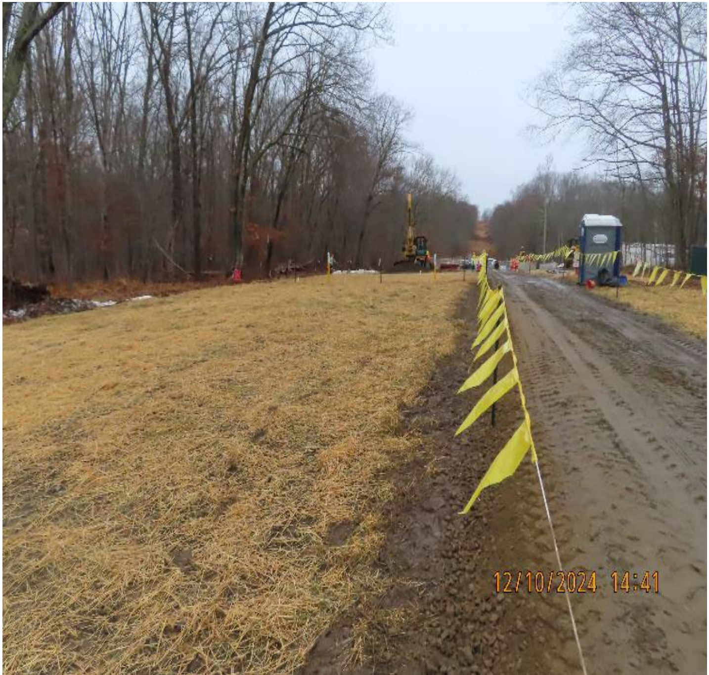
Photo 2: View (looking northeast) of former staging area after application of winter stabilization measures.
