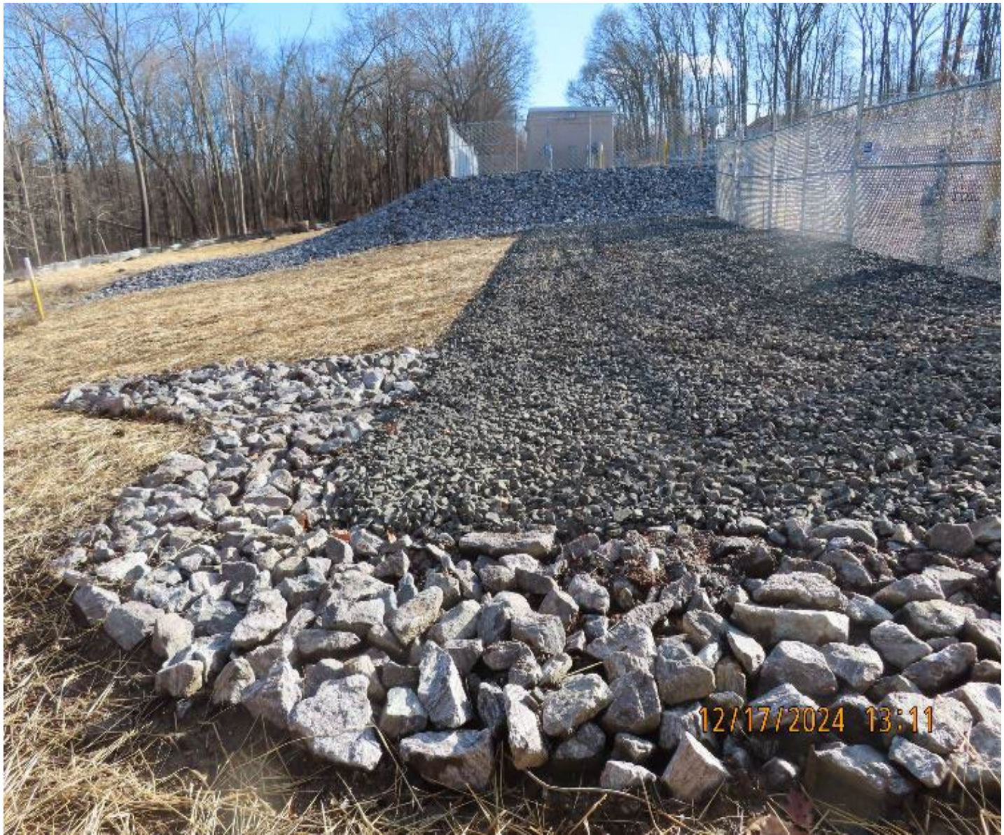
Photo 7: View (looking east) along north side of the valve yard.
