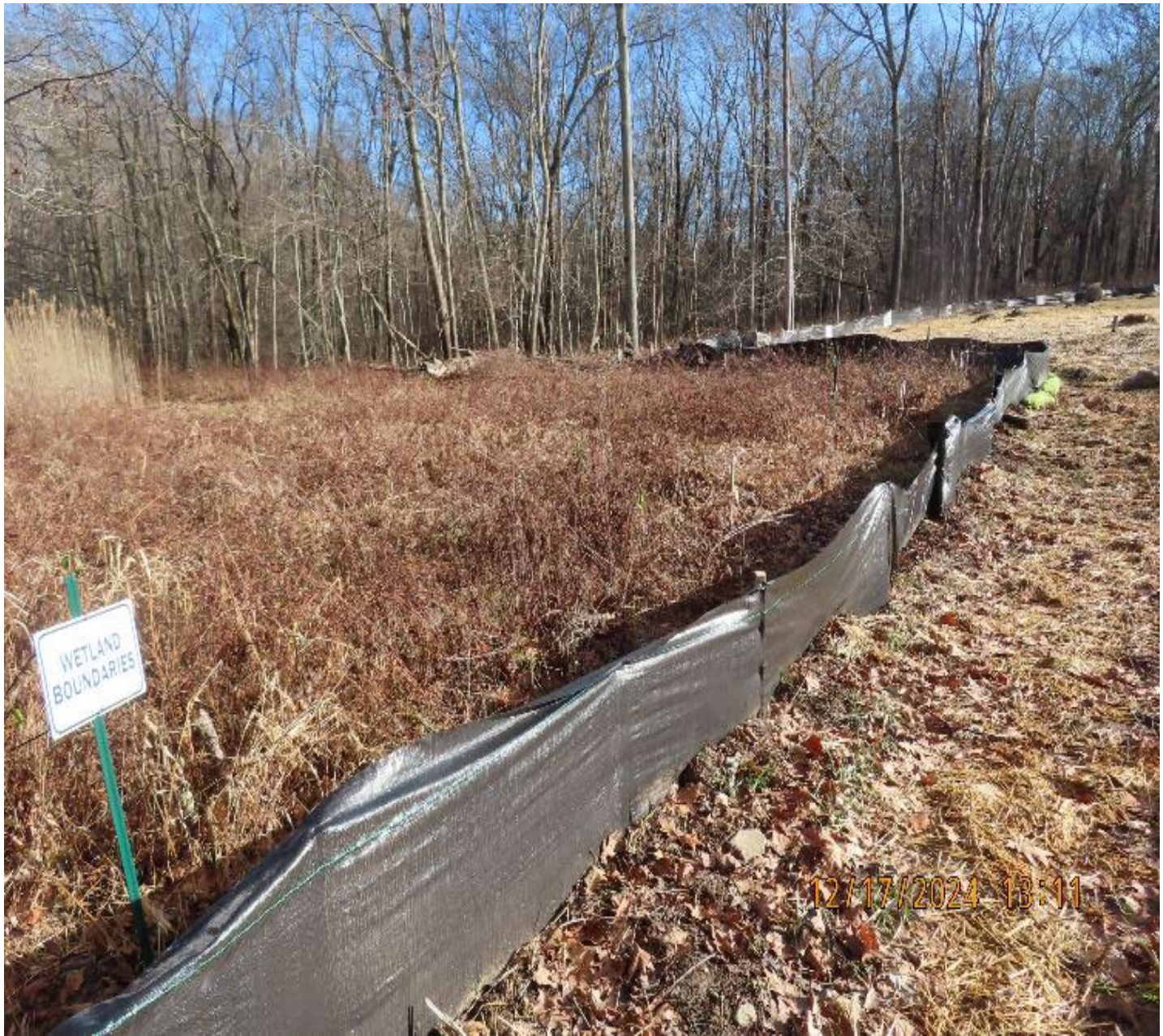
Photo 8: View (looking northeast) of silt fence between restored workspace and wetland W-CZ-01.
