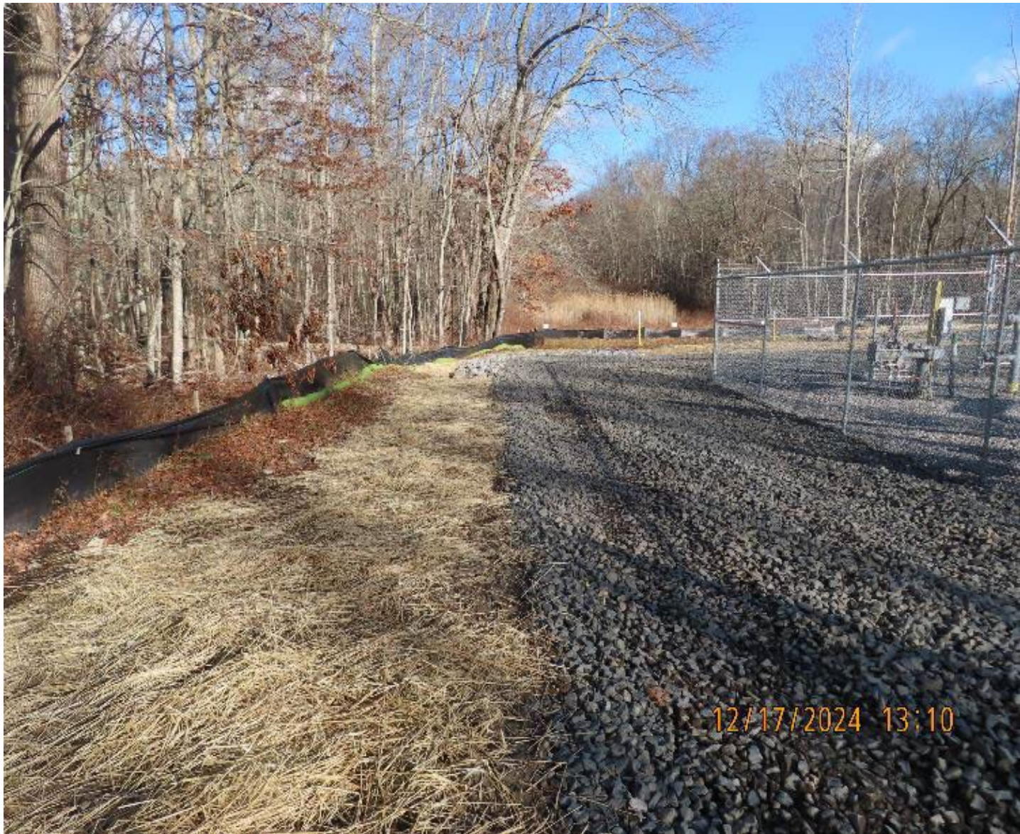
Photo 6: View (looking northeast) of rock travel lane constructed along west side of the valve yard.
