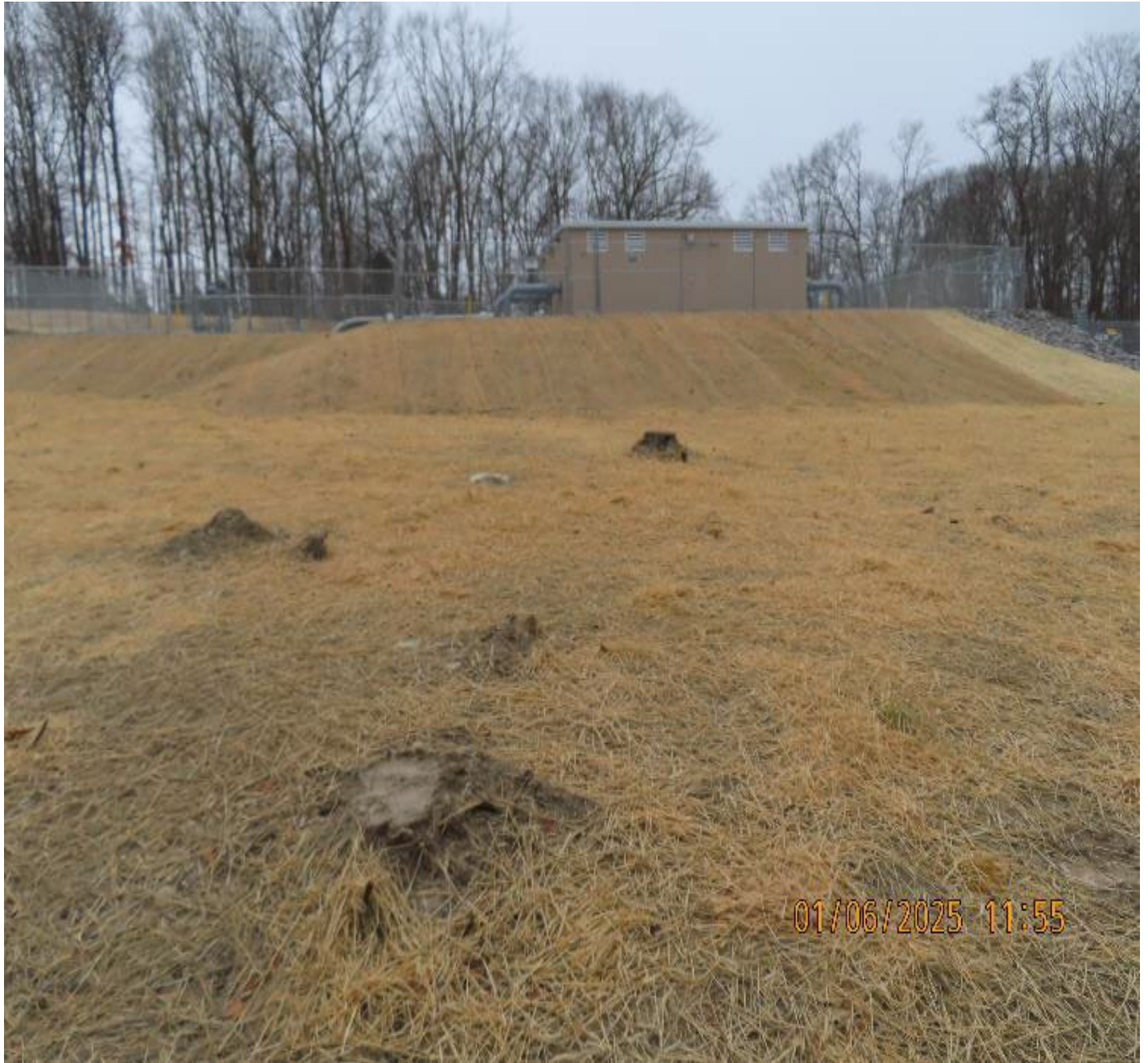
Photo 6: View (looking southwest) of former workspace and embankment downslope of the new regulator building.
