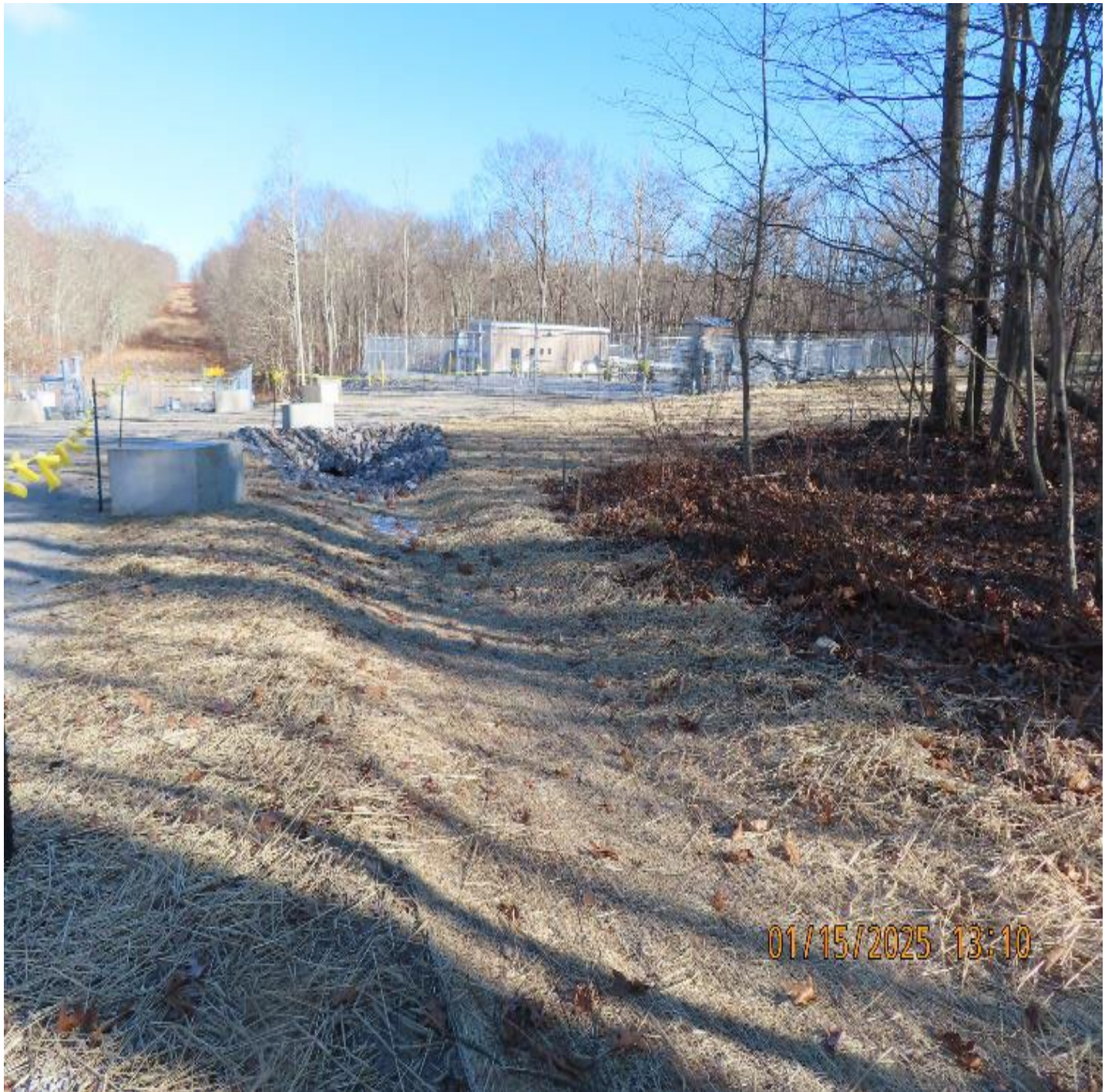
Photo 3: View (looking northeast) of restored drainage swale to culvert below access road into valve yard.
