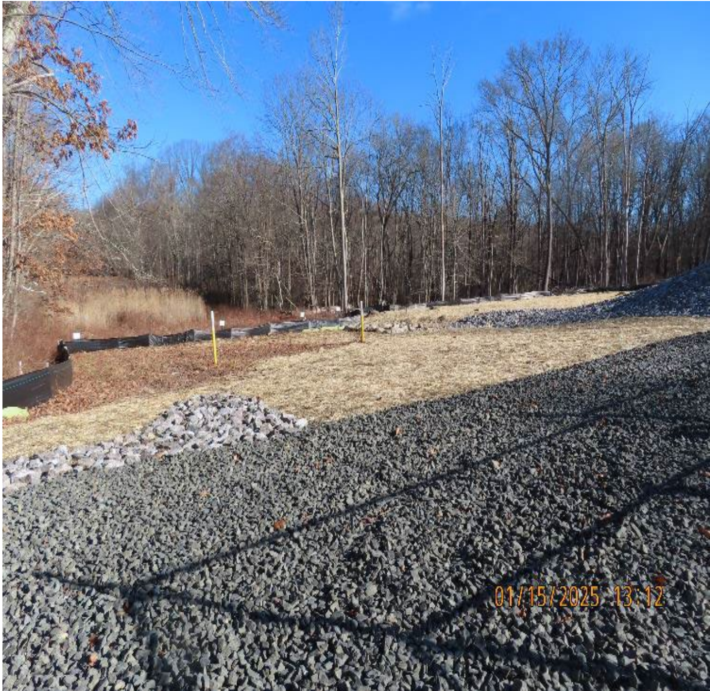
Photo 6: View (looking northeast) of new stone surfacing for access to the north gate of the valve yard.
