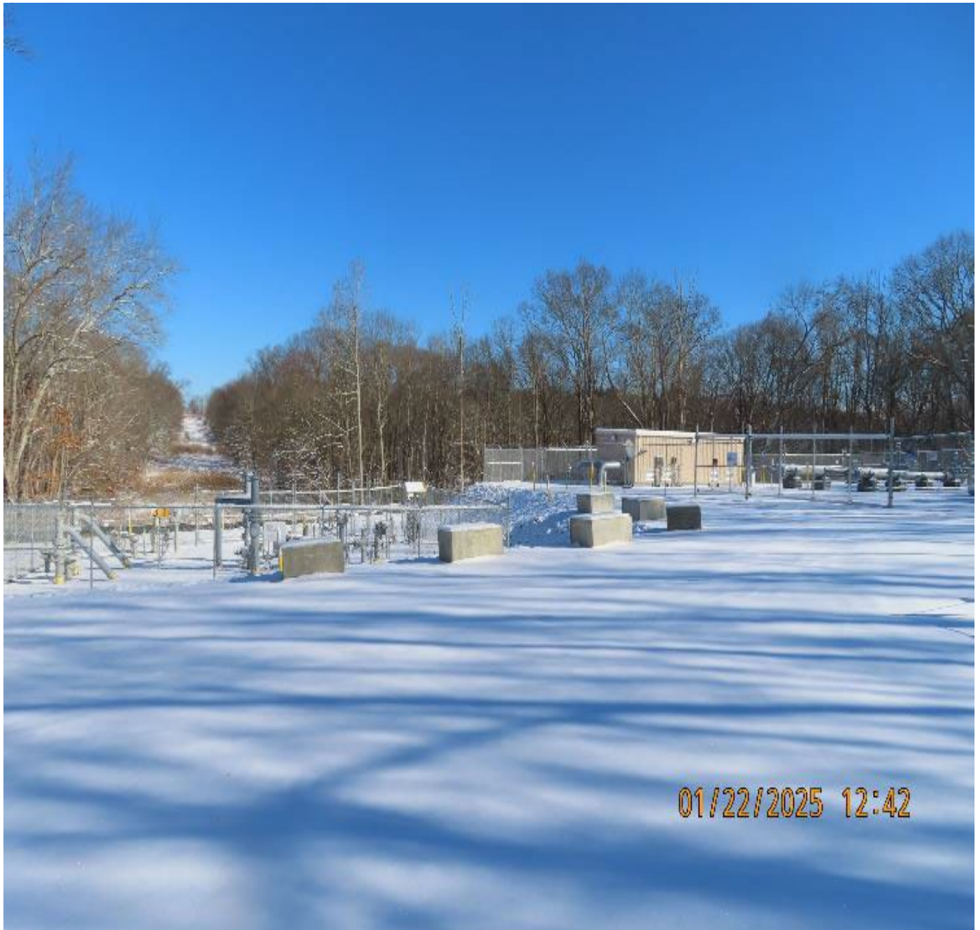
Photo 4: View (looking northeast) of valve yard.
