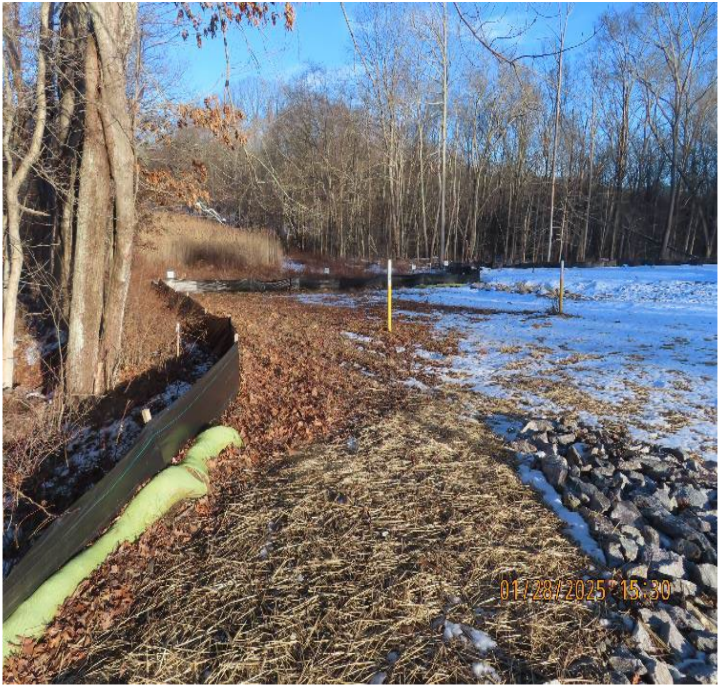
Photo 5: View (looking northeast) of erosion controls along northwest corner of former workspace.
