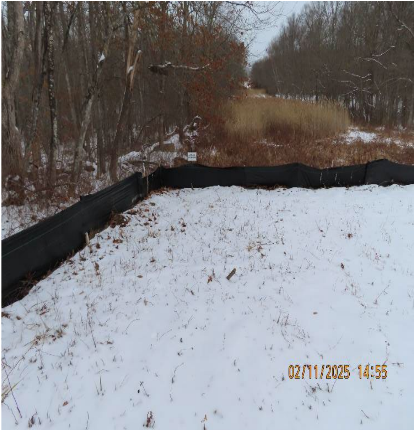
Photo 4: View (looking northeast) of silt fence along Wetland W-CZ-01 at northwest corner of workspace.
