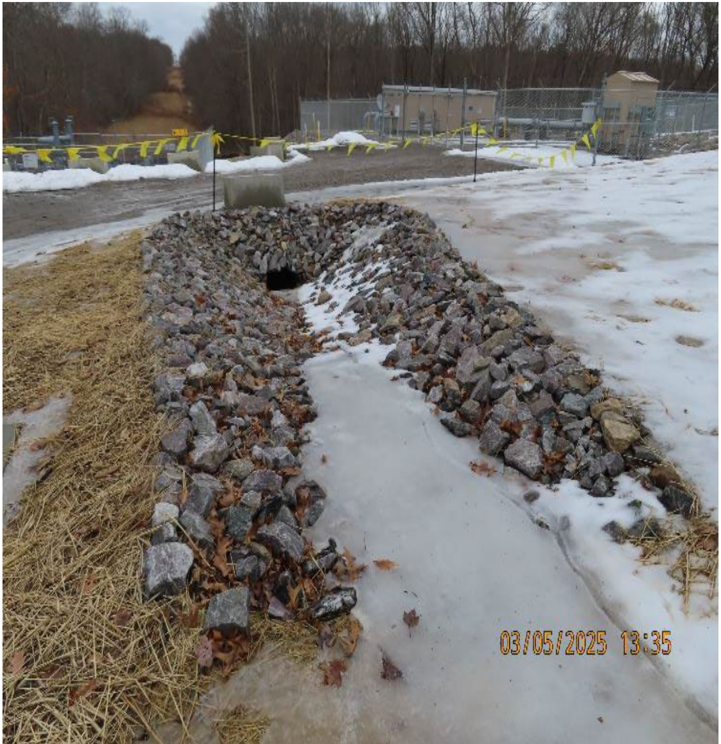
Photo 3: View (looking northeast) of drainage swale and culvert under entrance to the valve yard.
