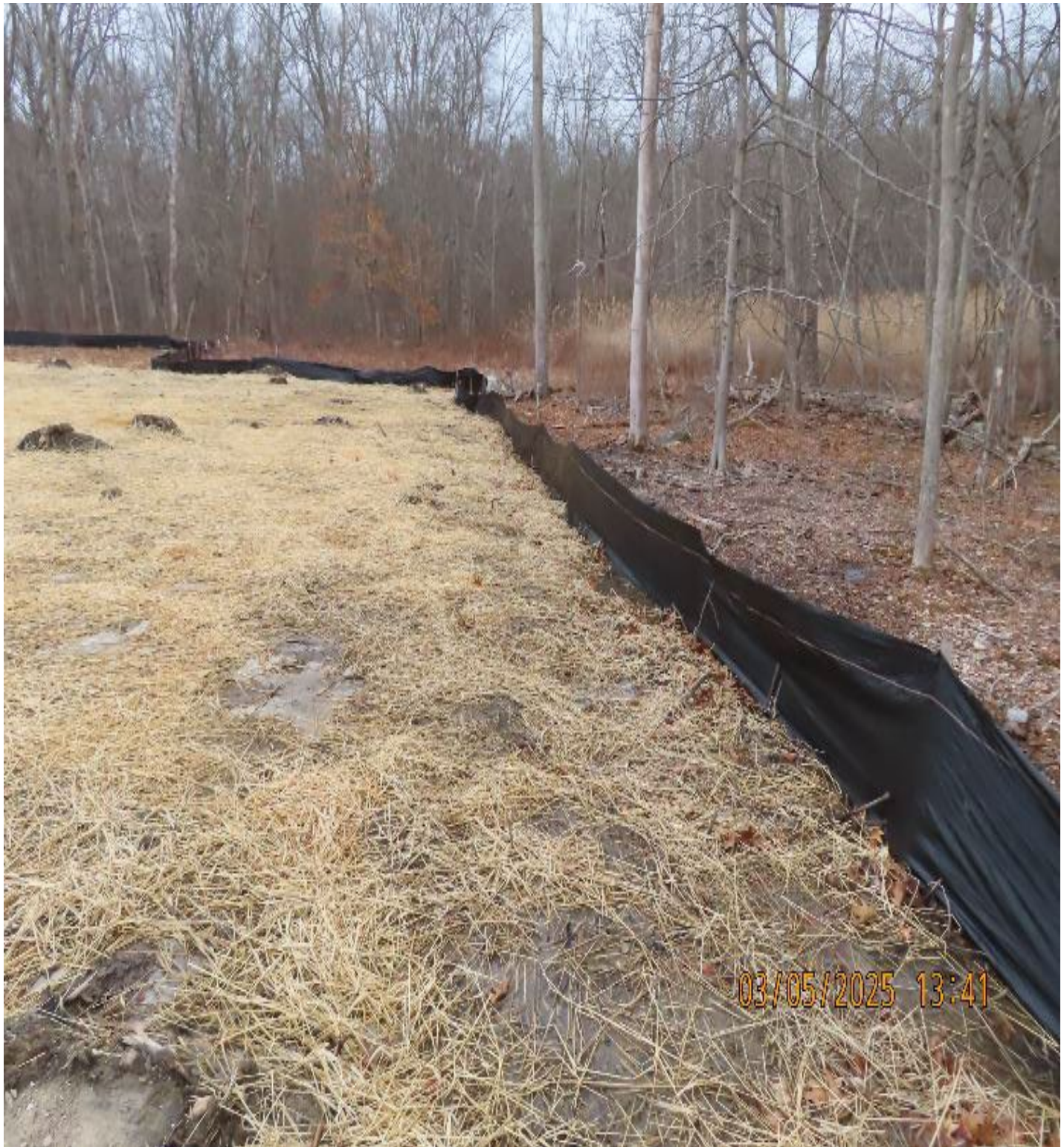
Photo 6: View (looking northwest) of perimeter silt fence along downslope side of former workspace.
