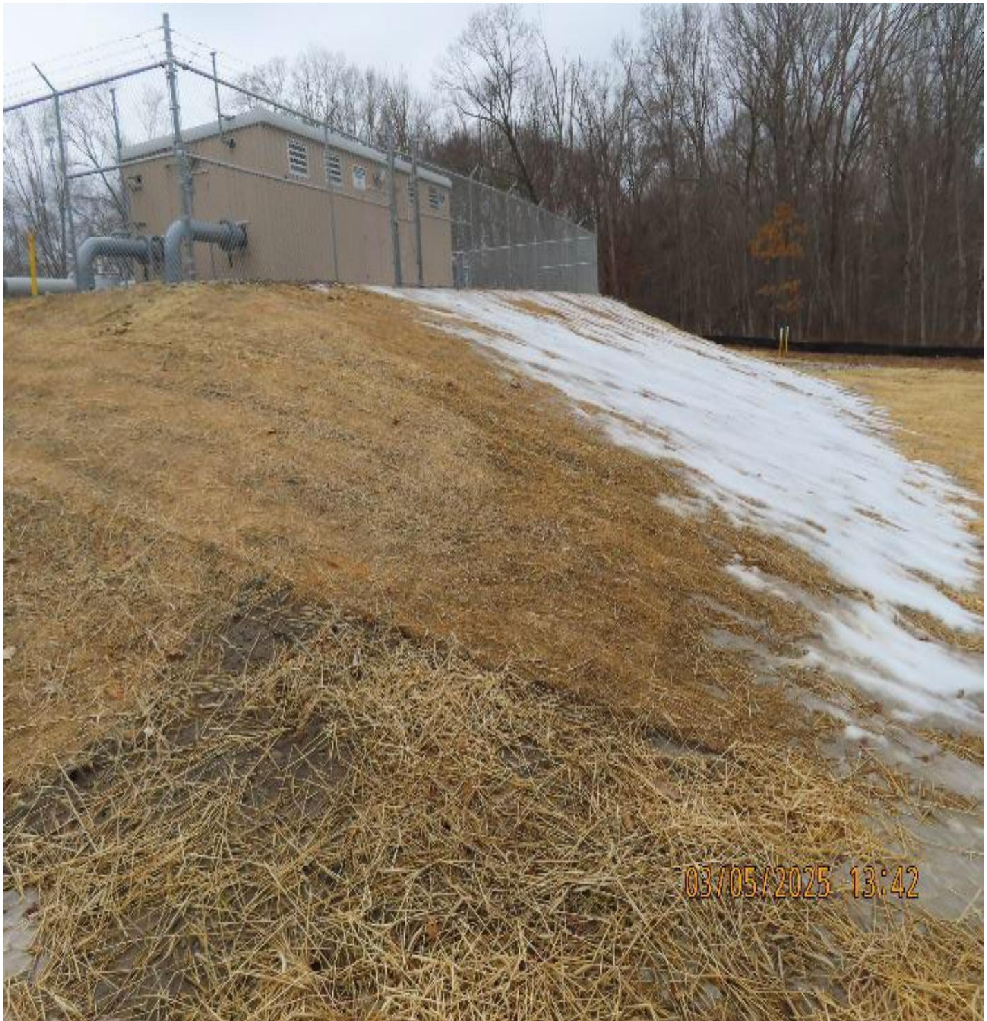
Photo 4: View (looking west) at restored slope north of the new regulator building.
