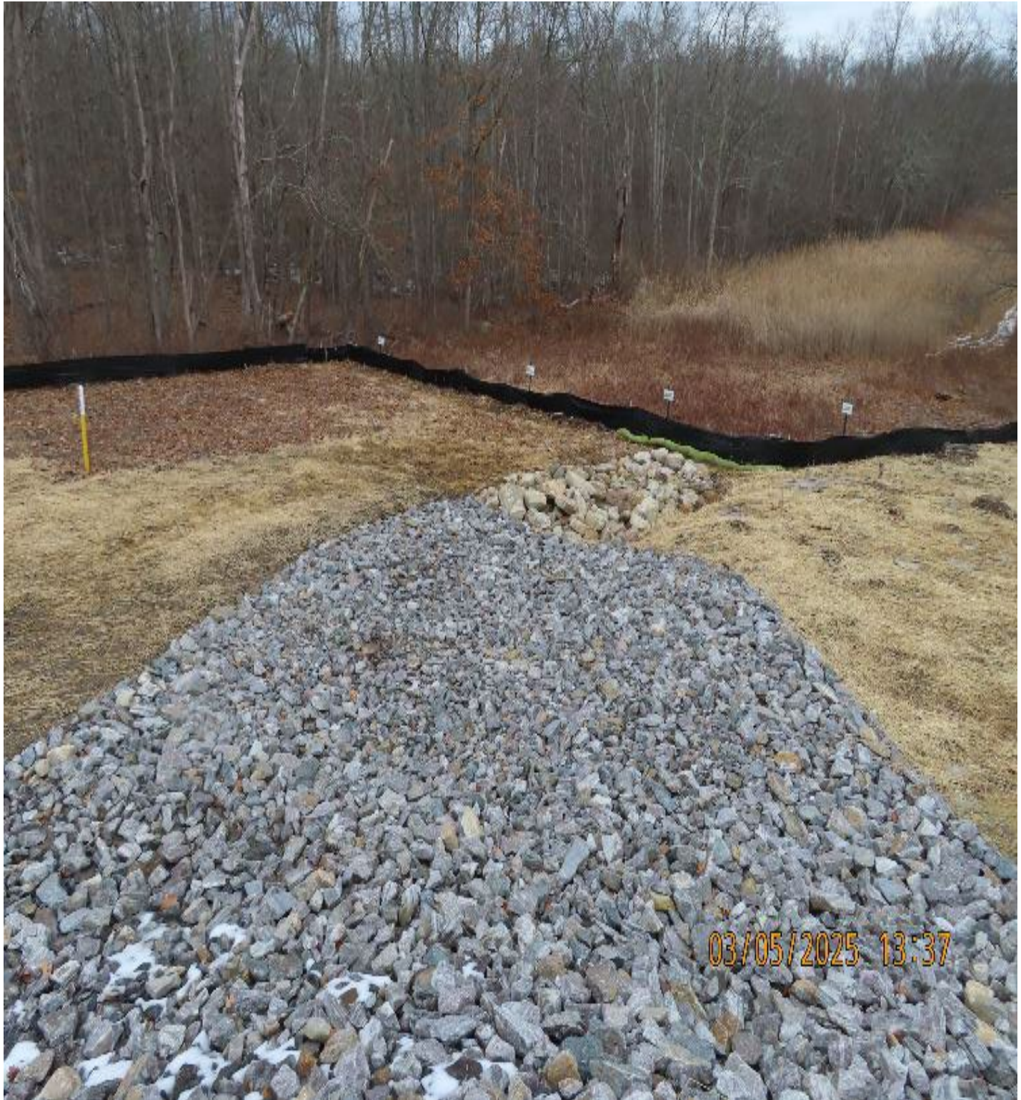
Photo 5: View (looking north) of drainage swale and perimeter silt fence at northwest corner of former workspace.
