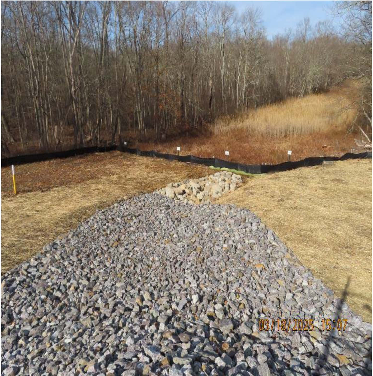
Photo 6: View (looking north) of rip-rap and rock armored drainage swale downslope from northwest corner of the new regulator building.
