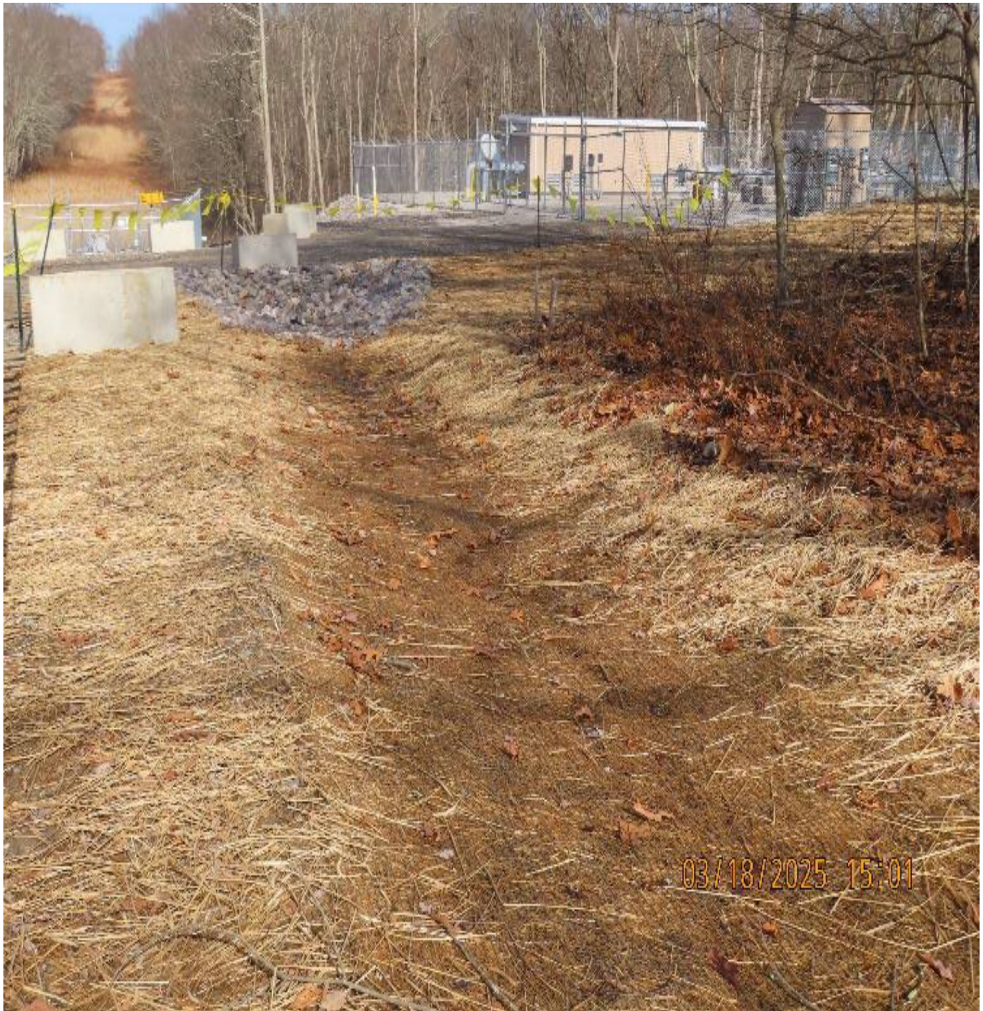
Photo 3: View (looking northeast) of drainage swale leading to culverted entrance into the valve yard.
